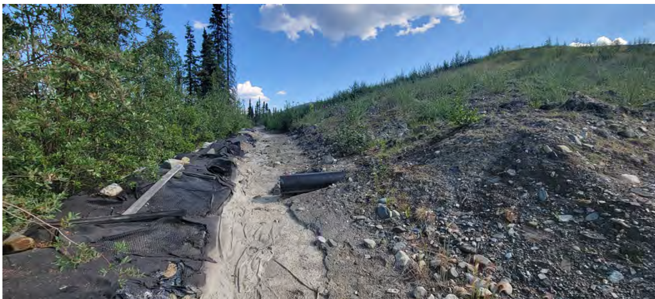
Photo 18: DSTF Phase 1 south west runoff collection ditching, Facing North. Typical, showing exposed an unanchored liner and buildup of sediment. (I. MacIntyre, July 20, 2023)
