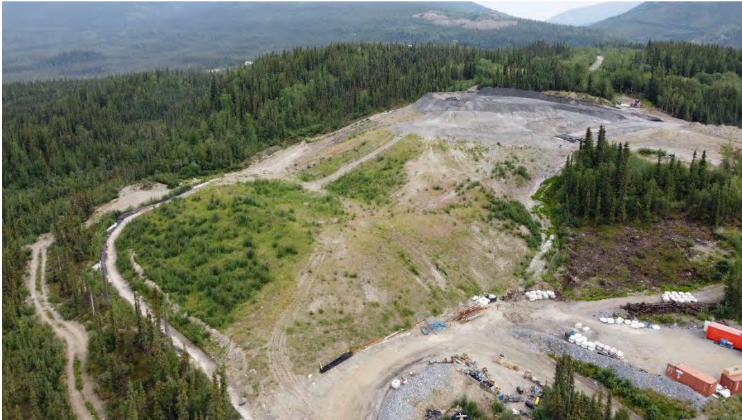
Photo 13: DSTF Phase 1 – aerial view facing northeast. Areas of erosion visible in foreground slope. (I. MacIntyre, July 22, 2023)
