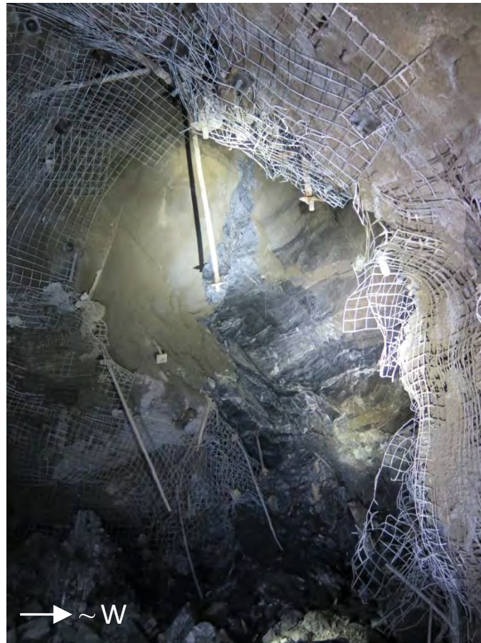
Figure 9. Photograph of the fall of ground on 1110L at the intersection with the first ore lens.
