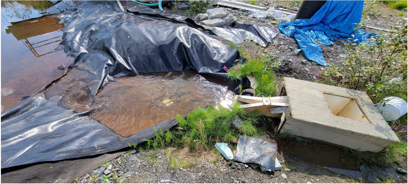
Photo 5: Bellekeno 625 Water Treatment Ponds, outlet structure. Note unsupported liner and flume. (I. MacIntyre, July 20, 2023)
