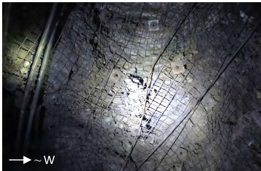
Figure 2. Photograph of the south shoulder of the Main Ramp towards the portal, showing weak ravelling material accumulating in the screen.
