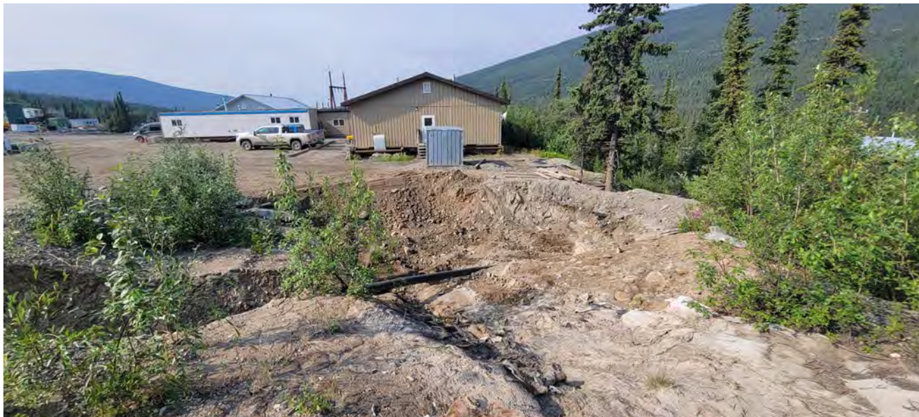
Photo 17: DSTF Phase 1 collection sump after cleaning of sediment build up. Liner was later installed. Facing southwest. (I. MacIntyre, July 22, 2023)
