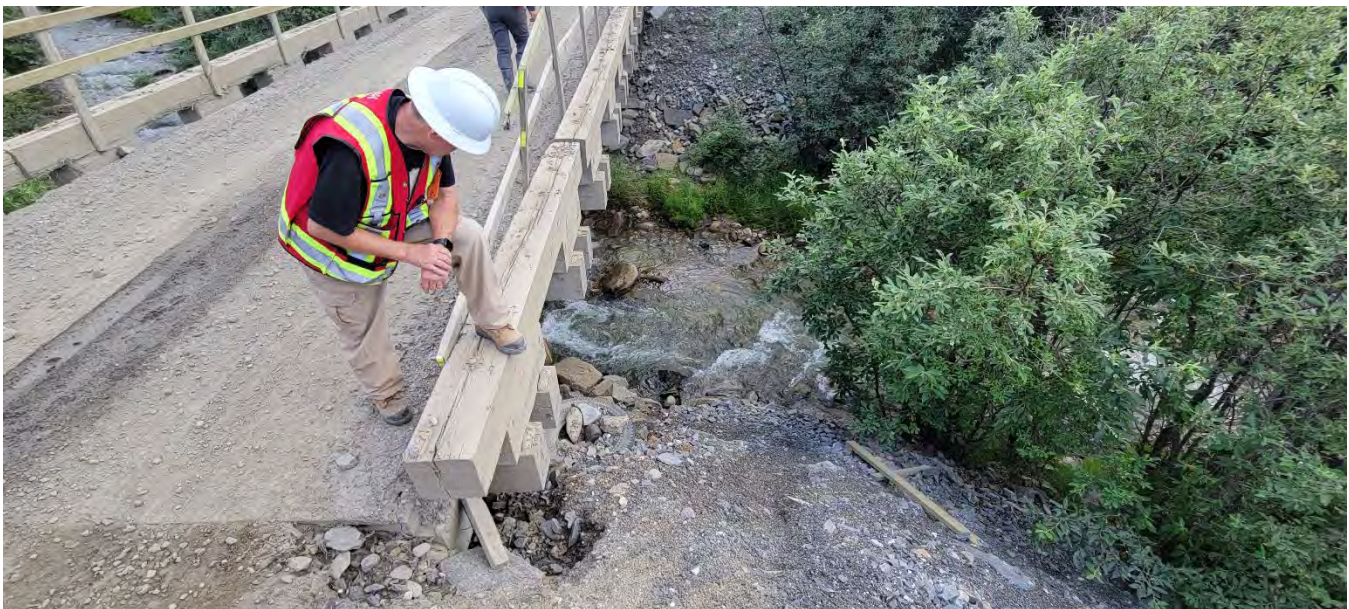
Photo 7: Lightning Creek Bridge – Bellekeno Haul Road, erosion along abutment (I. MacIntyre, July 20, 2023)
