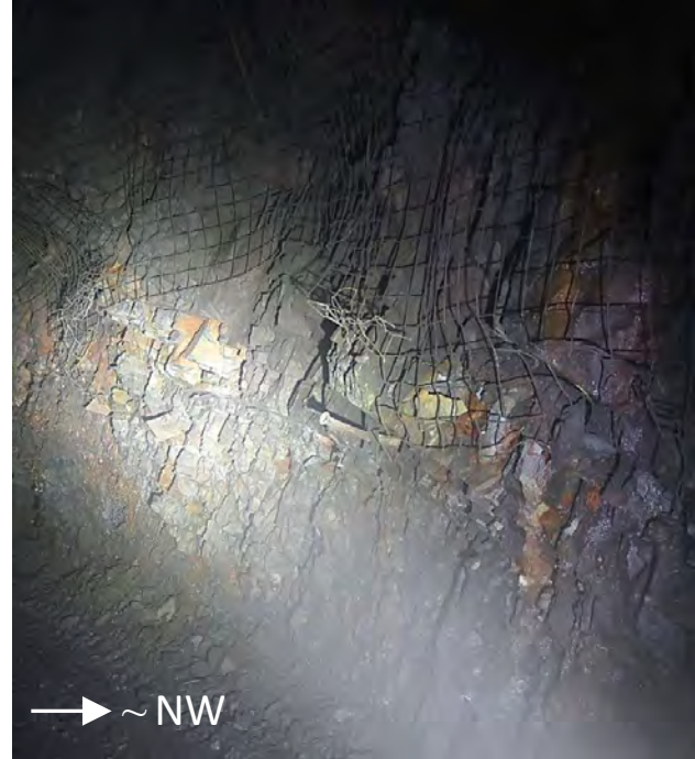
Figure 13. Photograph of the west wall of the Main Ramp showing damage below the ground support. At least a foot of wall has been lost.
