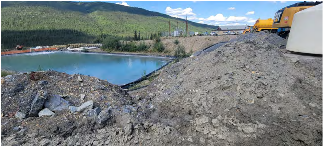
Photo 11: Fill Water Storage pond, erosion gully – facing northeast (I. MacIntyre, July 20, 2023)
