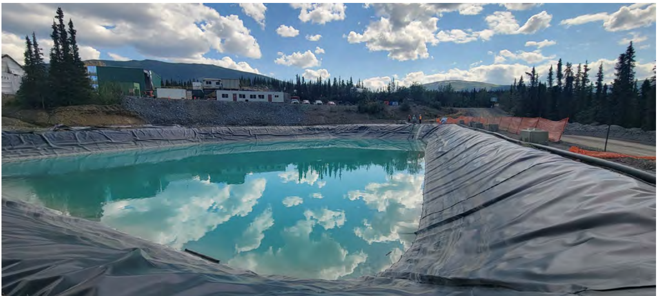
Photo 12: Mill water storage pond, erosion gully – facing south (I. MacIntyre, July 20, 2023)
