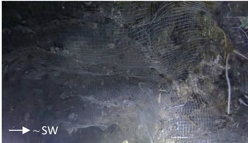
Figure 3. Photograph of the roof of the Main Ramp in a sector with persistent structures that delineate larger blocks / wedges.
