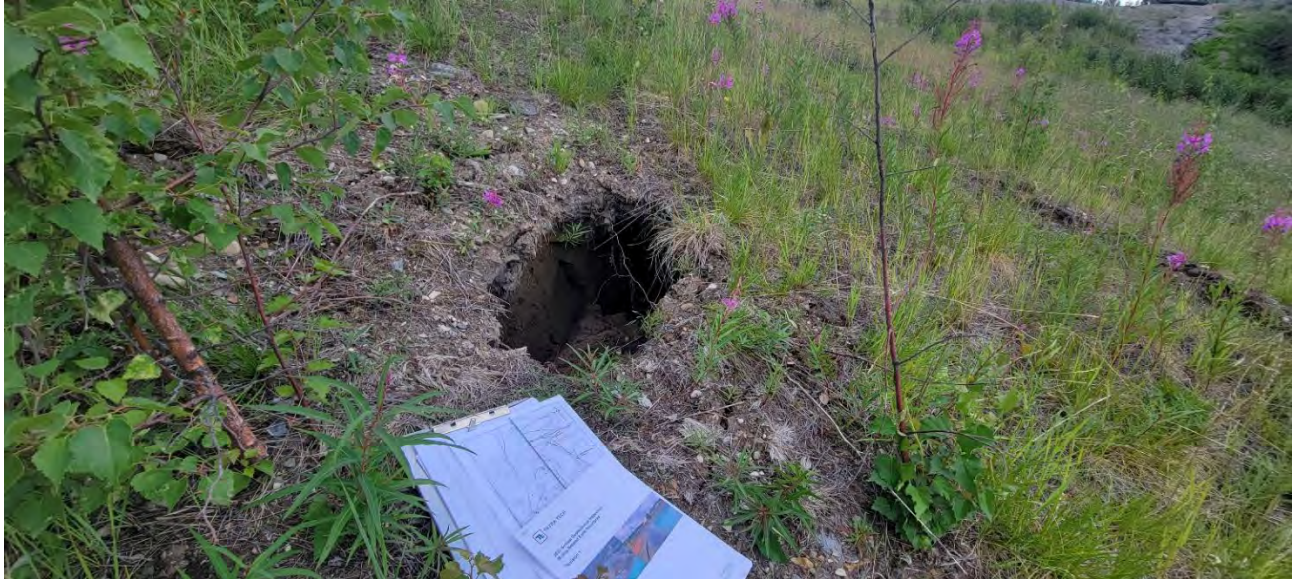
Photo 16: DSTF Phase 1A area, southwest slope. Small sink hole indicating migration of materials. Extends below cover into tailings. Erosion gully visible in background (I. MacIntyre, July 20, 2023)
