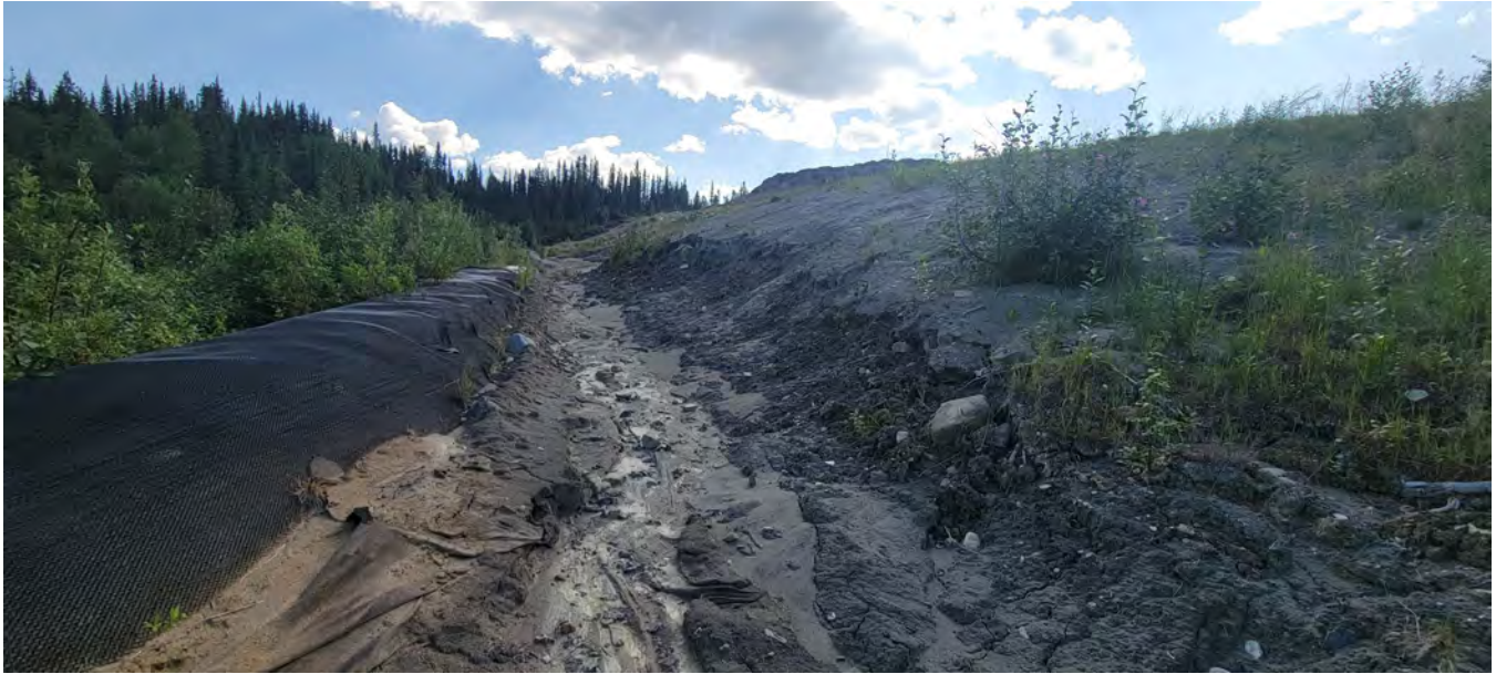
Photo 19: DSTF Phase 1 north perimeter runoff collection ditching, Facing North. Typical, showing exposed an unanchored liner and buildup of sediment. (I. MacIntyre, July 22, 2023)
