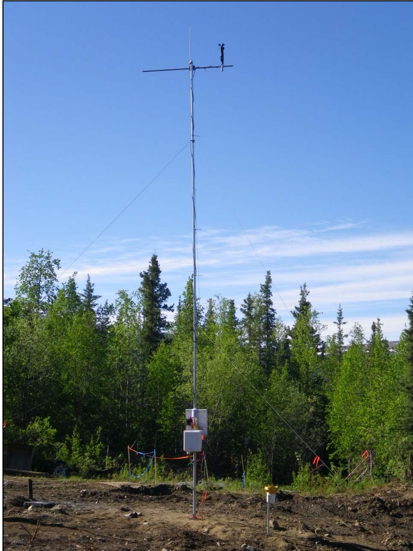
District Mill Campbell Scientific Meteorological Station
