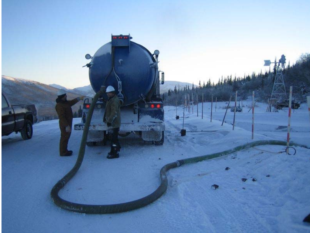
FIGURE 4 – VACUUM TRUCK USED TO DESLUDGING PONDS
