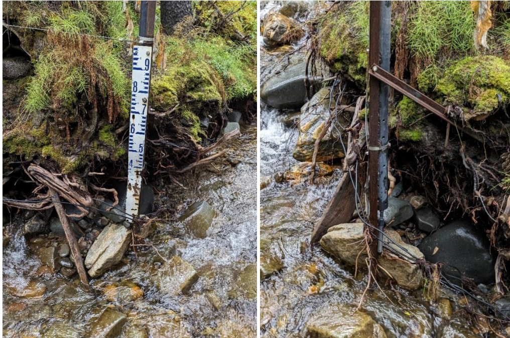
Figure 1 Damaged staff gauge and improperly installed data logger at Monitoring Station KV-64.
