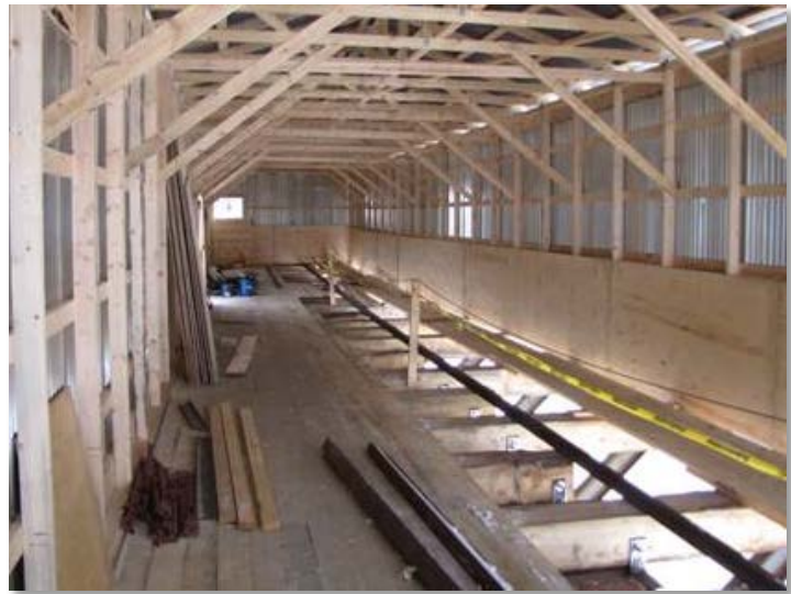
Figure 2. Lucky Queen trestle area at portal pad for 7 t mine trucks to dump their load. (Image from proponent)
