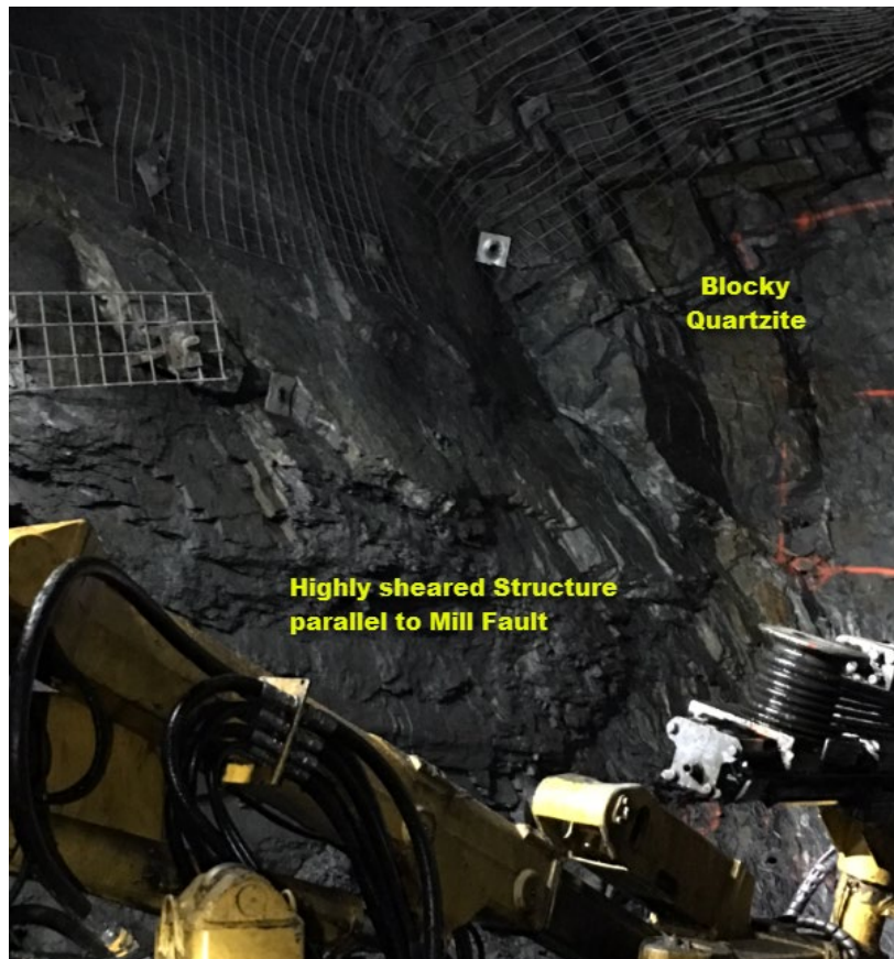
Figure 4.3 Ground condition of first remuck drift in main decline ramp from Flame and Moth
