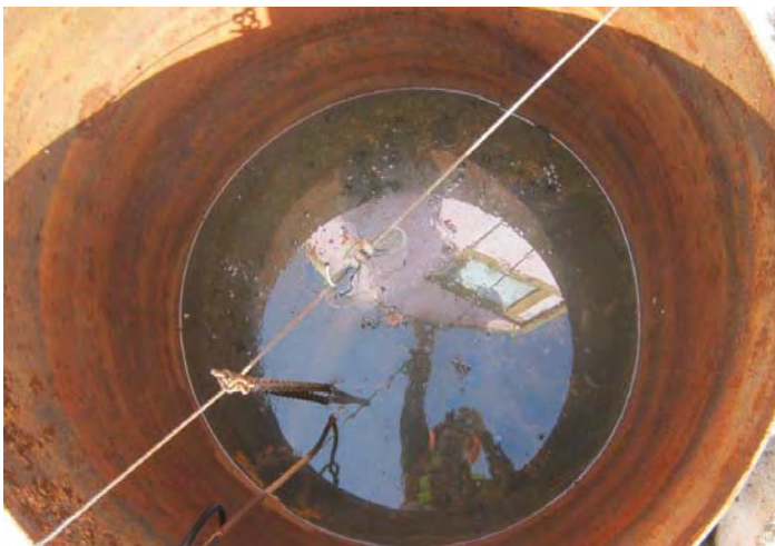
Figure 3 - Bioreactor Influent Sump
