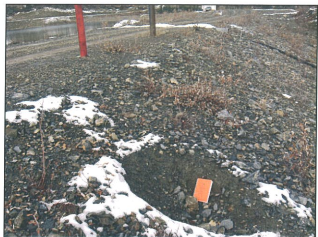
Figure 19 Sinkhole in South Dam
