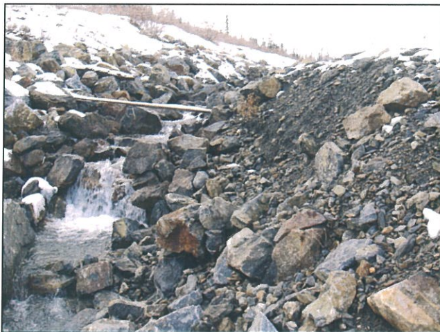
Figure 22 Ravelling of Riprapped Bank
