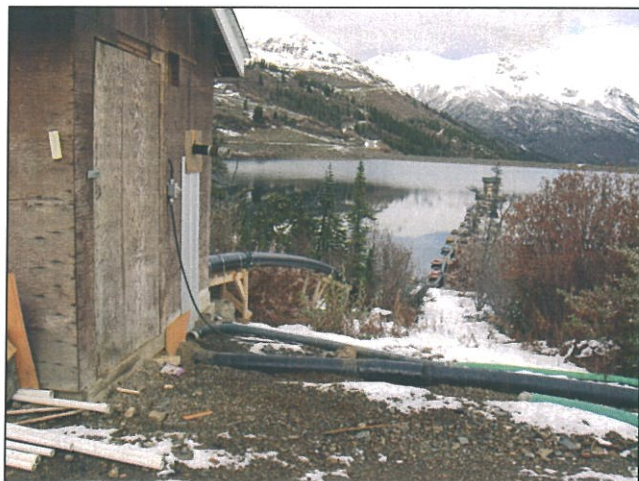
Figure 06 Pumphouse, Intake and Discharge Lines
