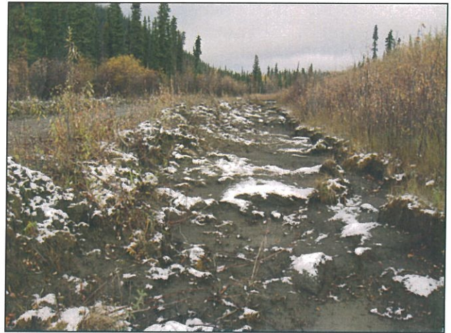
Figure 45 Drainage Channel at Location H
