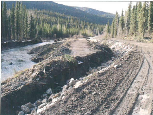
Figure 32 Road Washout at Location B
