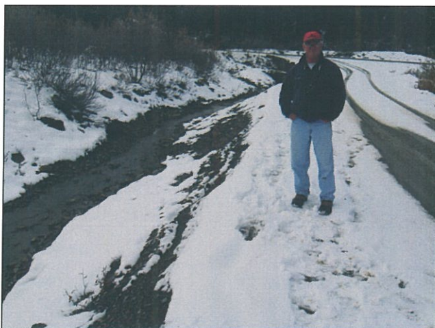
Figure 26 Minor Bank Slumping
