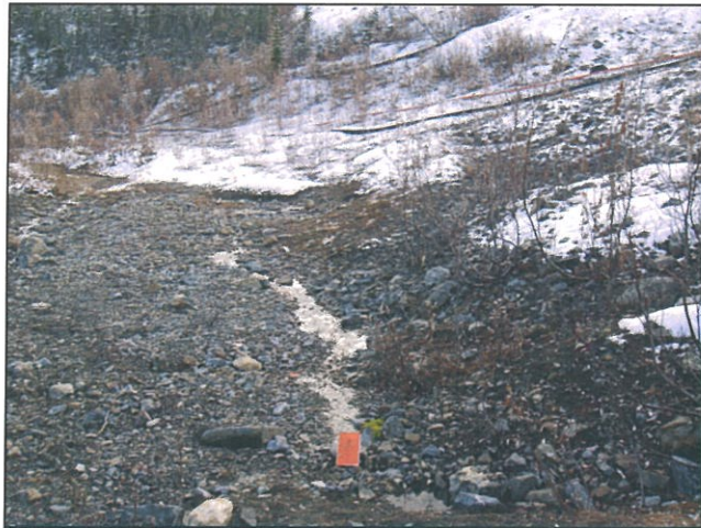
Figure 16 Seepage at Toe of North Dam
