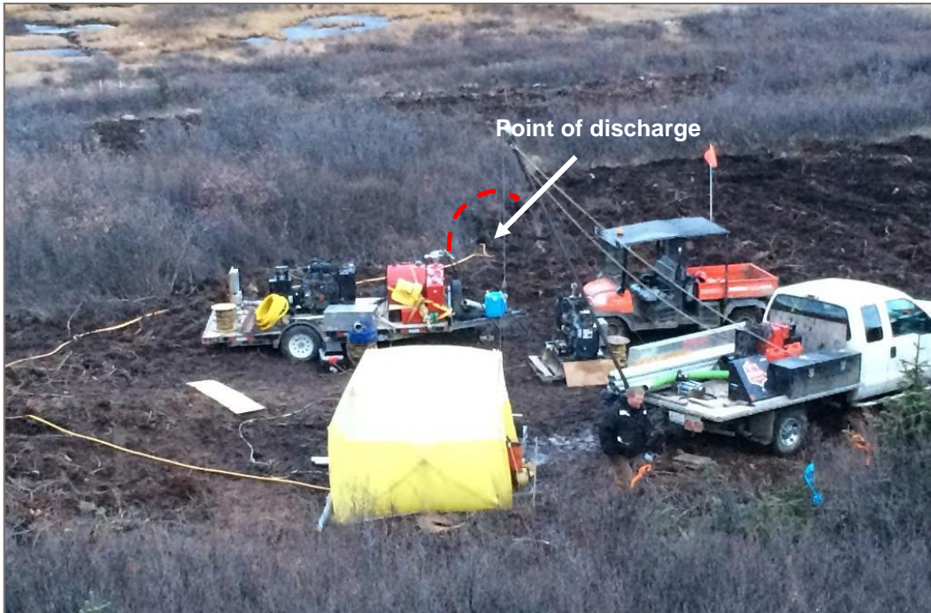
Photo 5: WW15-02 (view east) Pumping test setup, nearest surface waterbody (creek on the valley floor) is visible at the top of photograph. The red line shows the approximate extent of overland flow during water discharge.
