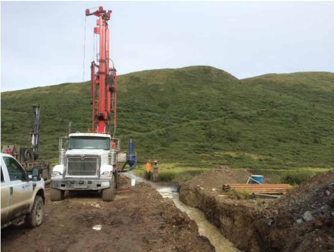
Figure A: Sump adjacent to WW15-01 used to store development water.
