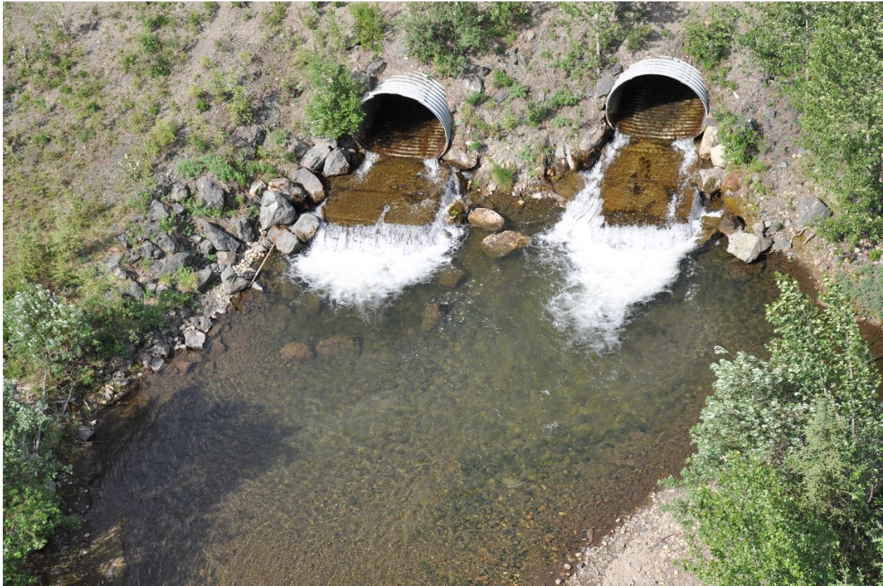
Plate 7-1: Downstream aerial view of Finlayson Creek Culverts at the Robert Campbell Highway June 17, 2016
