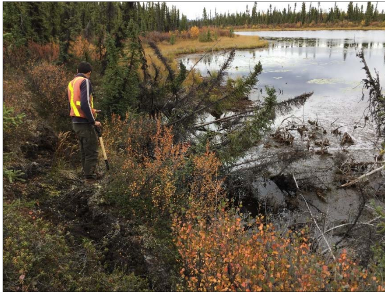
Photo 4-8. Leaning trees and collapsing bank indicative of thermokarst subsidence (-Xt) along shoreline of pond adjacent to access road near KM 5.5
