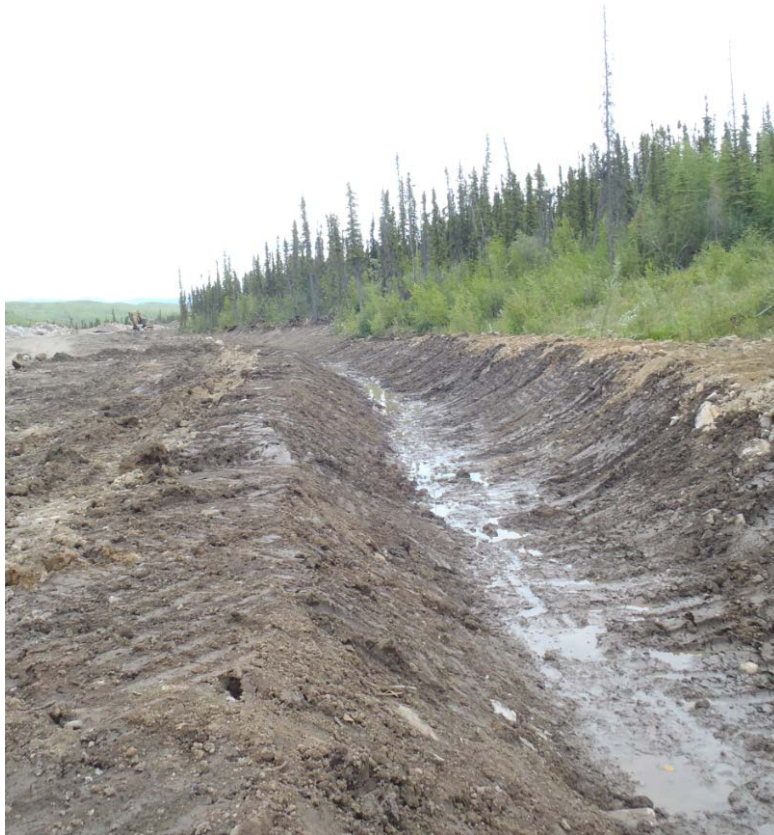
Figure 8: Section C Looking East with Overburden Placed On Top Of Geosynthetic Clay Liner
