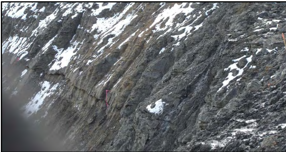
Figure 1-2: Movement along failure plane in overburden, south wall, Main pit, Stage 3 pushback, April 2009.
