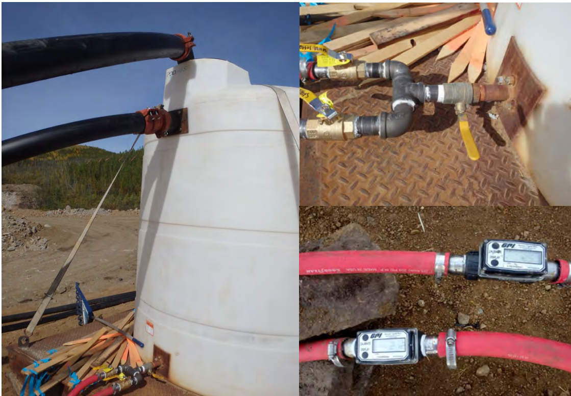
Figure 14. Clockwise from left: holding tank, splitting control valve, and flow meters.
