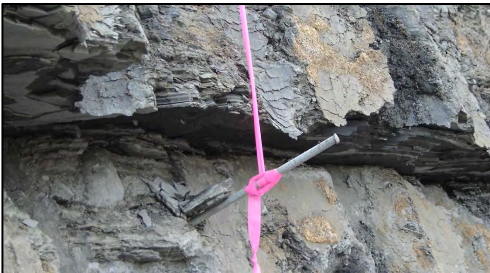
Figure 1-3: Displacement along the plane of movement: south wall, Main pit, Stage 3 pushback, April 2009.
