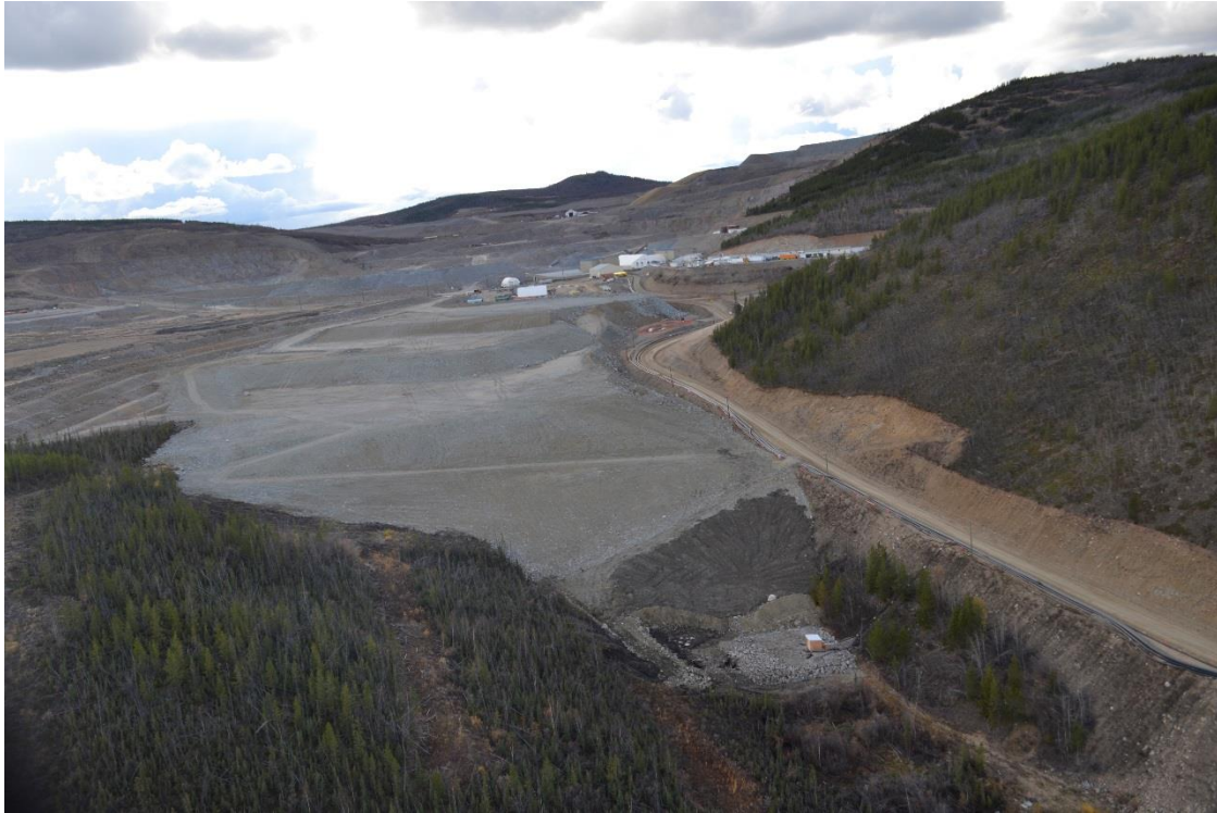
Figure 16-1: MVFES2 front face (looking west) recontoured at a maximum slope grade of 3:1.
