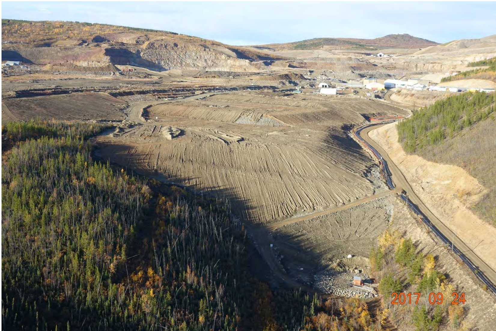
Figure 16-2: Minto Mine – Overburden cover pushed into place on the MVFE and DSTSF.
