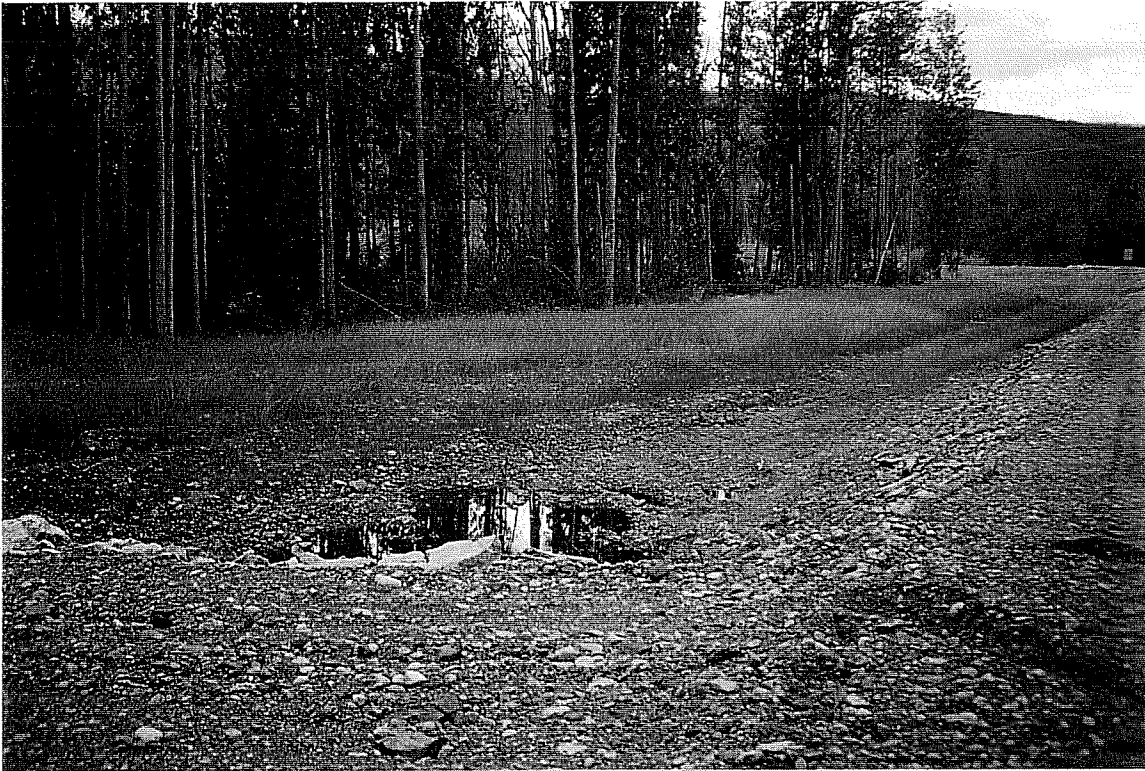
Photograph #6 – View of plant growth resulting from May 1999 seeding effort. South drainage ditch between ditch block #4 and #5. 05/September/1999
