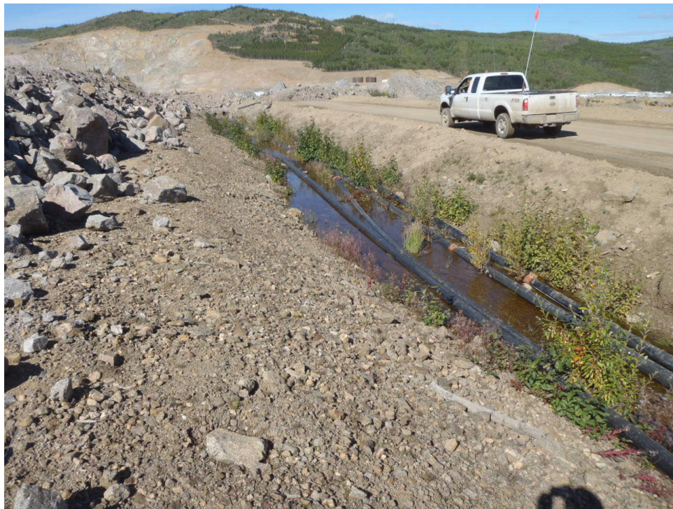
Photo 2 Area of settlement between STA 0+600 and STA 0+650. (August 25, 2011)
