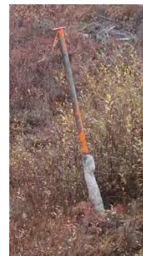
View of SWD-03A; leaning and heaved 75cm out of the ground.
