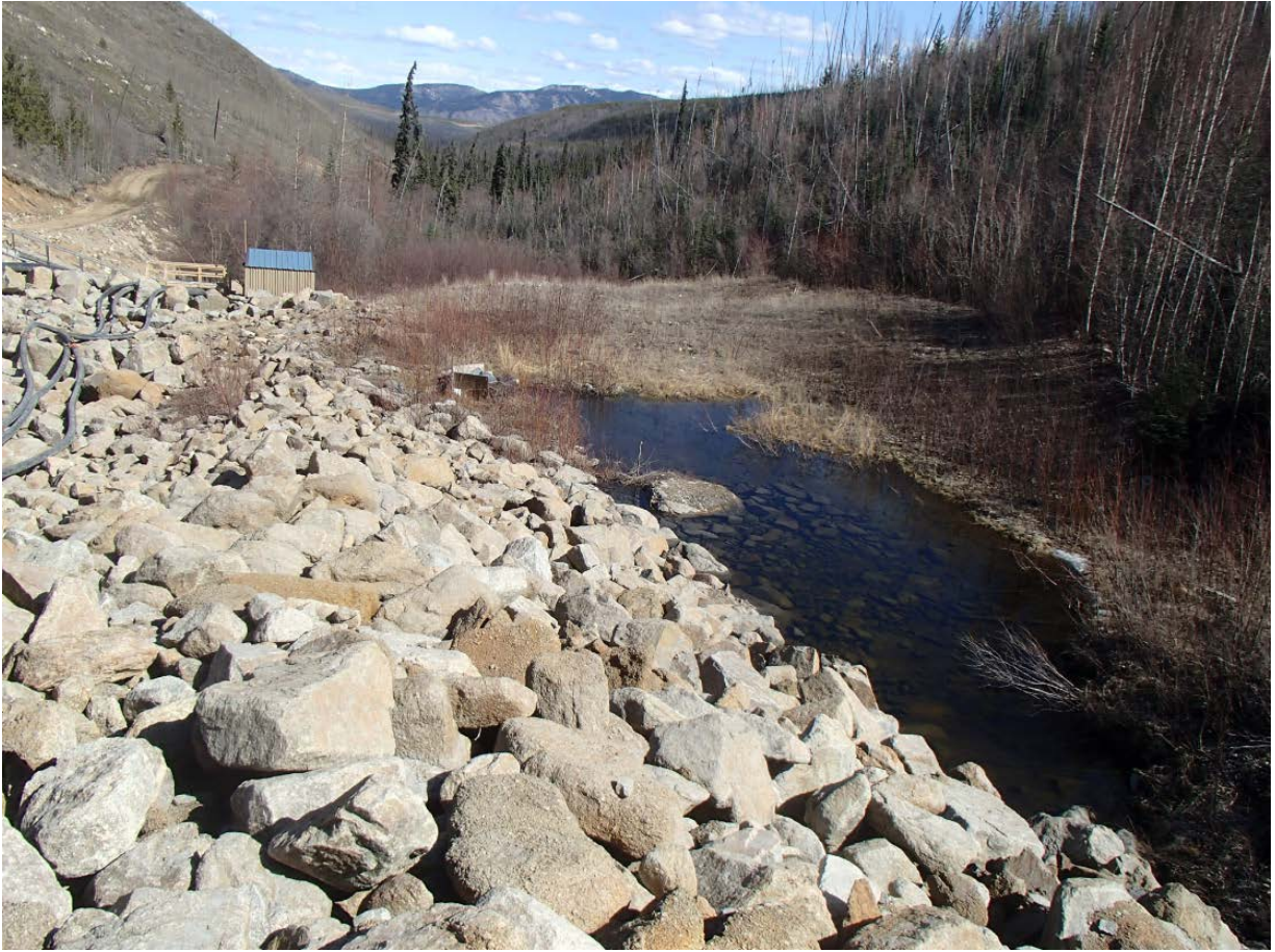
Figure 11: Water Storage Pond Dam - Ditching of the ponded water on the south abutment of the WSP Dam should be considered to ensure low groundwater pressures are maintained on the dam face
