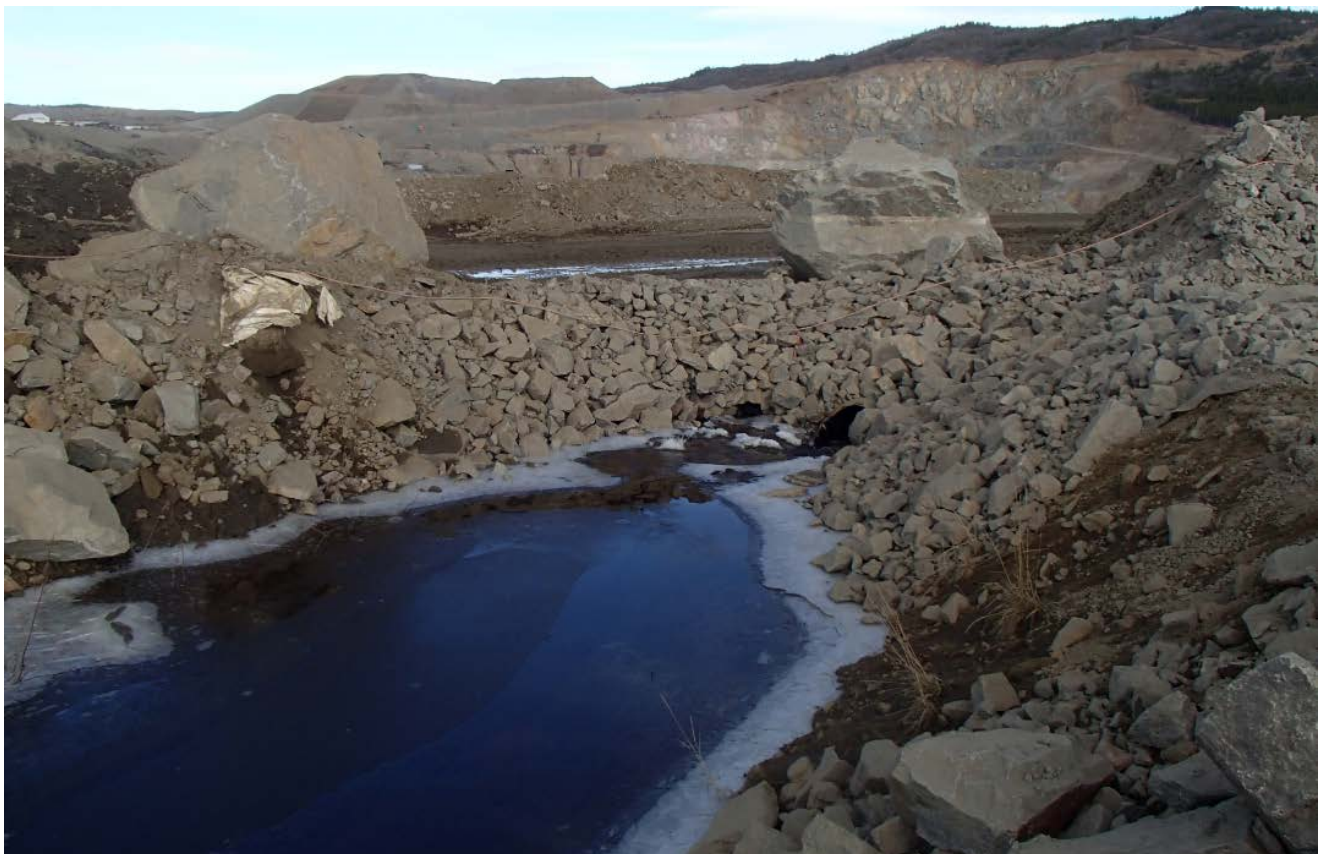
Figure 8: South Diversion Ditch - The swale for the South Diversion ditch should be completed as per SRK's South Diversion Ditch construction drawings, it is lacking width. The two boulders should also be removed.
