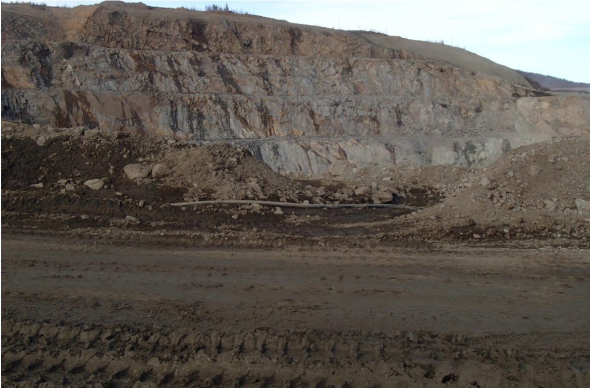
Figure 9: South Diversion Ditch, cont'd - The swale for the South Diversion ditch should be completed as per SRK's South Diversion Ditch construction design, it is lacking width, the downstream outlet for the swale is blocked
