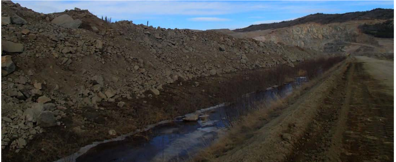
Figure 7: South Diversion Ditch - Should the South Diversion Ditch continue service, the deciduous vegetation should be cut back and removed.
