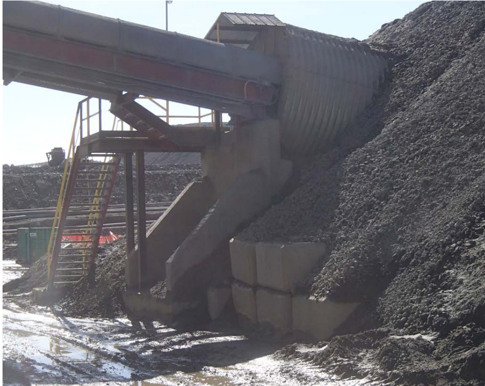
Figure 5: Mill - The retaining wall at the mill's apron feeder tunnel should be monitored, it is tilting forward in an active condition with the potential for overtopping.
