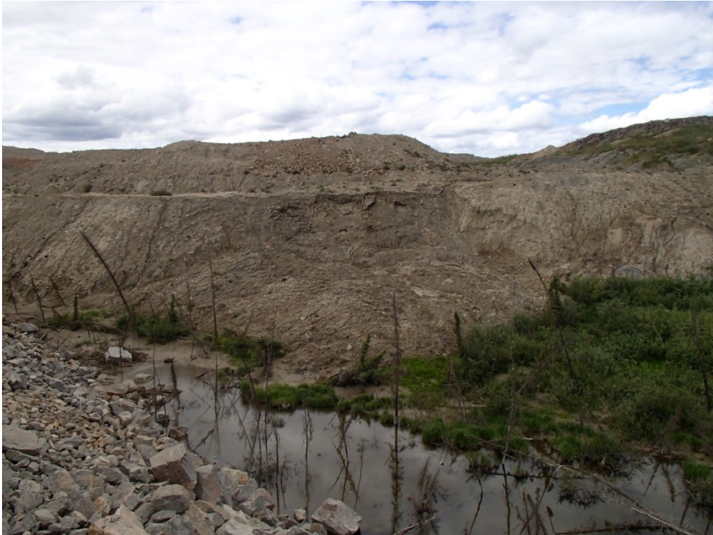
Figure 6: Reclamation Overburden Dump - Crest failure on southeast side of the ROD. Not a concern to large scale stability.
