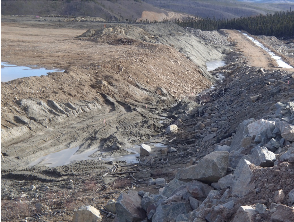
Figure 3: Dry Stack Tailings Storage Facility - South side of DSTSF at East end.
