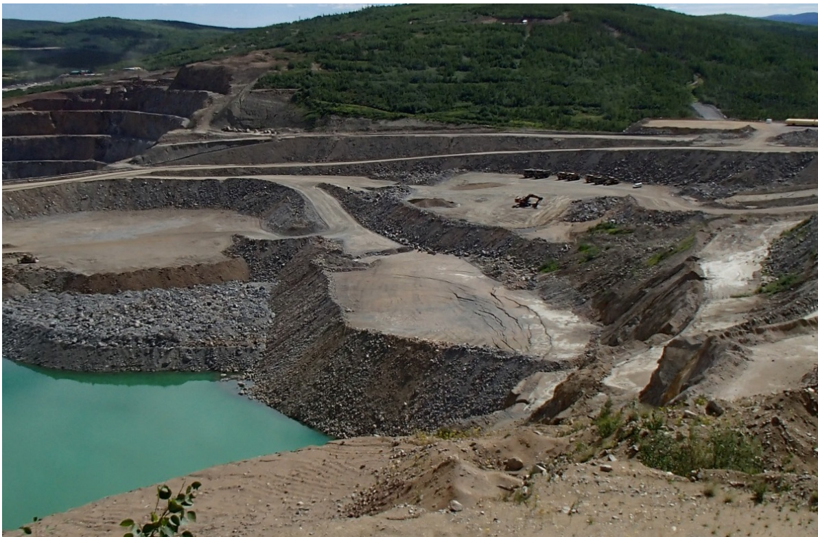
Figure 10: Main Pit South Wall Buttress – Tension cracks appear to have increased/dilated from the previous inspection. Install prisms along crest to monitor movement.
