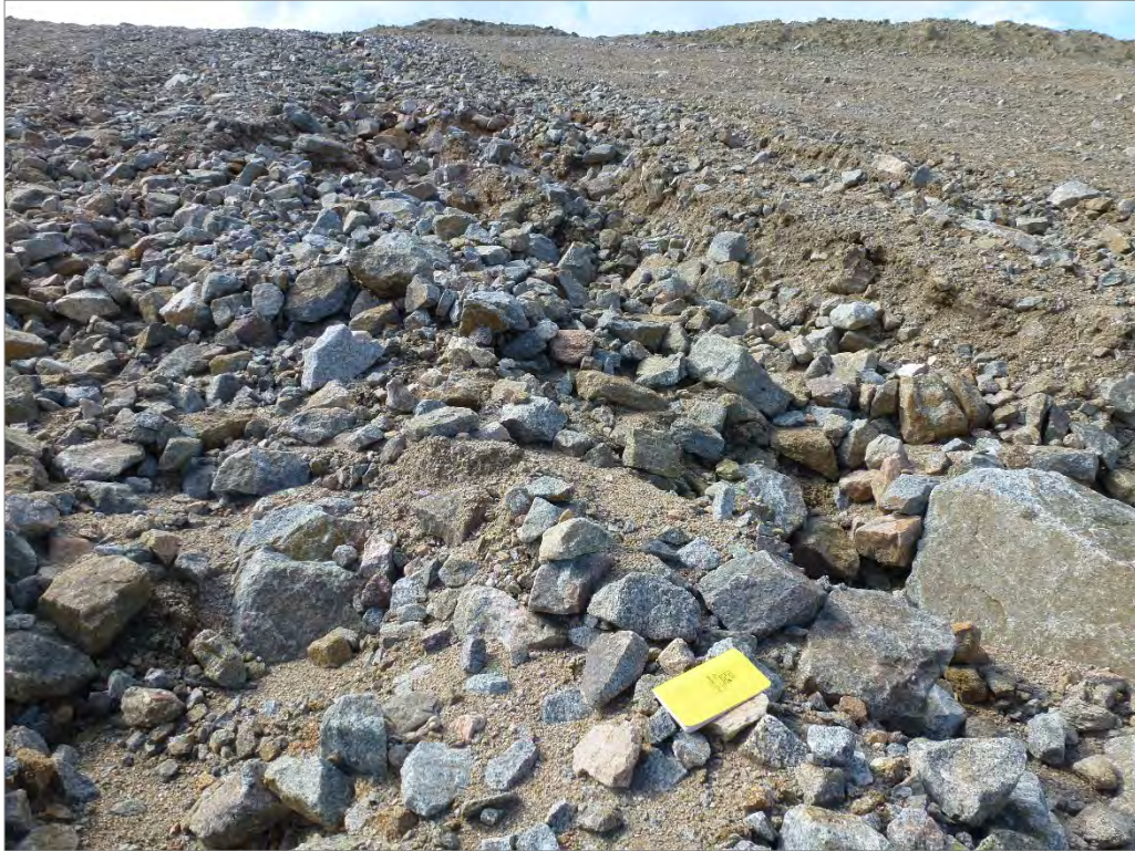
Photo 43: Eroded portion of the regraded slope due to the 2016 dewatering of ponded water from the area west of SWD and south of the former Ice-rich Overburden Dump
