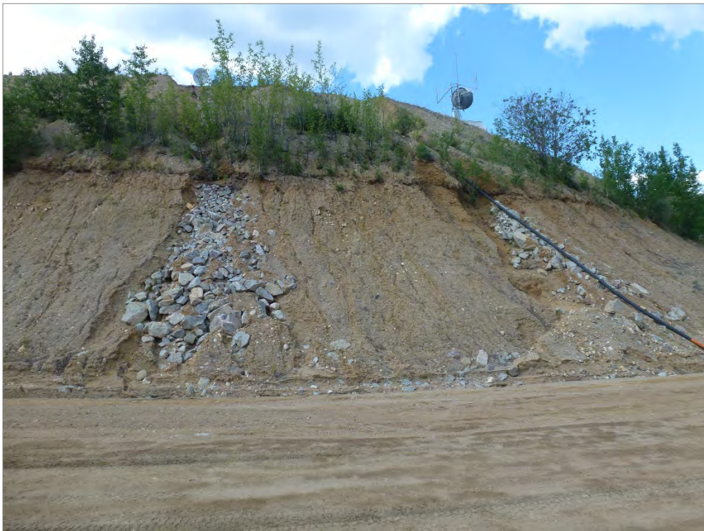
Photo 57: Erosion gullies with rockfill armoring on the slopes of the Camp Site pad (looking north)
