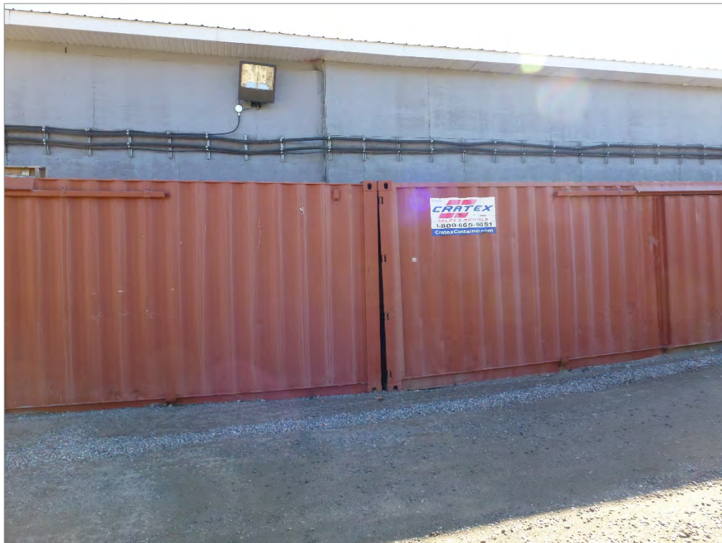
Photo 105: Observed settlements in the Underground Maintenance Shop adjacent to the Area 2 Pit Stage 3
