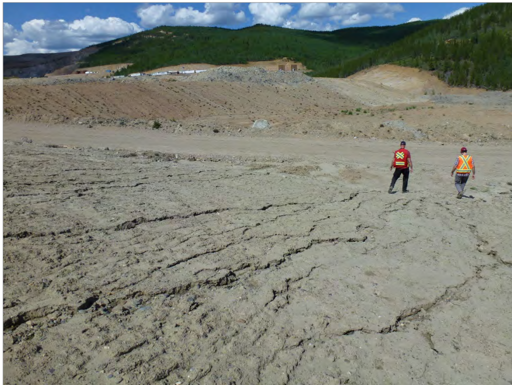
Photo 12: Multiple erosion gullies forming on closure cover (looking northwest)
