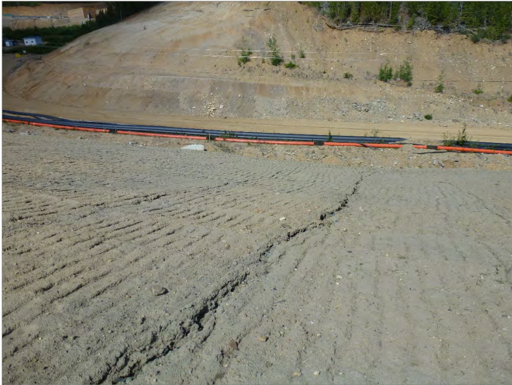
Photo 17: Erosion gully (looking north)
