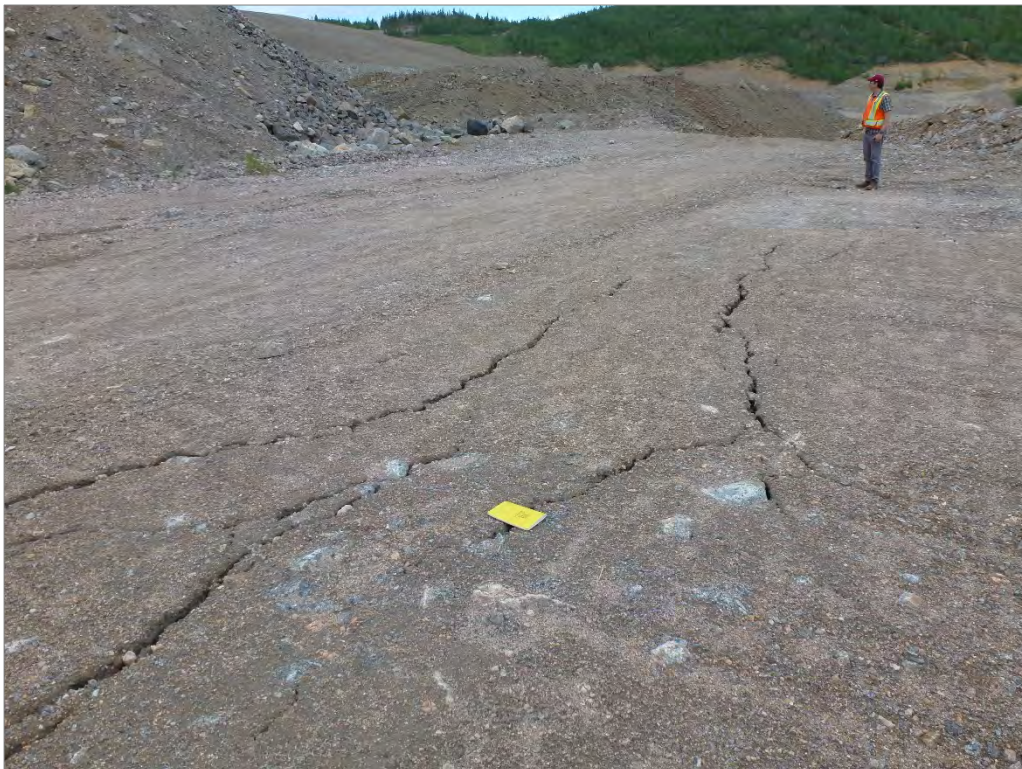
Photo 32: Cracking on the crest of the MWD Wrap (looking north)
