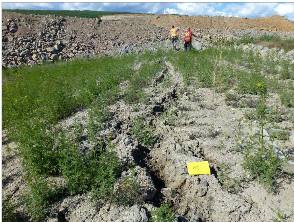
Photo 8: Settlement cracking along crest of placed cover material (looking west)
