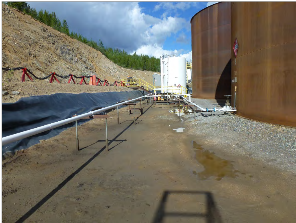
Photo 61: Inside Fuel Containment Facility (looking east)
