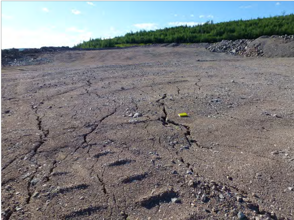
Photo 93: Further cracking in MPD crest (looking east)
