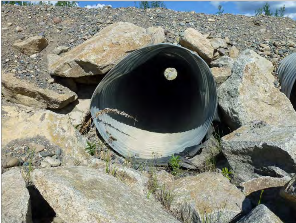
Photo 83: One of the four road culverts partially deformed
