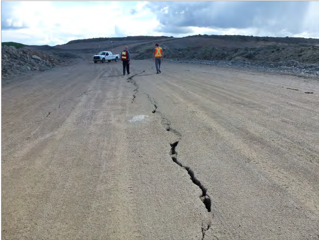
Photo 45: Observed longitudinal cracking on the crest
