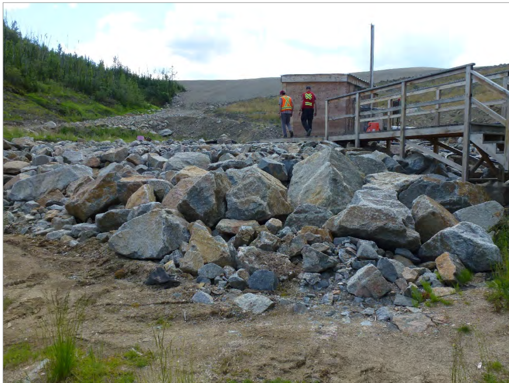
Photo 19: Seepage collection system downstream of the MVFE
