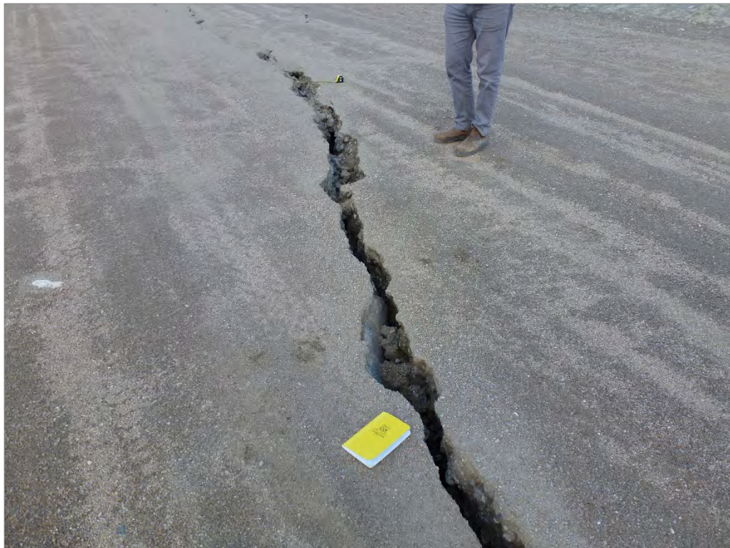
Photo 46: Close-up of longitudinal cracking at the widest point
