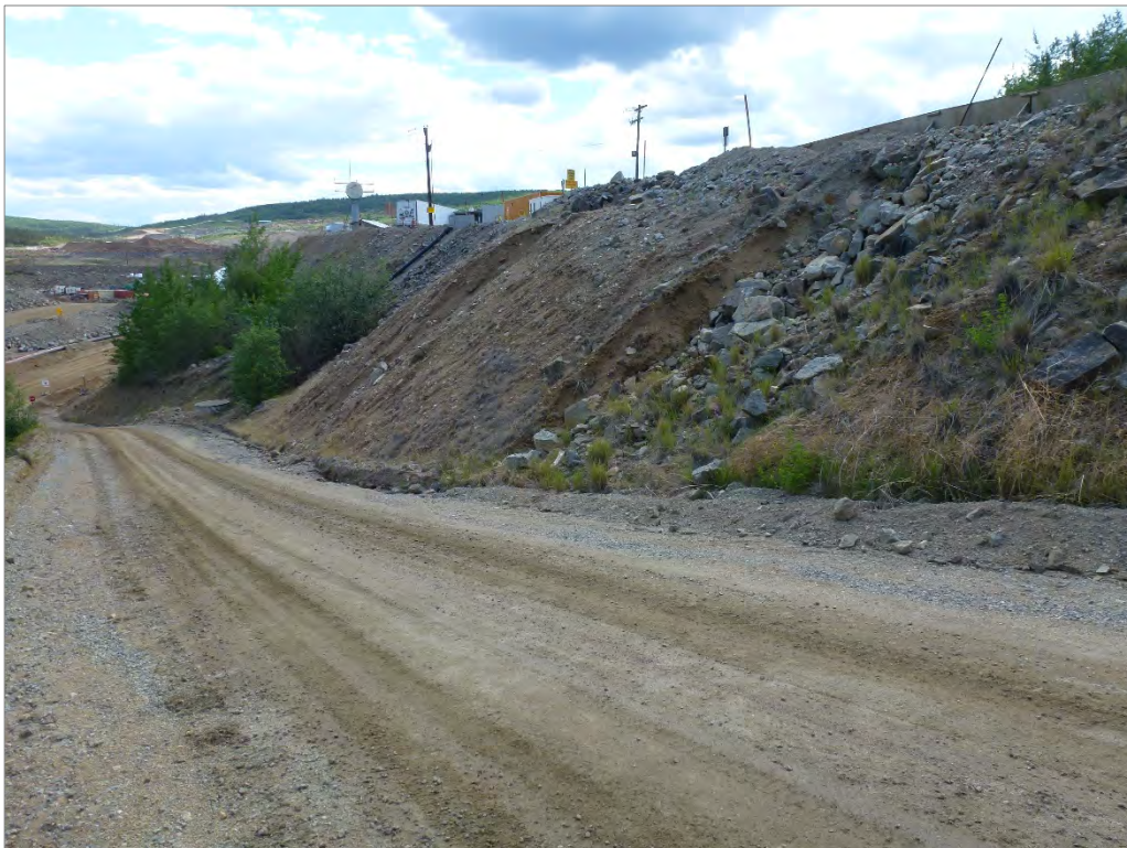
Photo 58: Erosion gullies on the slopes of the Camp Site pad (looking south)
