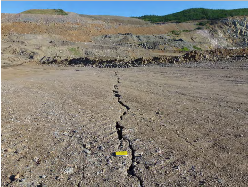
Photo 90: Cracking observed where MPD has expanded (looking north)
