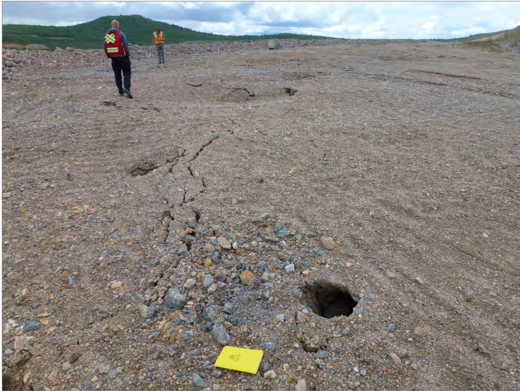
Photo 35: Small sinkholes and cracking on the crest of the MWD Wrap (looking west)
