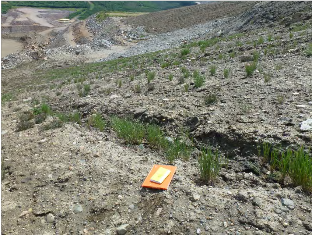
Photo 29: Erosion gully on MWD
