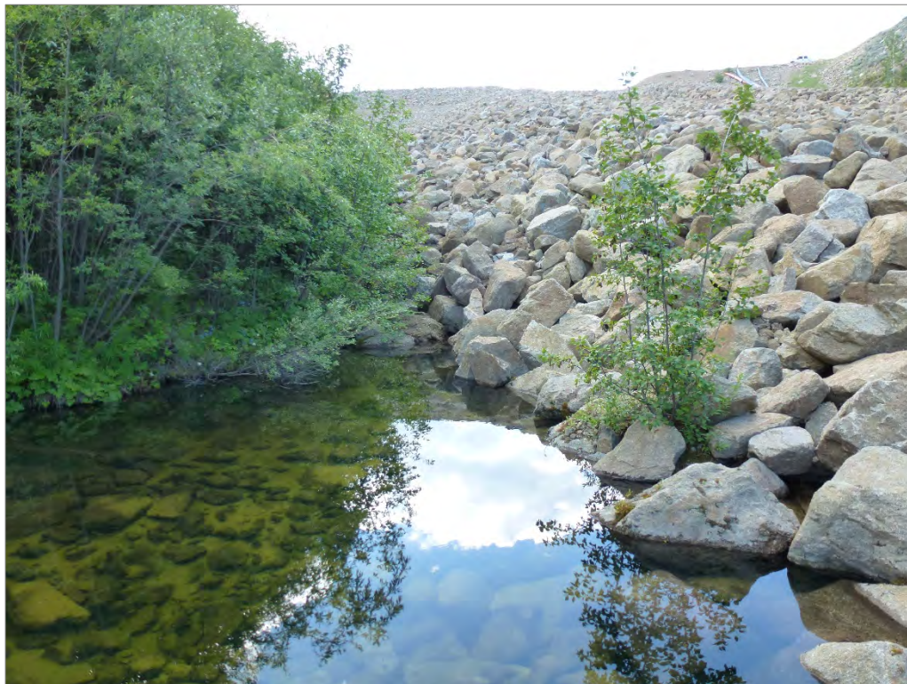
Photo 73: Ponding seepage downstream of WSP Dam – looking back towards the downstream slope.
