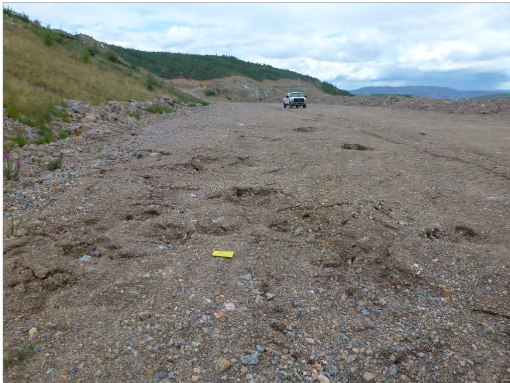
Photo 34: Area of differential settlement and small sinkholes (looking east)
