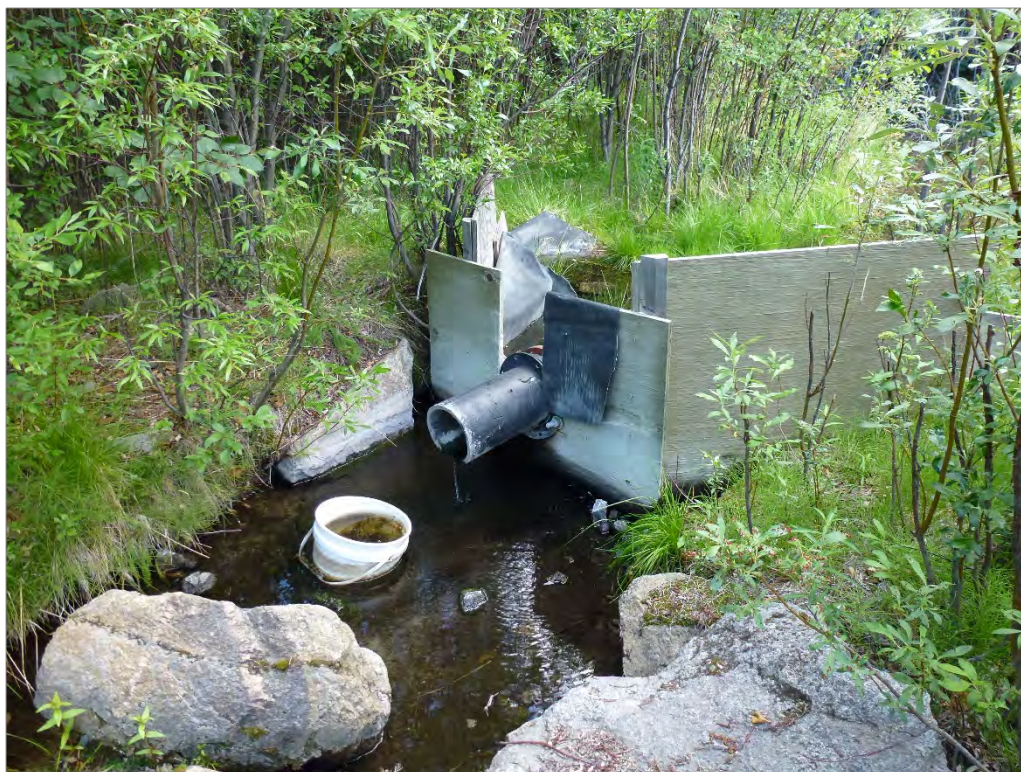
Photo 74: Outlet of the ponded seepage water
