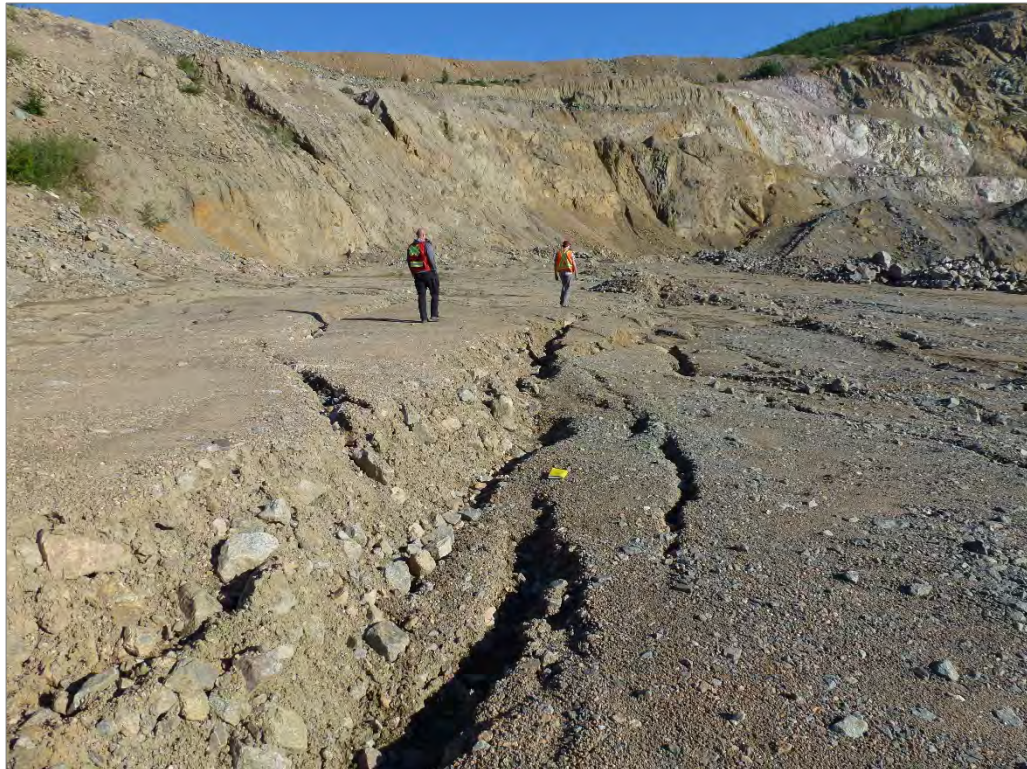
Photo 87: Longitudinal cracking in In-Pit Dump crest (looking northwest)
