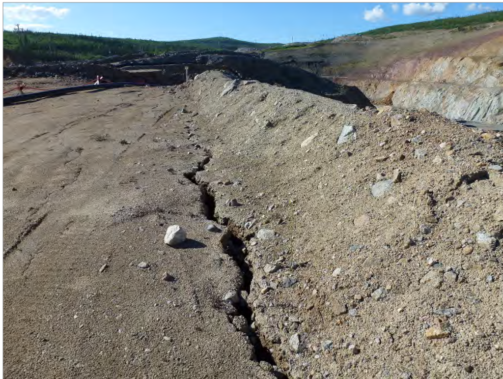
Photo 99: Observed cracking in access road along pit rim
