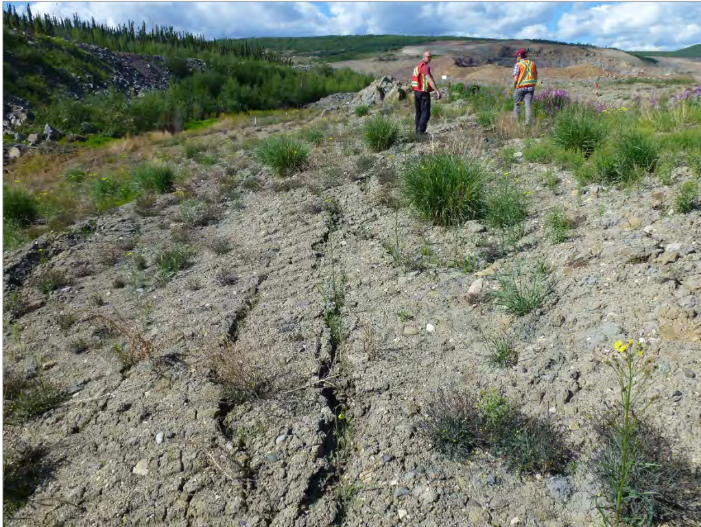
Photo 5: Settlement cracking along crest of placed cover material (looking west)
