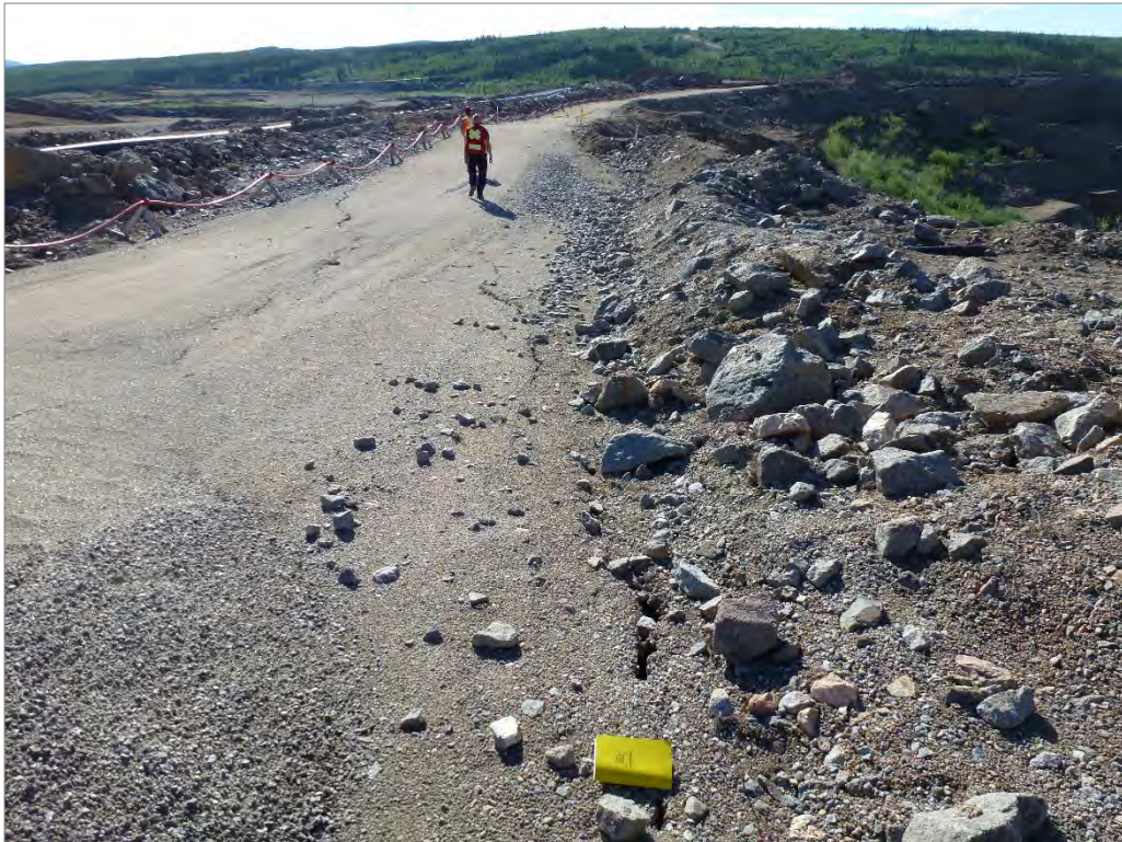
Photo 97: Cracking observed in access road along pit rim
