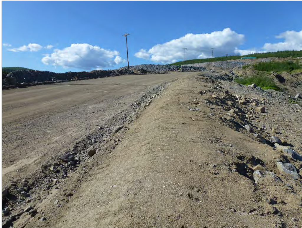
Photo 106: Haul road upstream of Area 2 Pit Stage 3 with surface water diversion berm (looking south)
