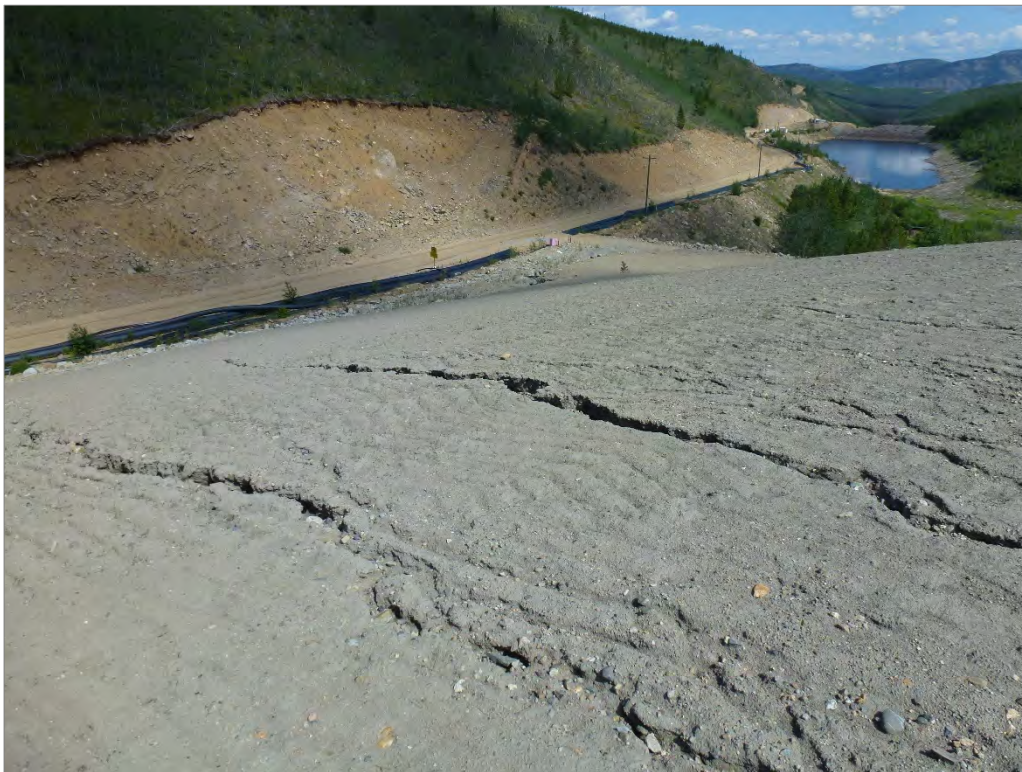
Photo 15: Erosion gullies (looking northeast)
