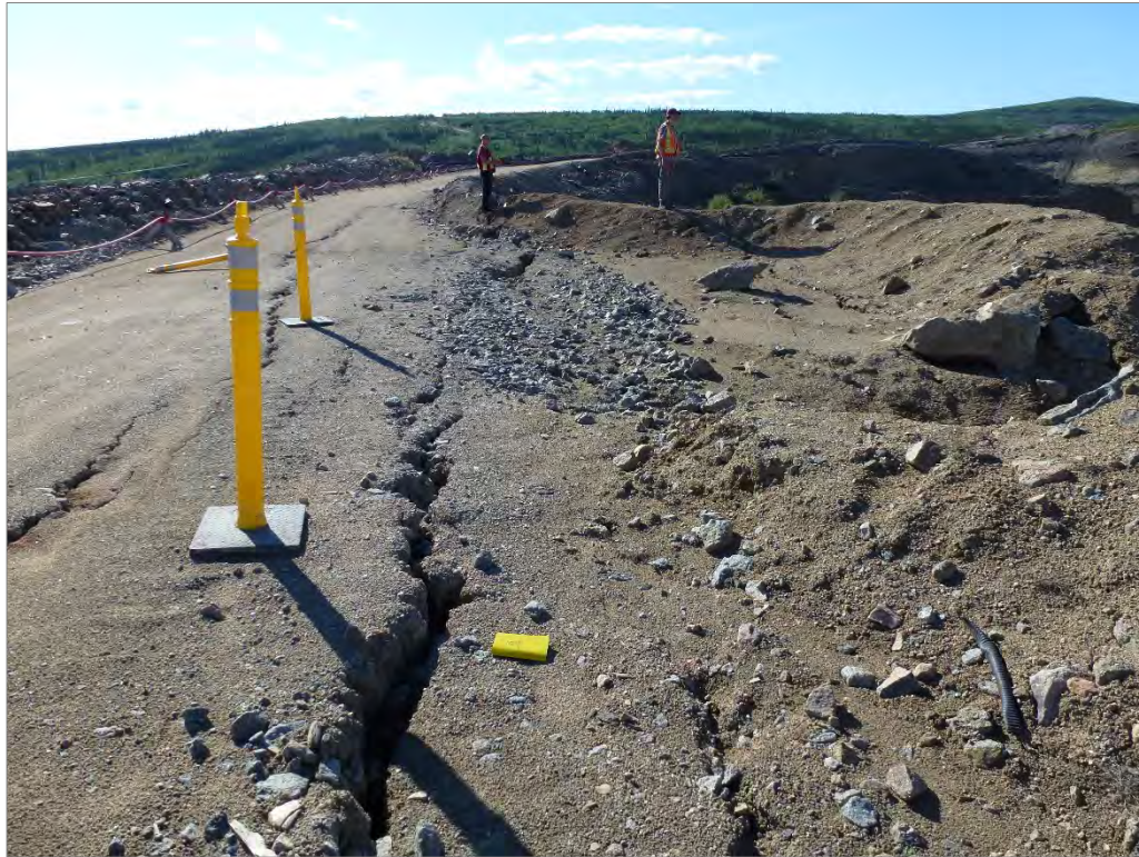
Photo 98: Observed cracking in access road along pit rim
