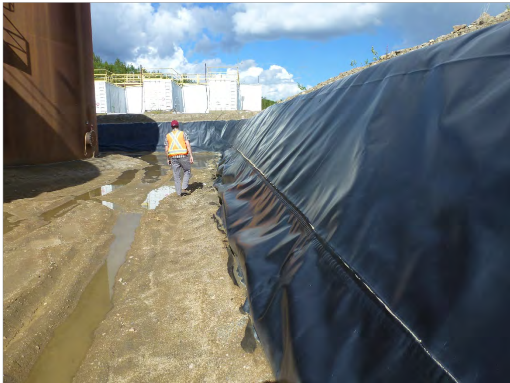
Photo 60: Inside Fuel Containment Facility (looking east)
