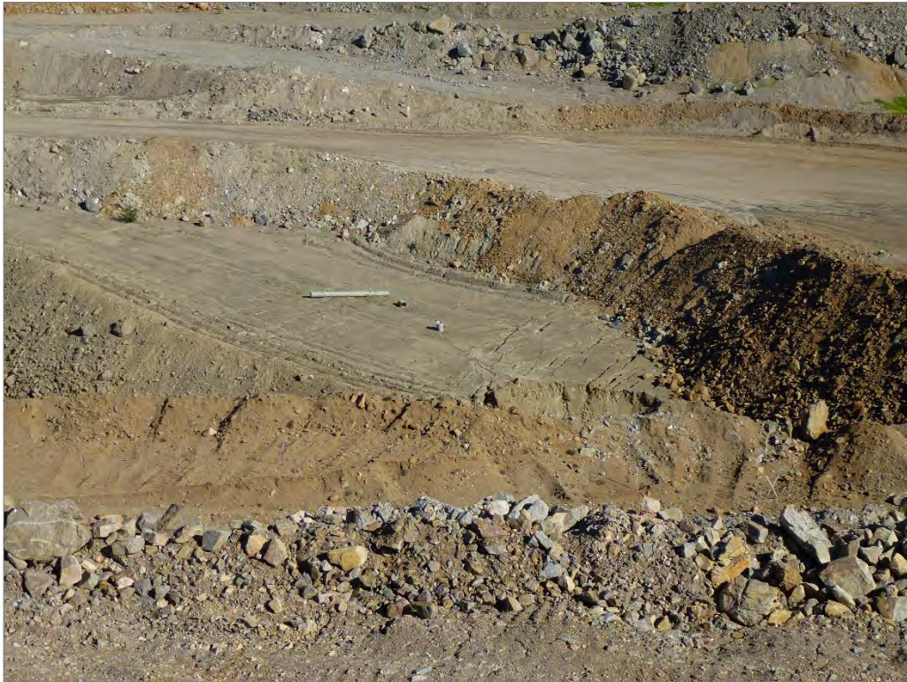
Photo 94: Cracking MPD (looking north)
