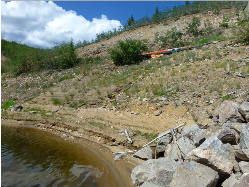
Photo 65: Minor erosion upstream of the WSP dam close to the north abutment
