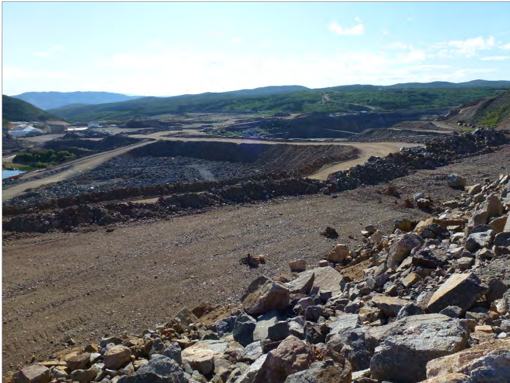
Photo 95: View of the South Wall Buttress from the MPD crest (looking north)
