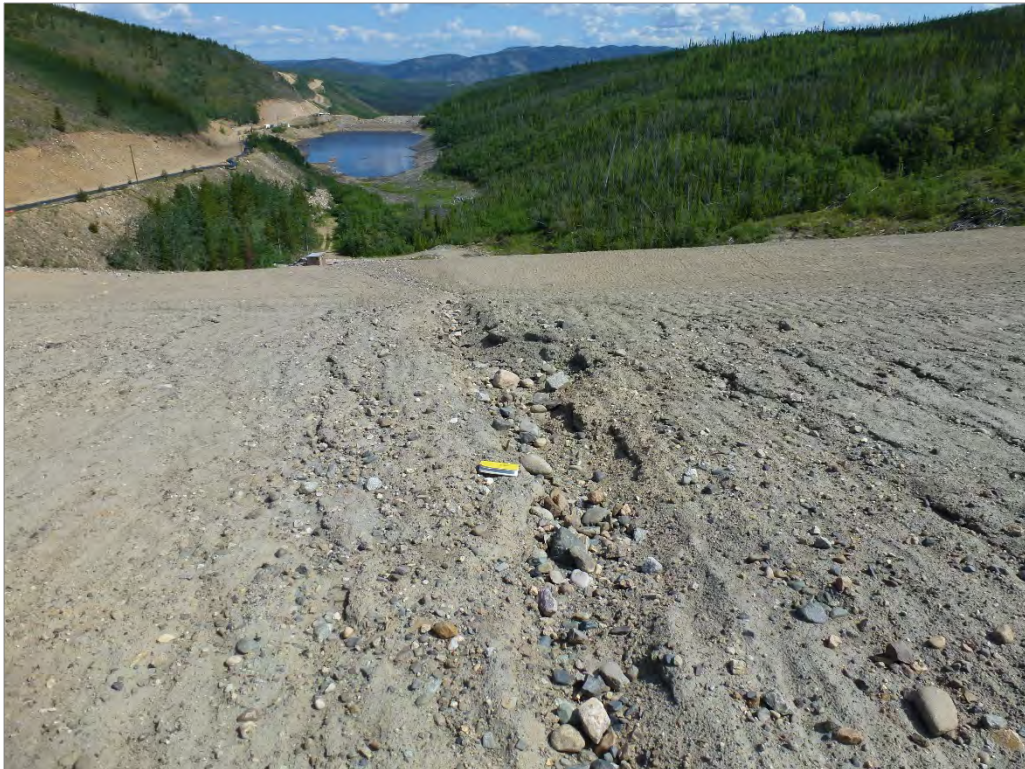
Photo 14: Erosion gullies – looking east towards the WSP
