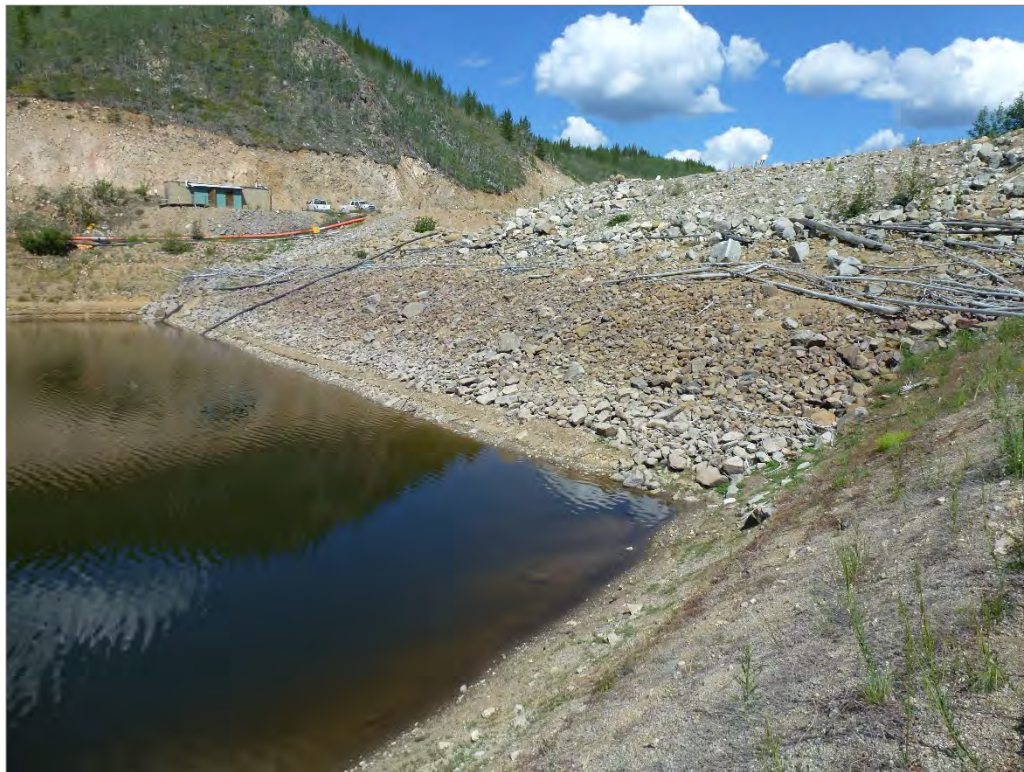
Photo 67: Upstream face of the WSP Dam – looking north from the south abutment.
