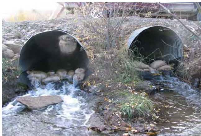
Plate 2. Temporary fish barriers placed at the outlets of Road crossing culverts – Km. 11, Minto Mine Road.
