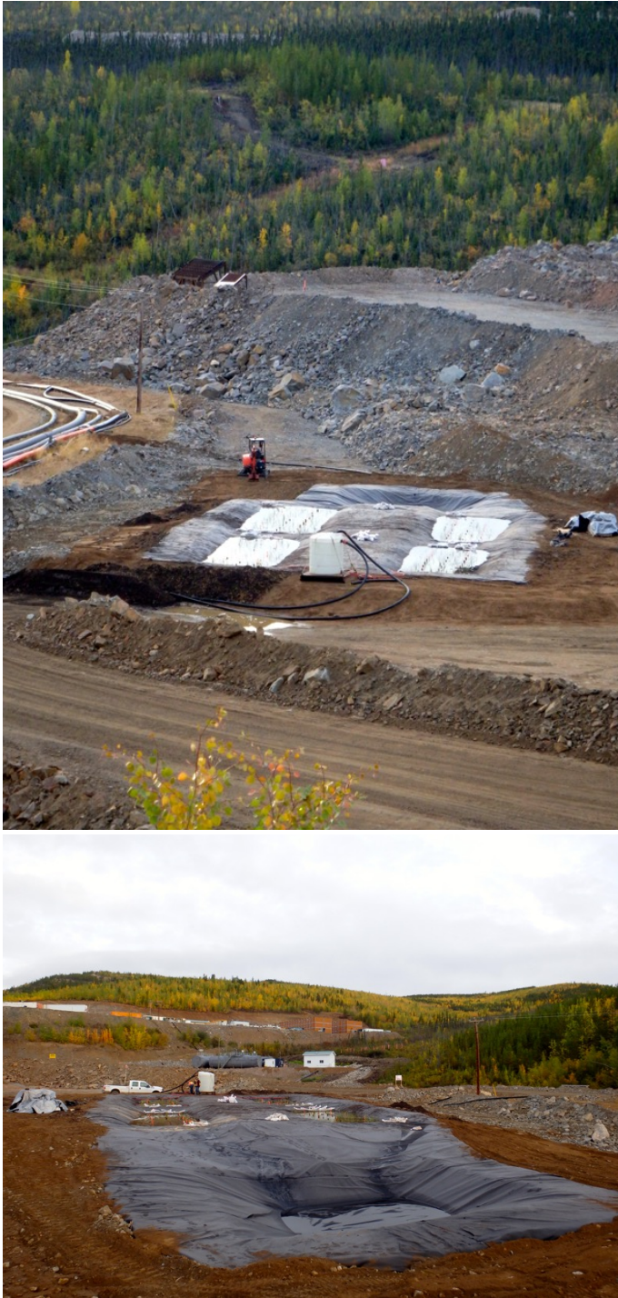
Figure 15. Demonstration-scale CWTS immediately after planting and filling with water (August 29, 2014). Top, photograph taken from camp behind kitchen looking down at inflow of CWTS; bottom, photograph taken from outflow holding pond looking towards camp in background.
