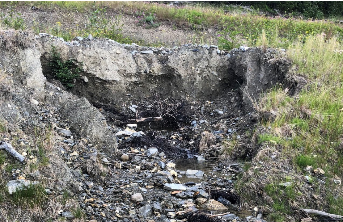
Photo 12 North Drainage Channel subsidence
