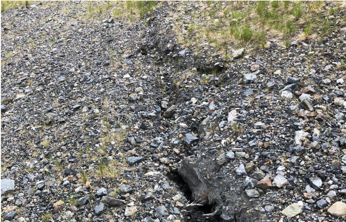
Photo 15 Tension crack in fill at the Burnick Waste Rock Dump
