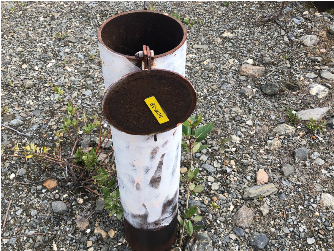
Photo 3 Piezometer NDW 3A protective cap
