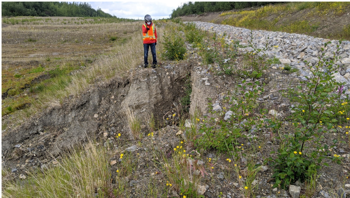
Photo 10 Subsidence in the berm adjacent to the North Drainage Channel
