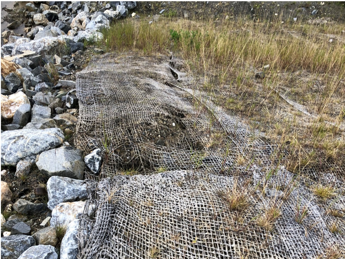
Photo 8 Downstream slope of SRS with shallow erosion rill
