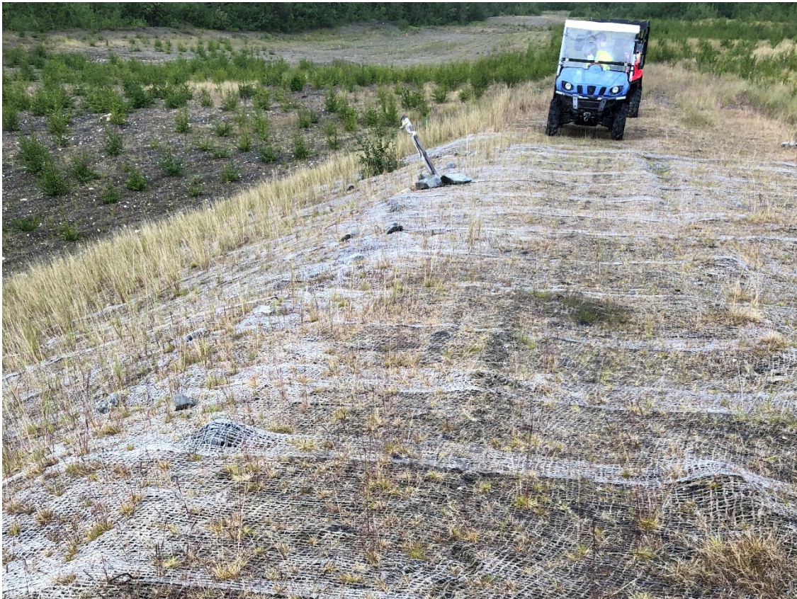
Photo 7 View west of the SRS crest. Note vegetation and geogrid for stabilization
