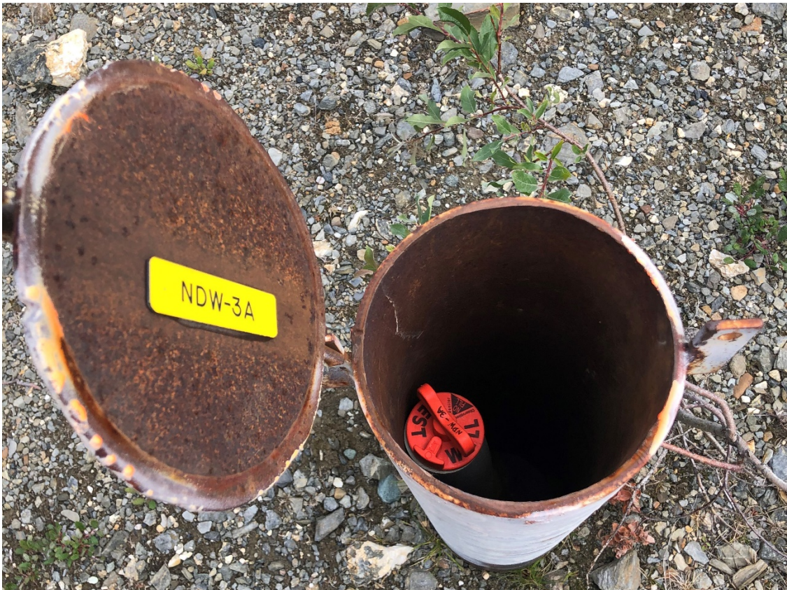
Photo 4 Piezometer NDW 3A PVC Standpipe with red cap
