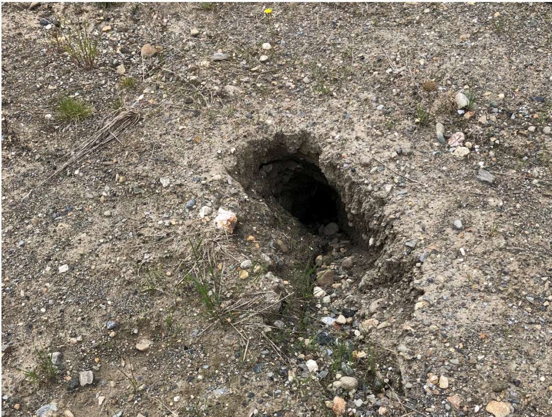
Photo 14: Small sink hole in the landfill south of the North Dam
