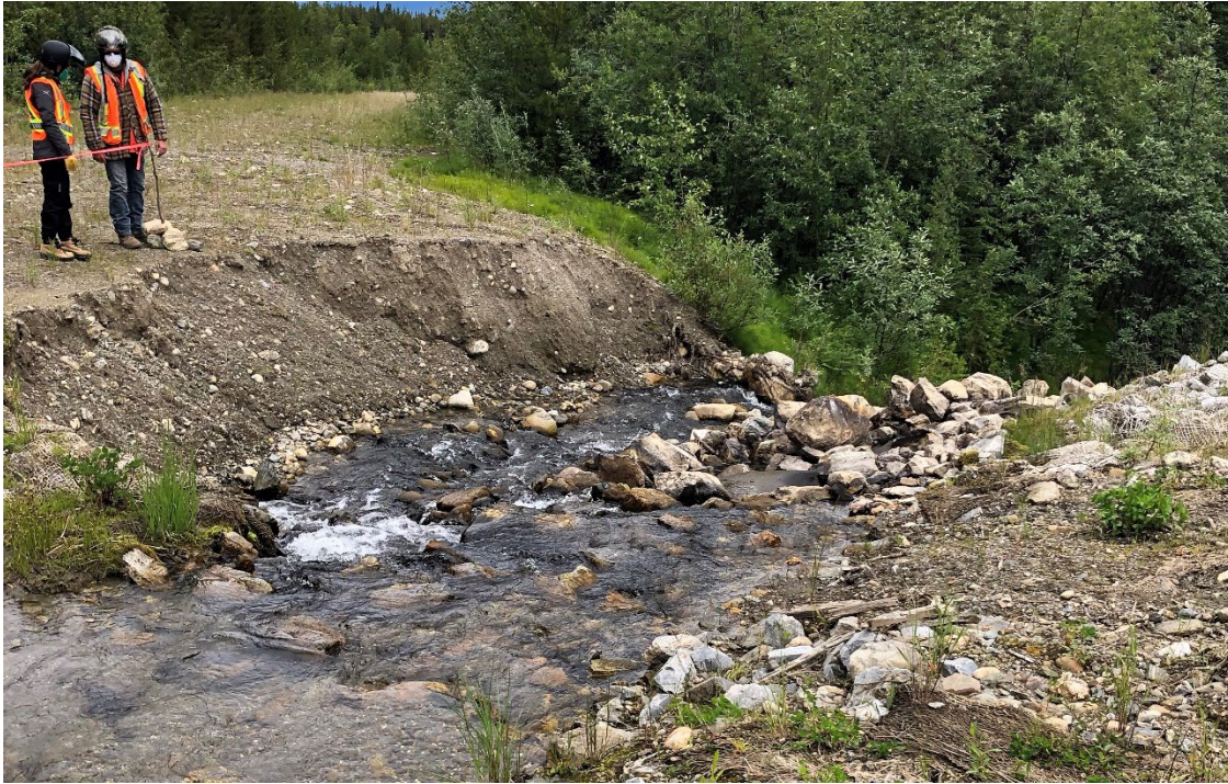
Photo 13 Subsidence in the channel slope at the North Creek second crossing
