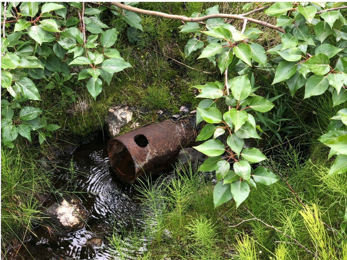
Photo 6 MH02 Flow Monitoring Pipe
