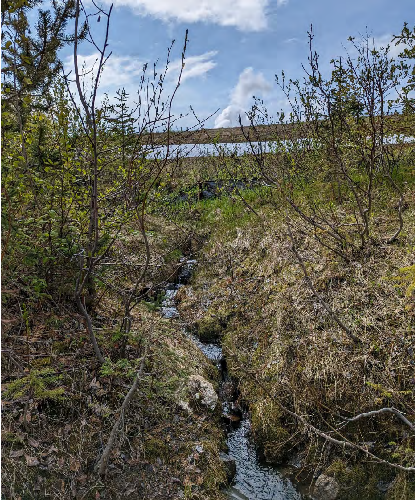
Photo NE-09: North embankment seen from the seepage monitoring station location. The flow appears to be clear.
