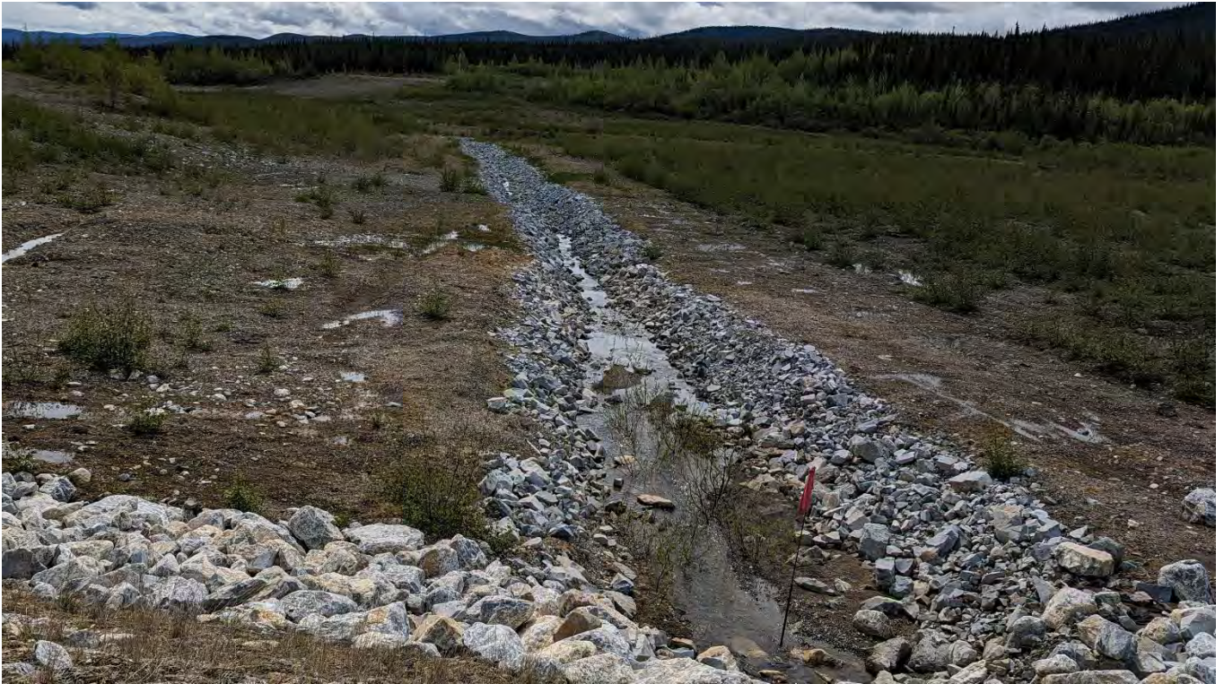
Photo SRS-03: Sediment accumulation in the spillway outlet seen from the east margin of the spillway.
