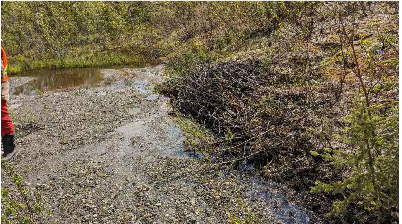
Photo NE-10: Seepage observed at the dam toe during the inspection.
