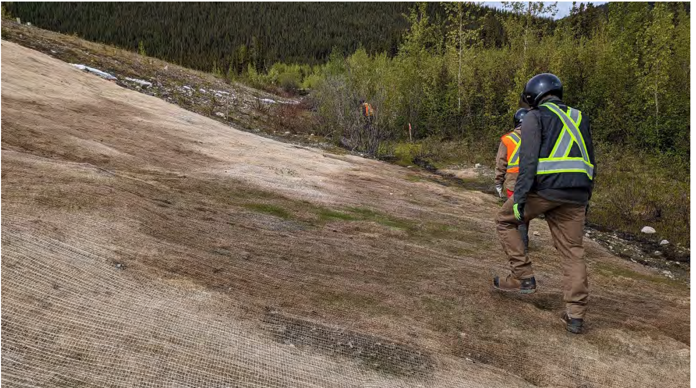
Photo NE-11: North embankment gully repair erosion protection mat at the toe was wet and the material underneath was soft.
