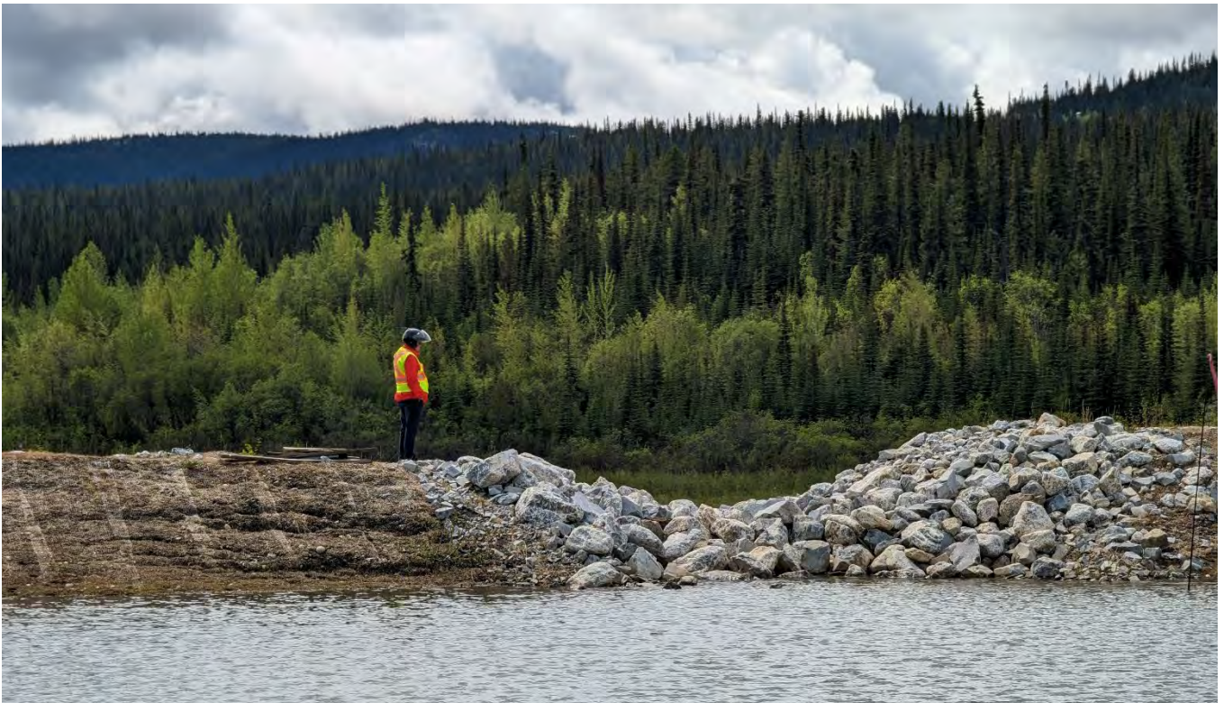
Photo SRS-04: The crest east of the spillway is lower in elevation compared to the west crest of the spillway with visible deformation observable on the upstream slope
