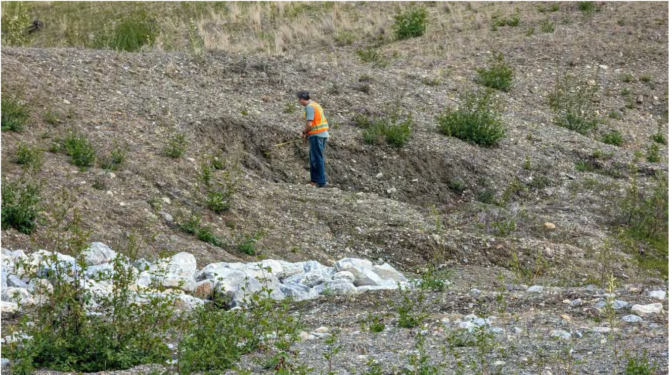
Photo SRS-05: Slough present on the downstream slope.
