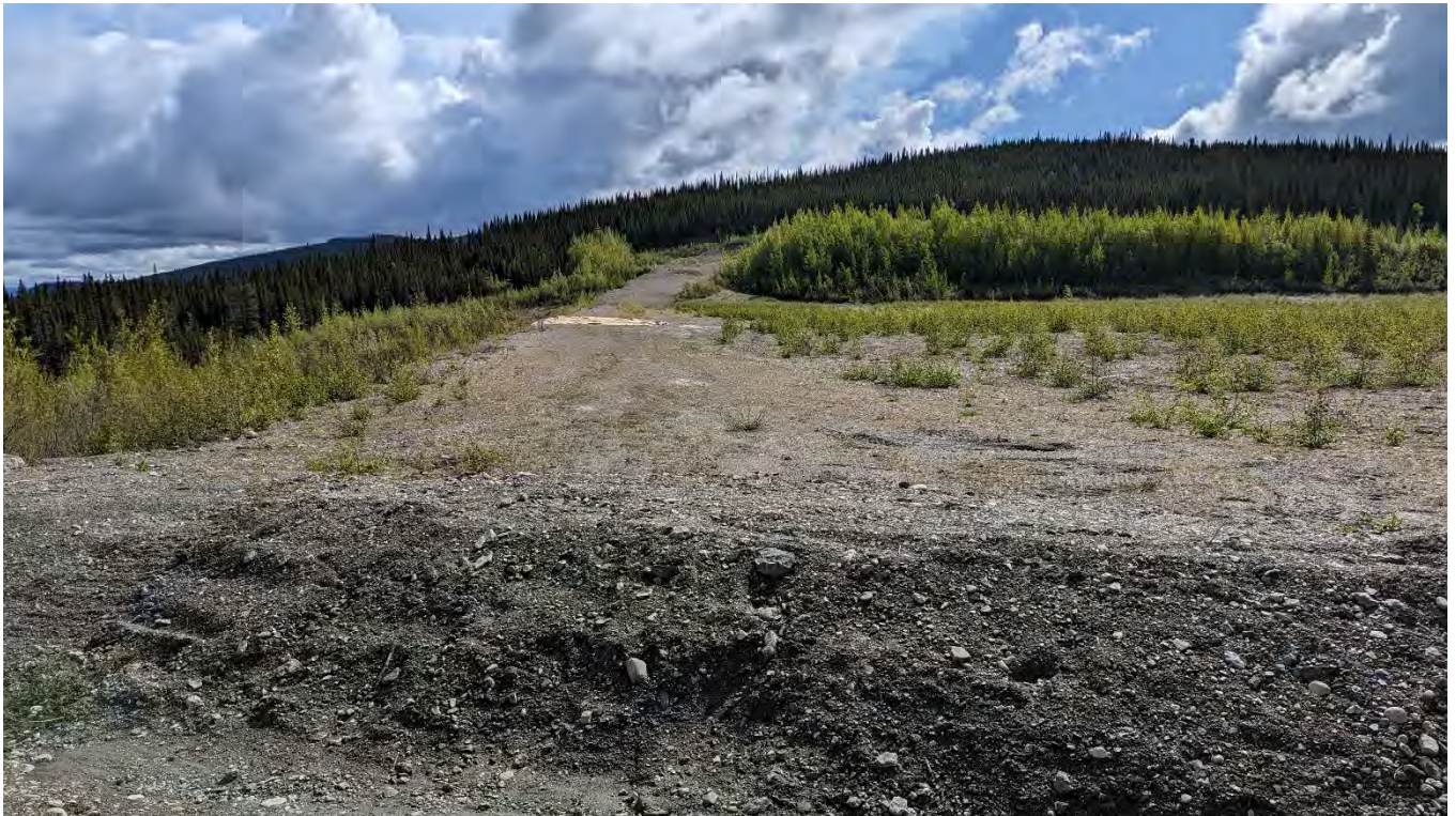
Photo NE-01: North Embankment alignment seen from the west abutment; it shows no abnormal deformation.
