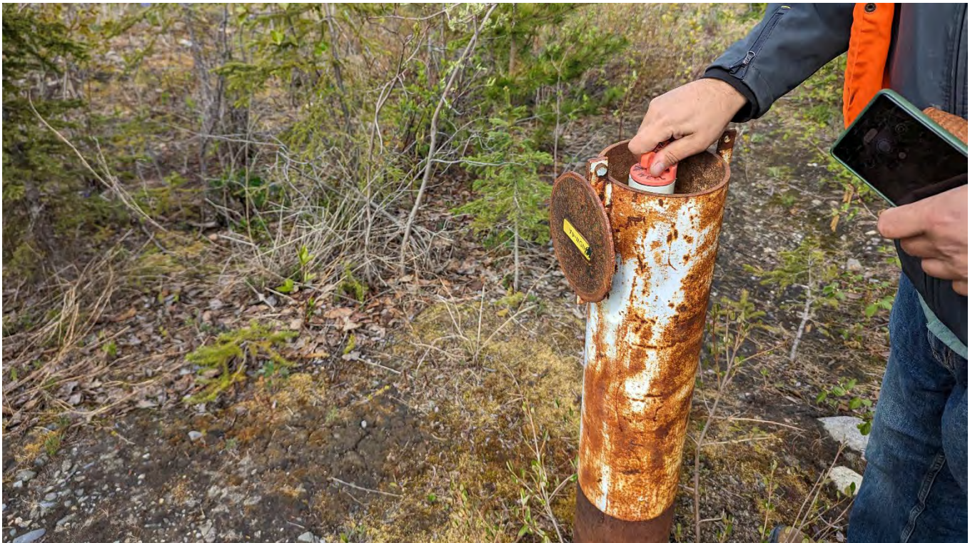
Photo NE-04: NDW-A4 Piezometer fitting in the casing after being trimmed following the 2022 recommendations.
