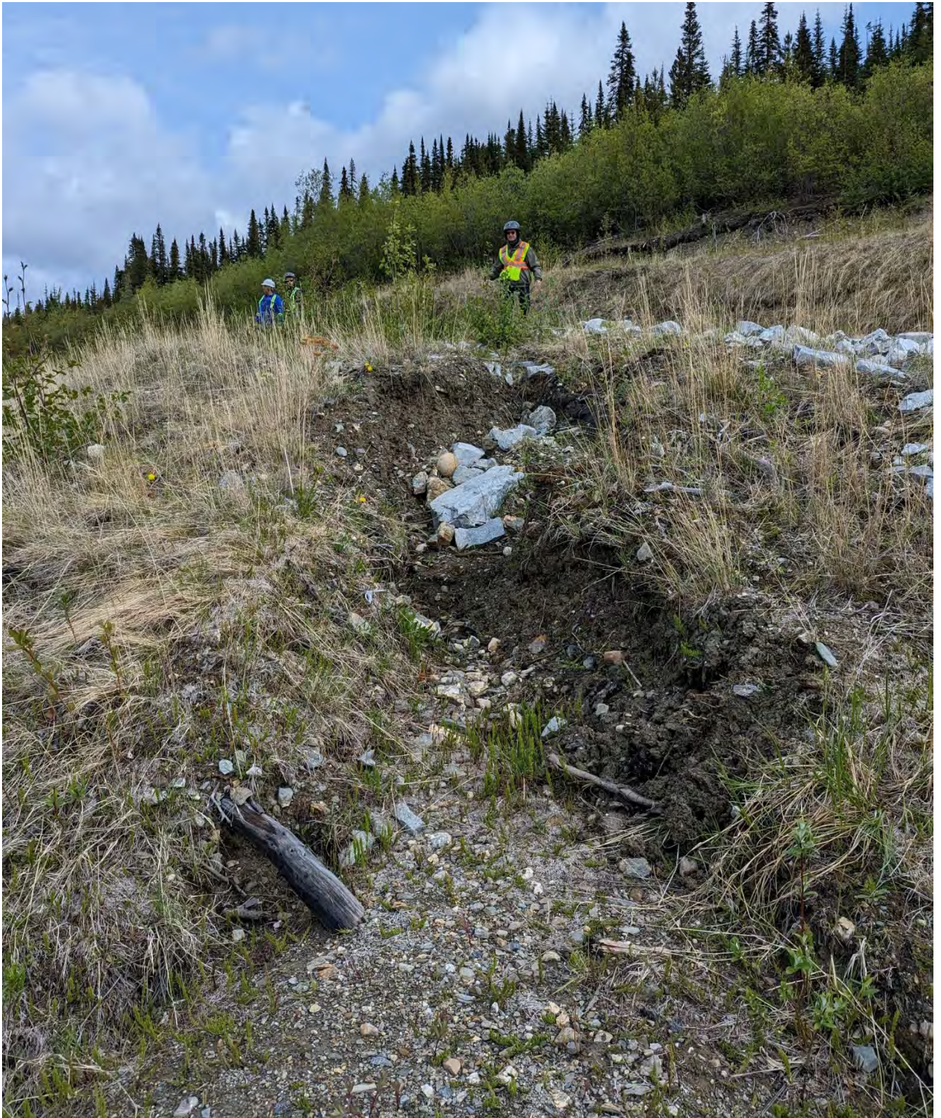
Photo NDC-02: Erosion gully immediately to the west of the riprap movement area.
