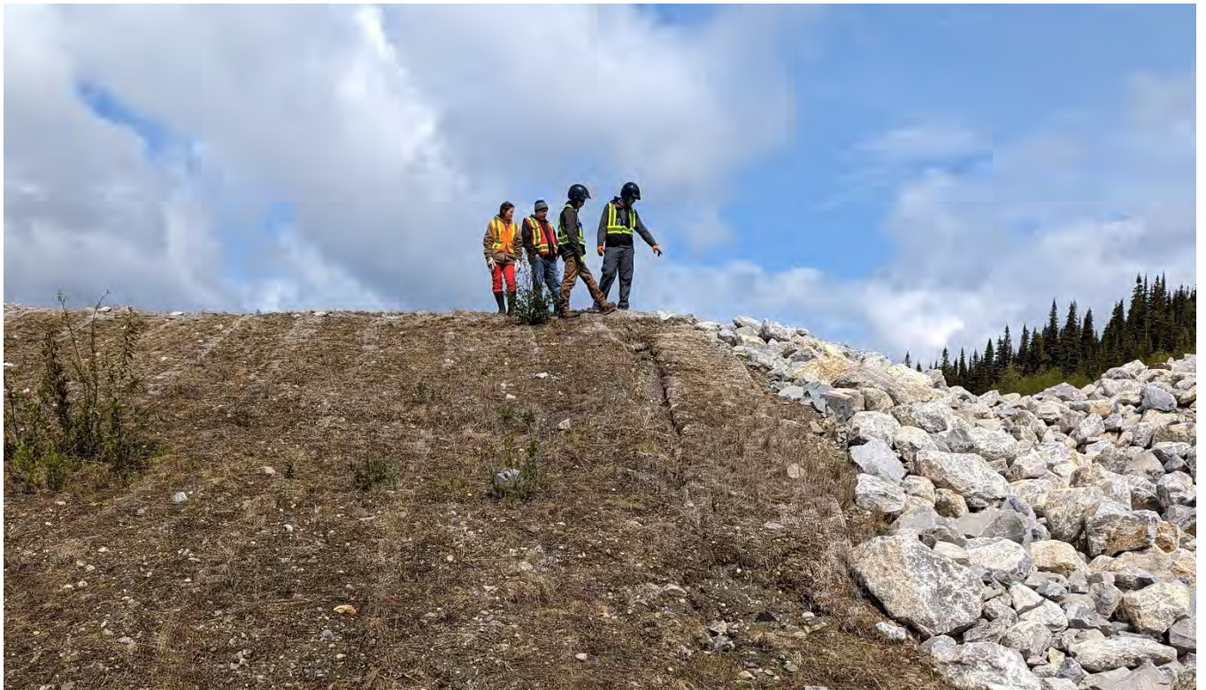
Photo SRS-02: Transverse crack across the dam crest approximately 1m east of the spillway seen from downstream.
