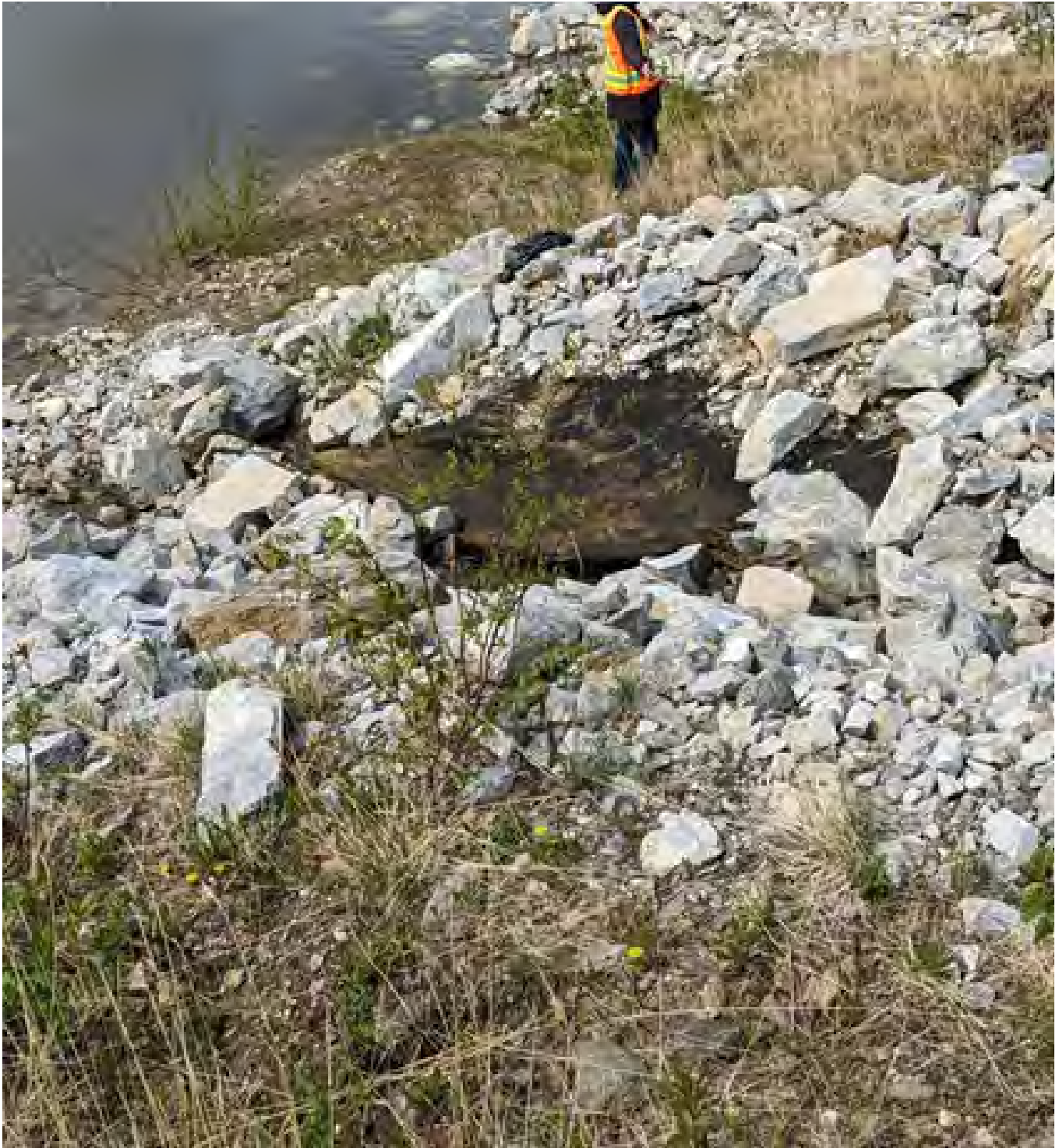
Photo NDC-01: Slippage of the riprap immediately upstream the channel outlet.
