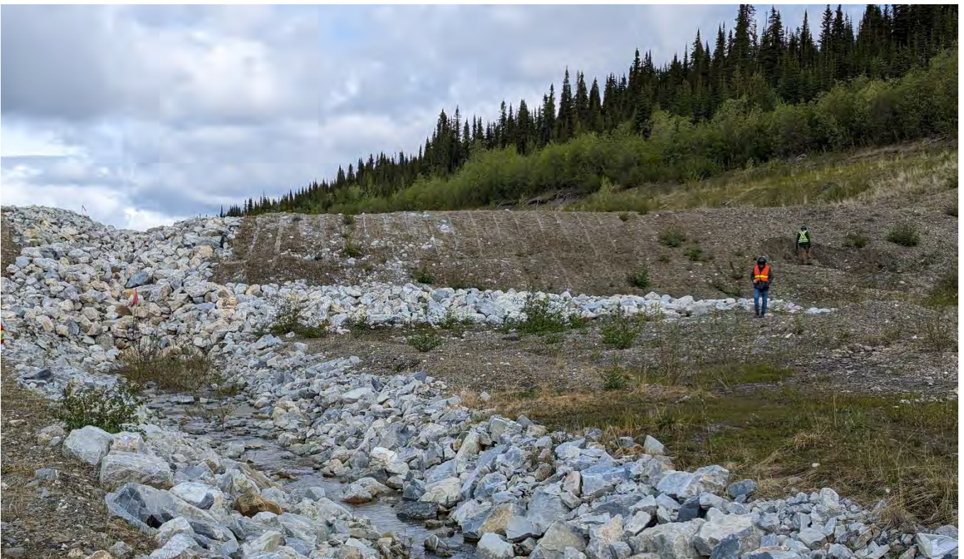
Photo SRS-06: Slough seen from downstream position. The slough is away from the spillway and the ponded water area, and approximately 8 meters from the east abutment.
