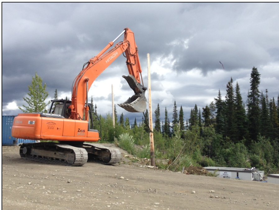
ELEC Photograph 6: IKC excavator working on behalf of CIPC removing power pole near main gate area.
