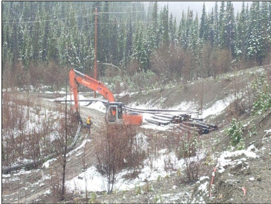
MISC Photograph 3: Removal, dismantling and stockpiling of pipeline along lower access road to TMA.
