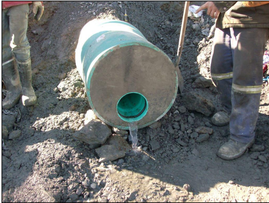
MTN Photograph 25: Burnick 1200 Portal drainage CSP-PVC connector.
