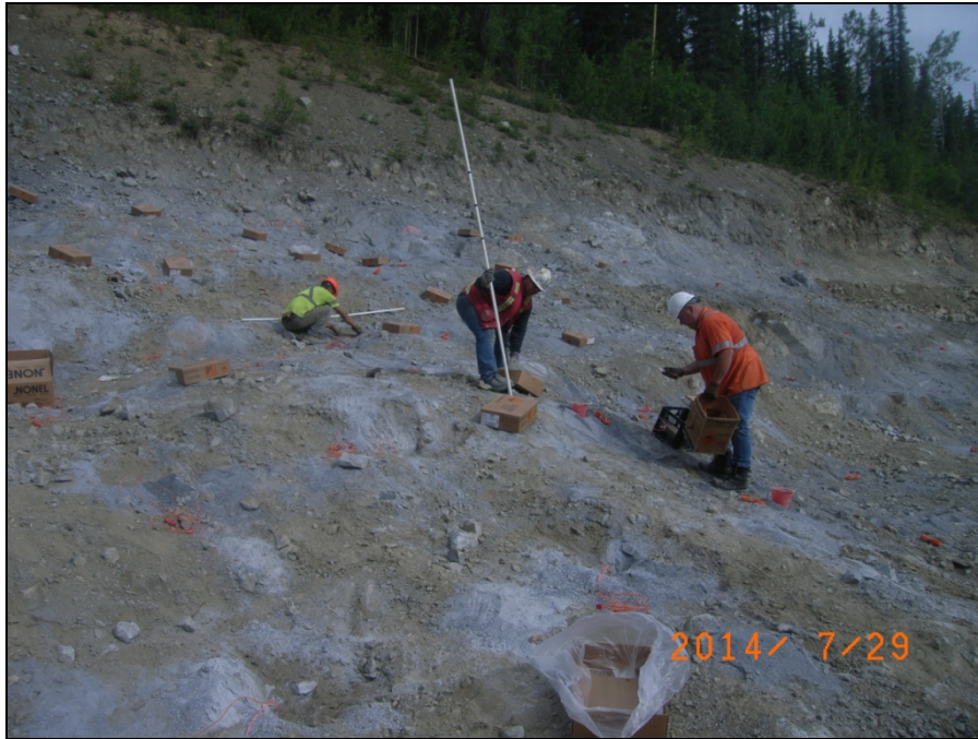
TMA Photograph 7: Blasting contractor measuring hole depths and setting charges at km 17 quarry.
