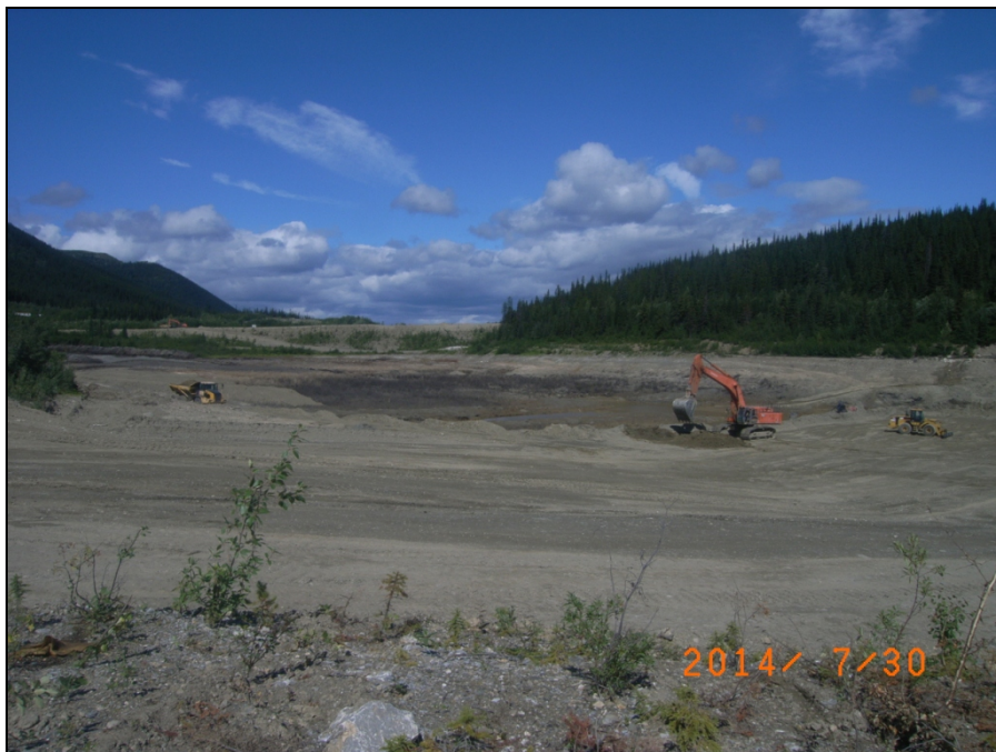
TMA Photograph 8: Reclaim Dam excavation nearing completion and capping of Reclaim Pond in progress.
