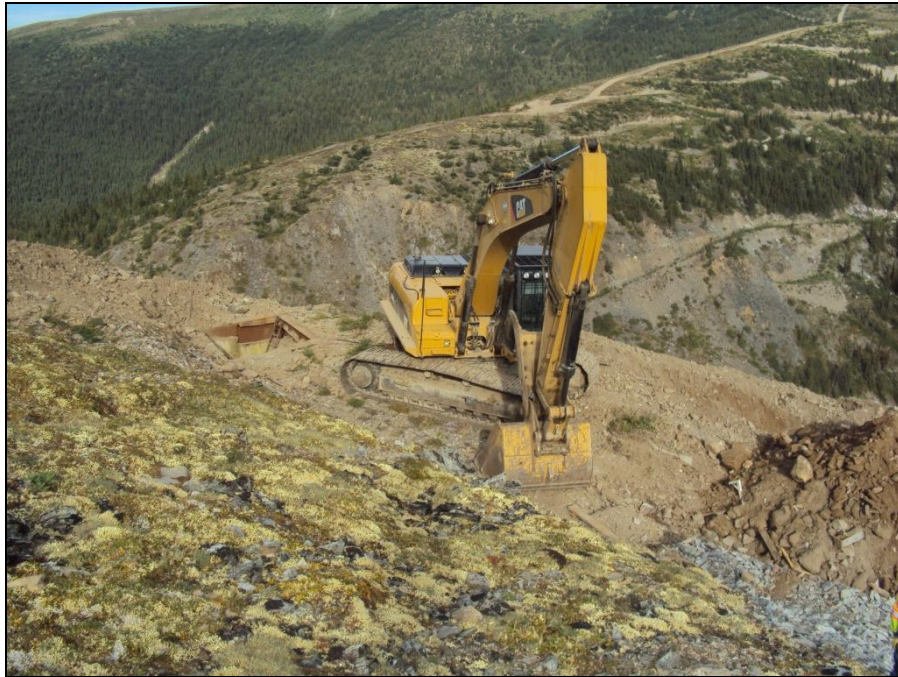
MTN Photograph 13: Jewelbox Summit Ventilation Raise (just left of excavator) before construction of permanent cap.
