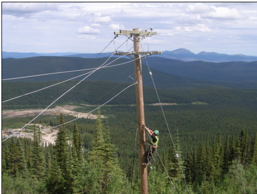
ELEC Photograph 4: CIPC disconnecting cable from power pole near Jewelbox waste rock dump.
