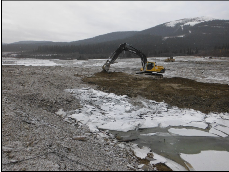
TMA Photograph 19: Capping of “deep tailings cell” in the former South Pond area using an excavator to place capping material.
