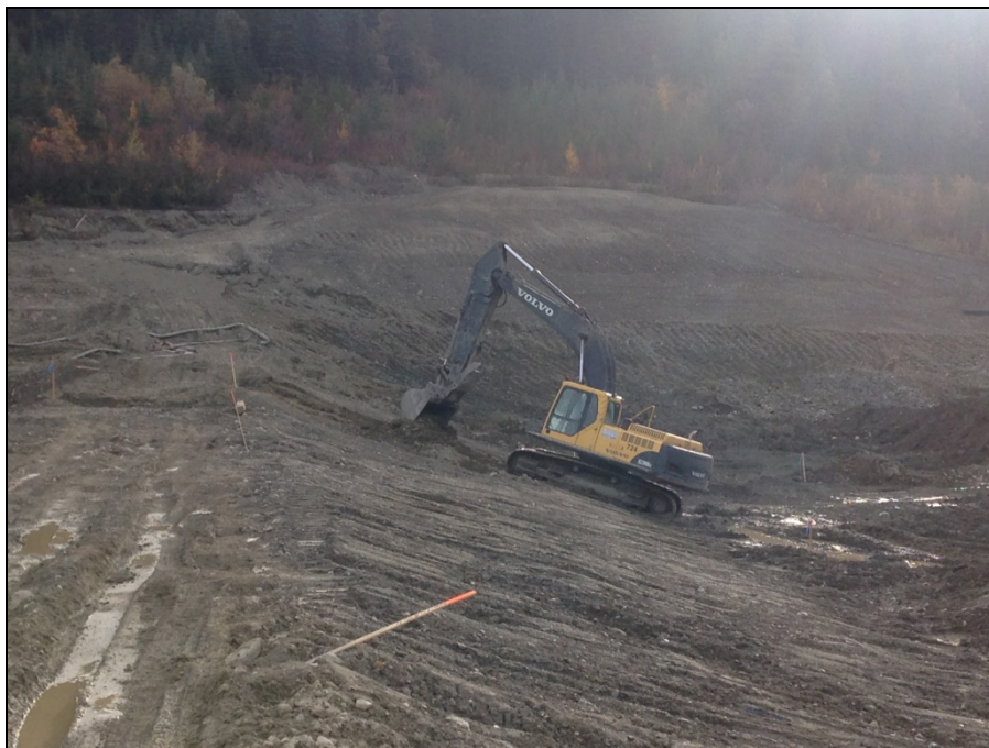
TMA Photograph 14: Excavator completing shaping of downstream slope of sediment retaining structure.
