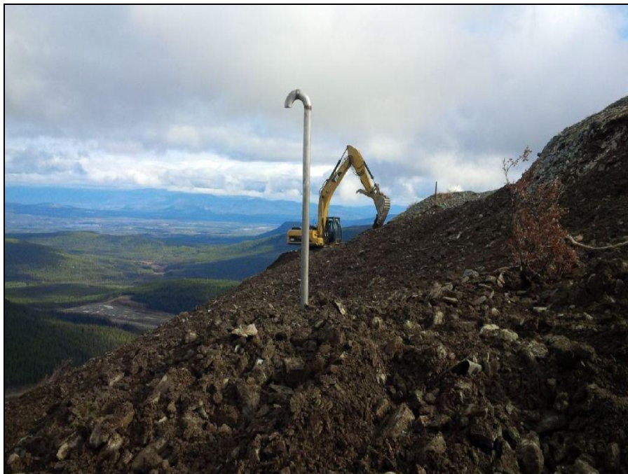
MTN Photograph 16: Jewelbox Summit Ventilation Raise cap completed and covered with stainless steel vent pipe protruding from slope.
