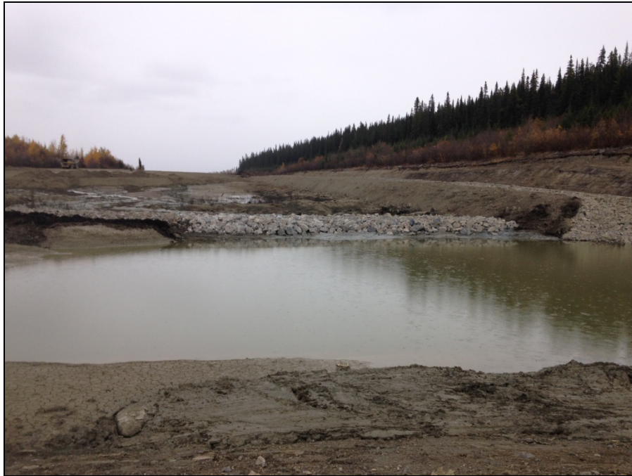
TMA Photograph 15: Looking north from sediment retaining structure toward sediment retaining pond and rock cofferdam, with North Drainage Channel along east bank of former South Pond.
