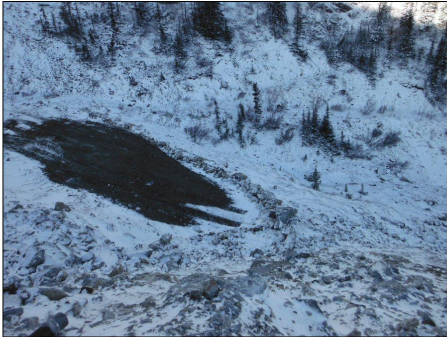
MTN Photograph 20: Capping of Jewelbox 1380 gully sediment pond with rock berm constructed.
