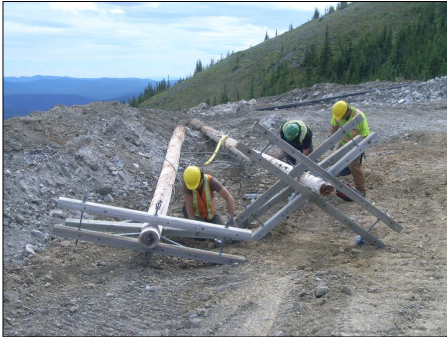
ELEC Photograph 3: CIPC technicians removing hardware from power poles near Jewelbox 1408 Portal.
