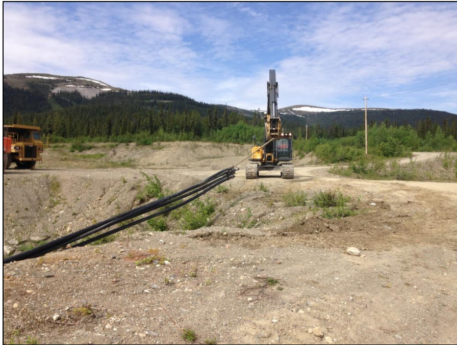
MISC Photograph 7: Excavator removing former siphon pipeline from exit chute of Camp Creek Diversion Channel.
