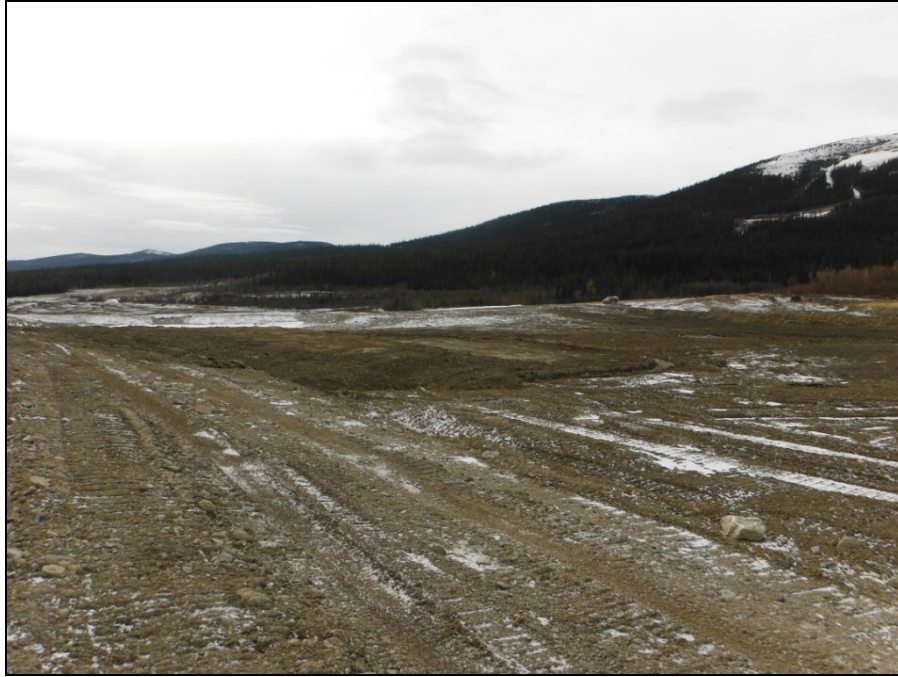
TMA Photograph 21: View from east bank of former South Pond looking south toward capped South Pond area with sediment retaining structure and spillway in background.
