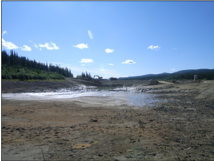
TMA Photograph 9: South Pond dewatering complete and South Dam excavation in progress.
