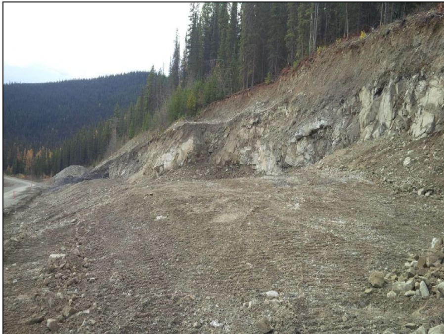
TMA Photograph 16: Reclamation of km 17 quarry site following extraction of riprap material.
