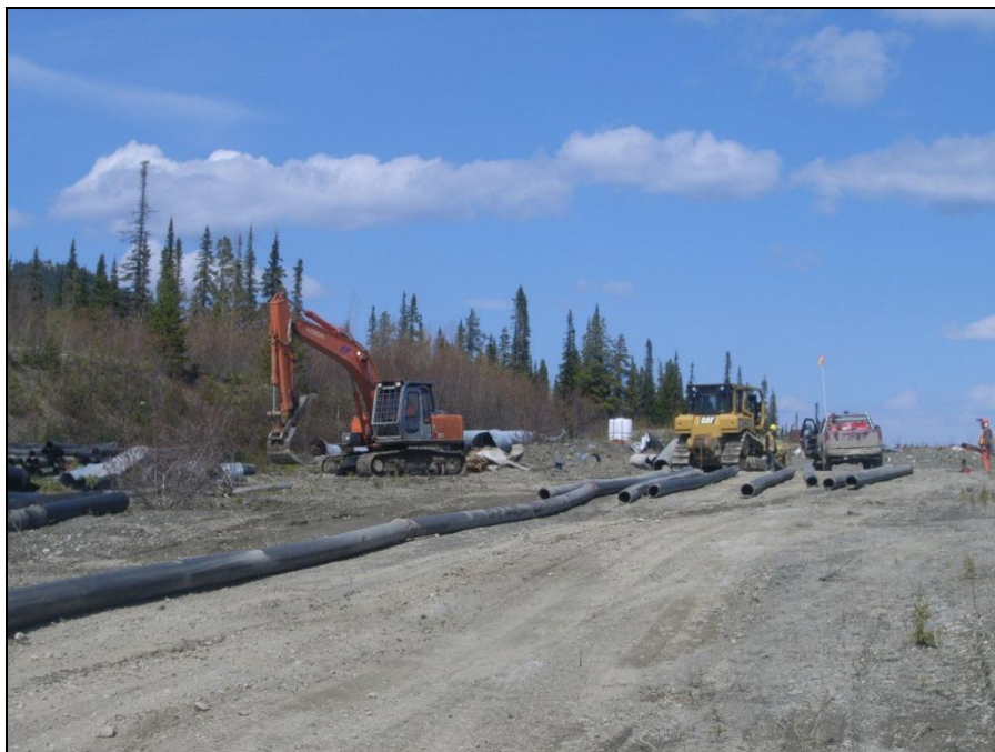
MISC Photograph 4: Boneyard clean-up including dismantling and stockpiling of pipeline for future off-site transport.
