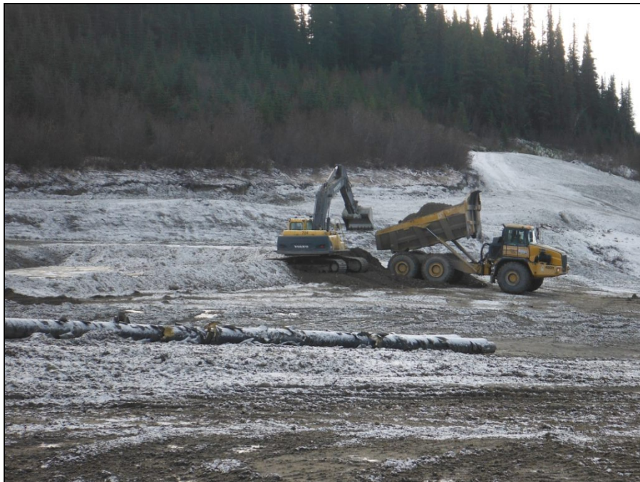
TMA Photograph 18: Construction of berm around “deep tailings cell” in the former South Pond area.
