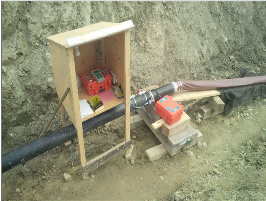
TMA Photograph 1: Dewatering discharge volume monitoring station.
