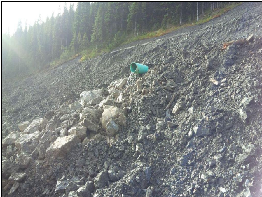
MTN Photograph 26: Burnick 1200 Portal drainage discharging from PVC pipe beneath reshaped waste rock.
