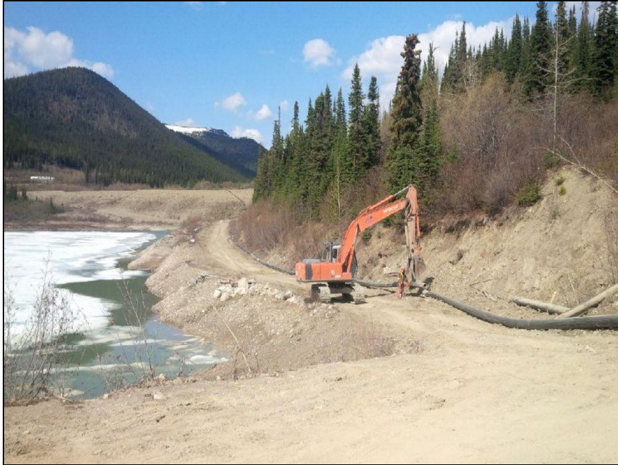
MISC Photograph 5: Assembly of pipeline along east side of Reclaim Pond in preparation for South Pond dewatering associated with the TMA Decommissioning works.
