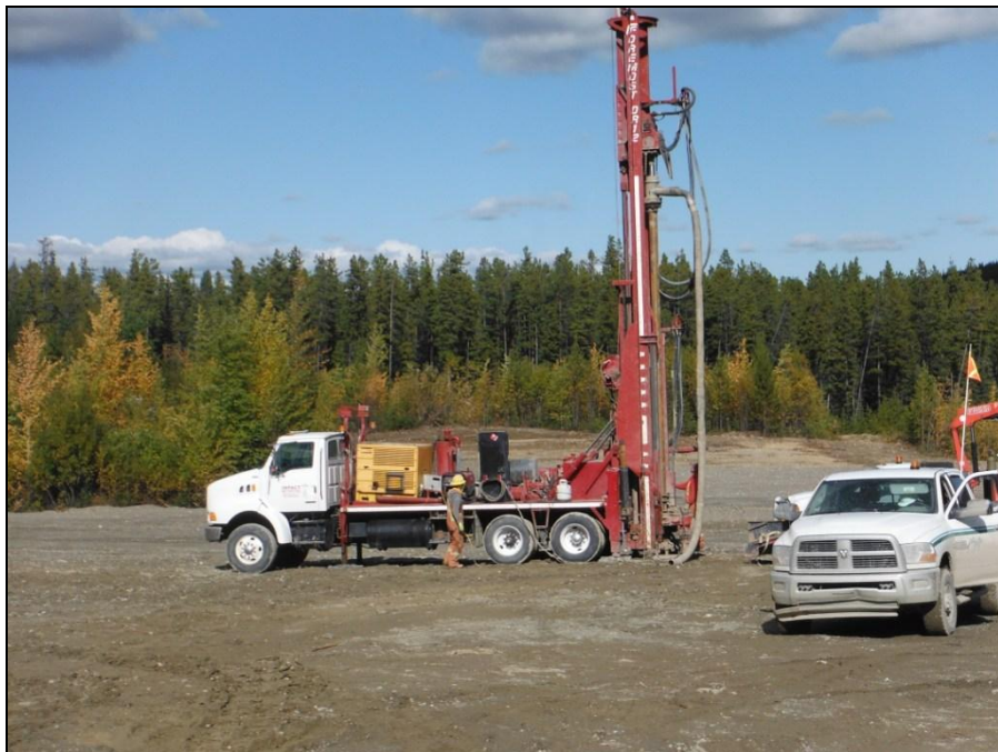
MISC Photograph 12: Golder Associates Ltd. overseeing installation of new groundwater monitoring well at landfill.
