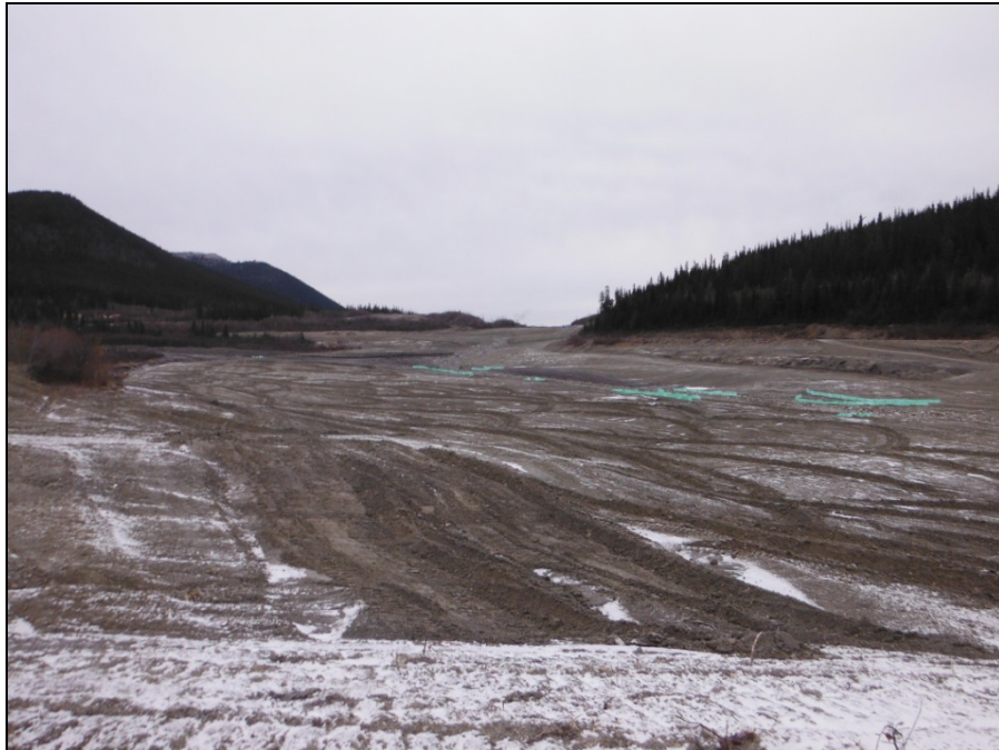
TMA Photograph 20: View from west abutment of former Reclaim Dam looking north toward capped Reclaim Pond, with sediment retaining structure in background.
