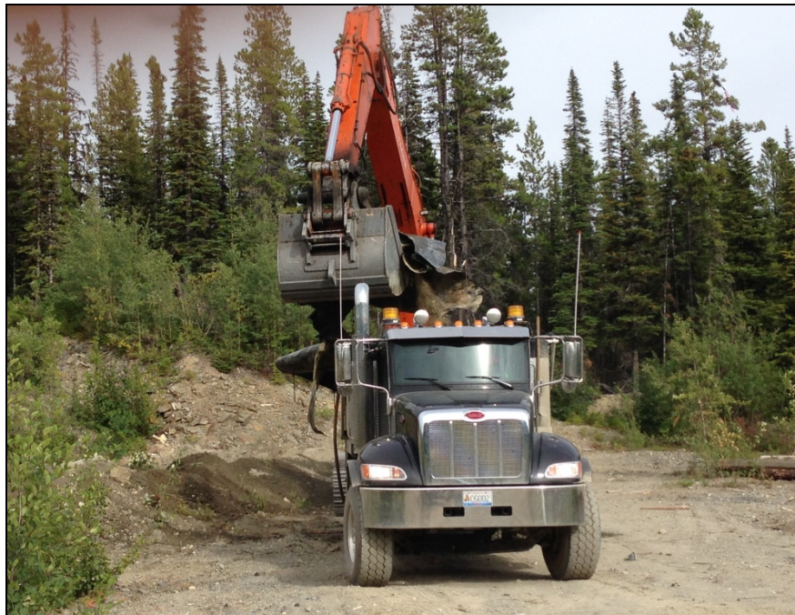
TANK Photograph 4: KPI loading tank containment berm liner into truck for transport to the Northern Environmental Services facility in Watson Lake.
