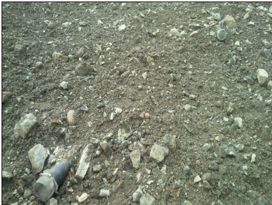
MTN Photograph 12: Sample Portal plug drainage pipes (top right and bottom left) at completion of reshaped waste rock dump material overtop of Portal plug.
