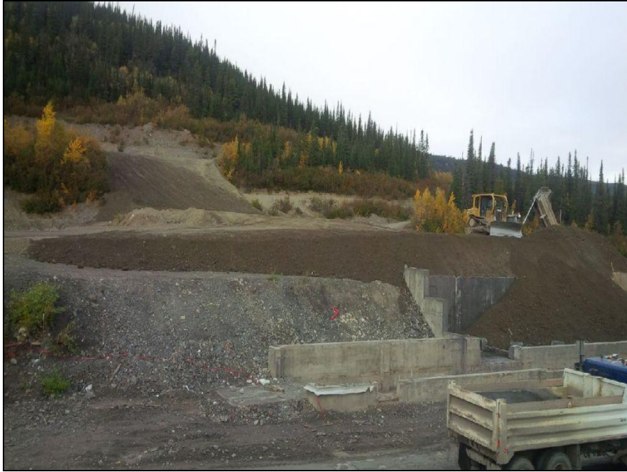
MISC Photograph 15: View of mill capping and shaping operations from east of former mill.
