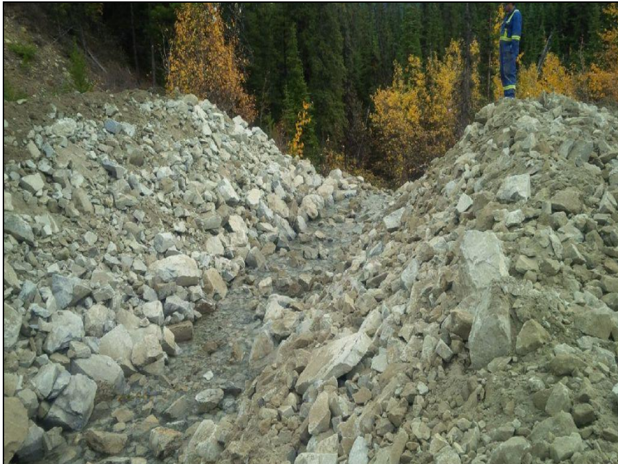
MISC Photograph 16: North Creek Dyke – construction of riprap lined channel through dyke at former culvert locations.
