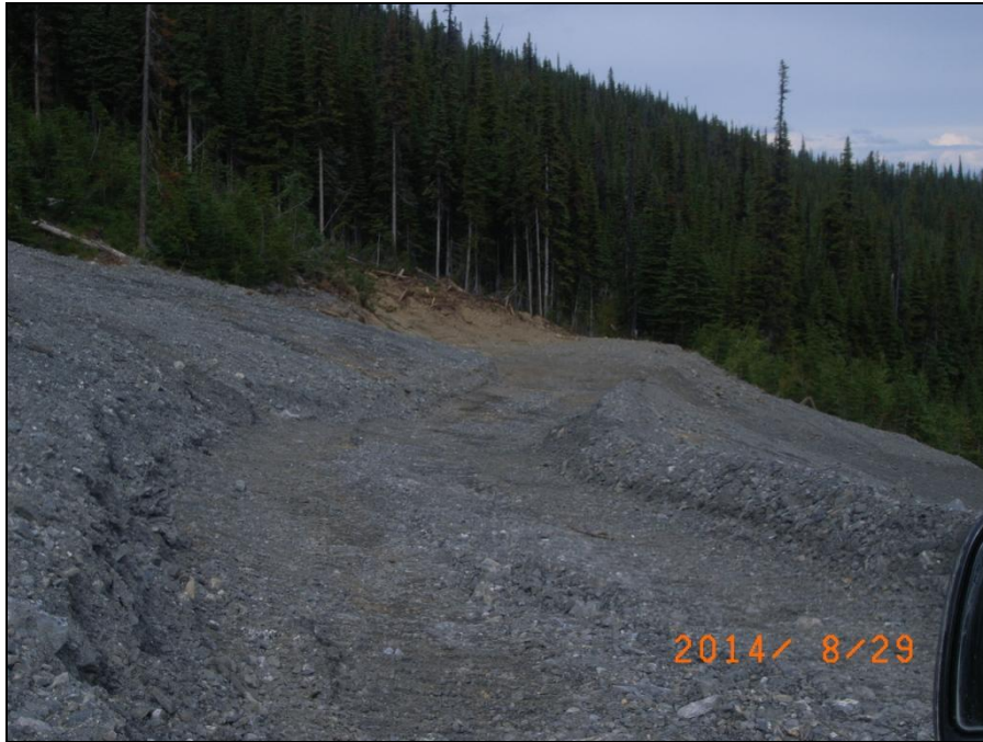
MTN Photograph 27: Helipad constructed at northern tip of Burnick 1200 waste rock dump.
