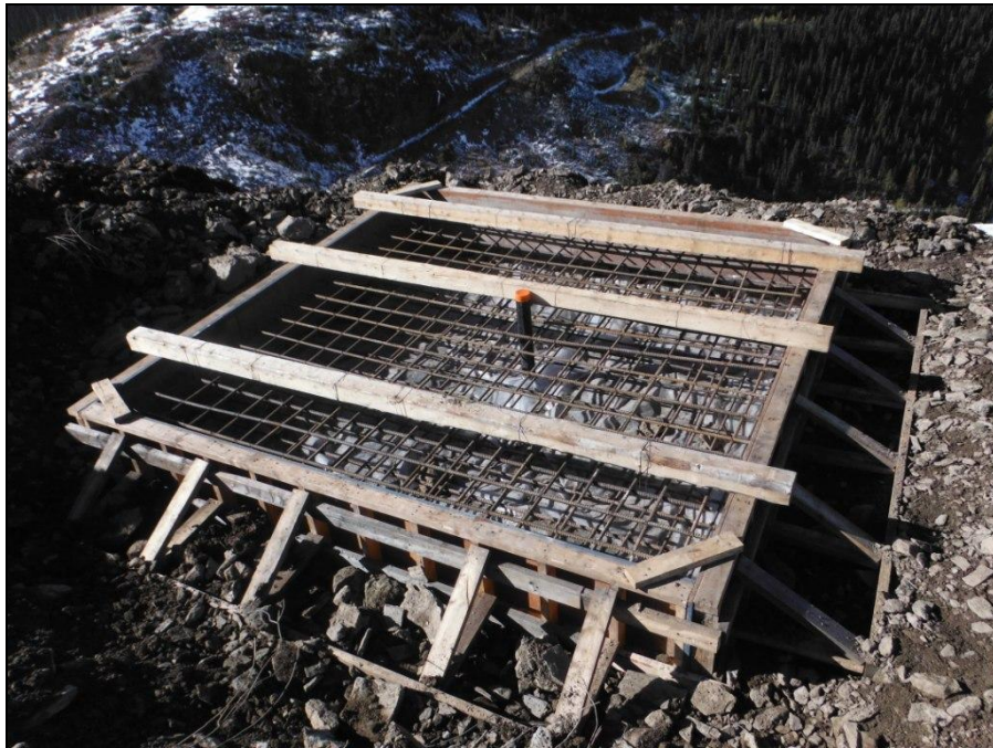
MTN Photograph 14: Formwork and reinforcing steel installed for construction of permanent cover over Jewelbox Summit Ventilation Raise.
