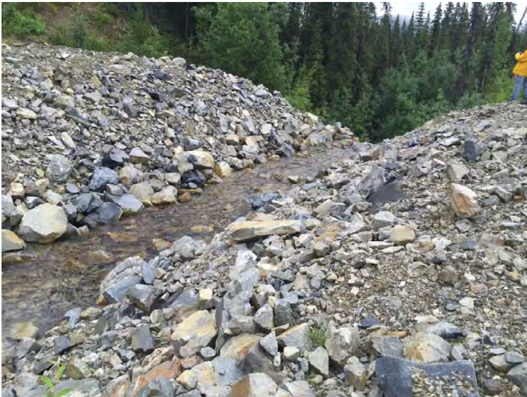
Photo 8: Ripped Section of North Creek at the Location of the Reclaimed North Creek Dyke
