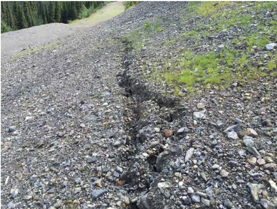
Photo 22: Subsidence Cracks due to Settlement of the Fill Placed over the 1200 Portal
