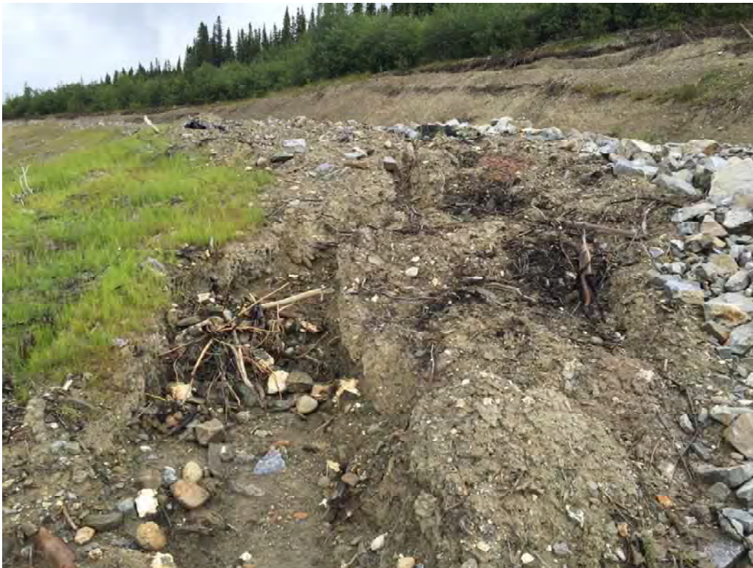
Photo 14: Subsidence Zone adjacent to the outlet of the North Channel
