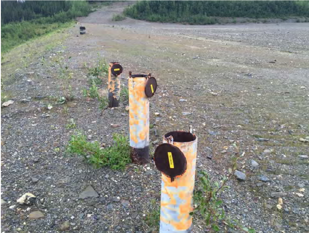
Photo 3: Protective Steel Caps for Piezometers NDM 3A and 3B, Settlement Gauge NDS 3
