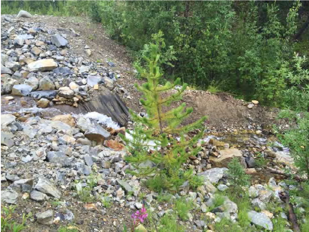
Photo 9: Exposed Fabric at the Outlet of the Riprapped Channel in North Creek
