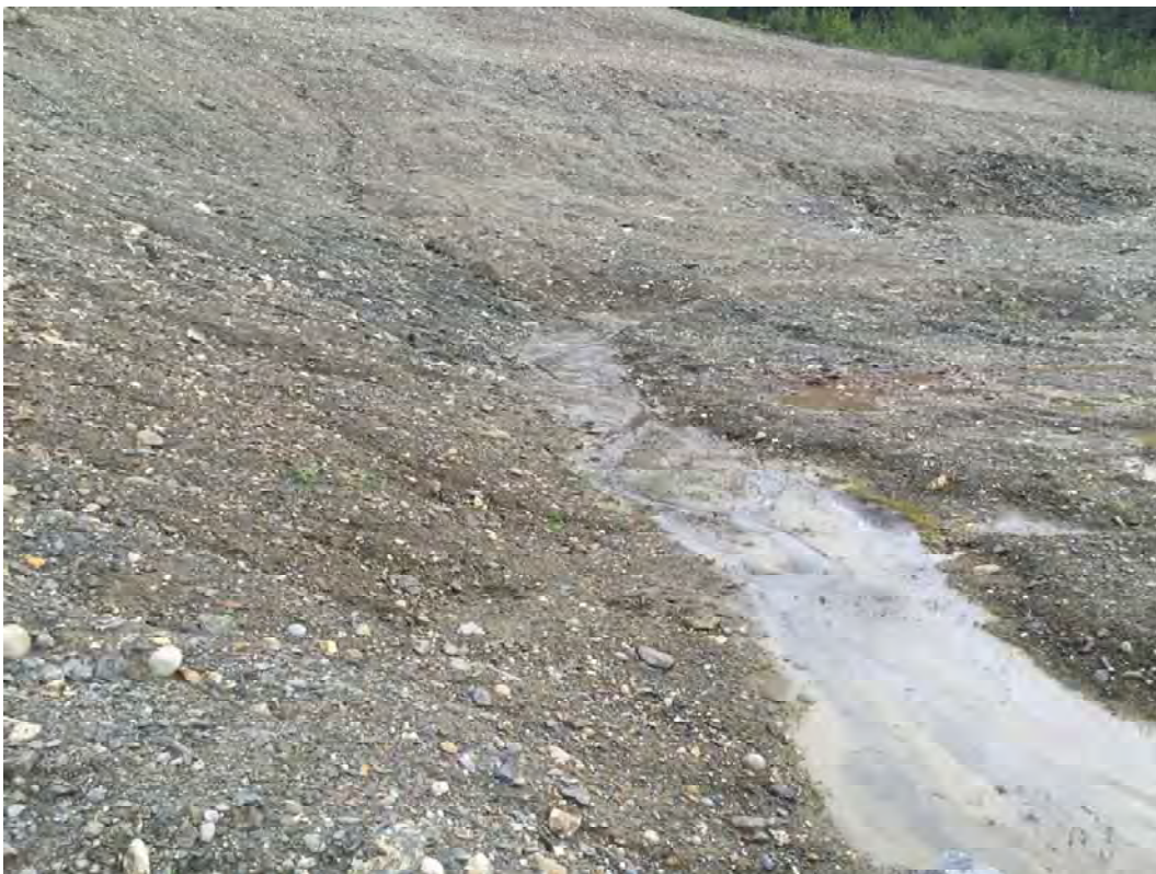
Photo 12: Seepage along Toe of the Sediment Retaining Structure from Hillside Springs
