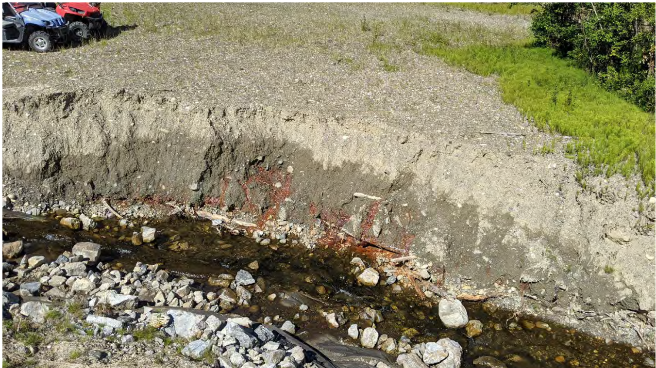
Photo NC-02: Channel Erosion at North Creek across the decommissioned access road to Burnick Zone. Seepage observed entering channel leaving a rusty-reddish coloured stain on the soils.
