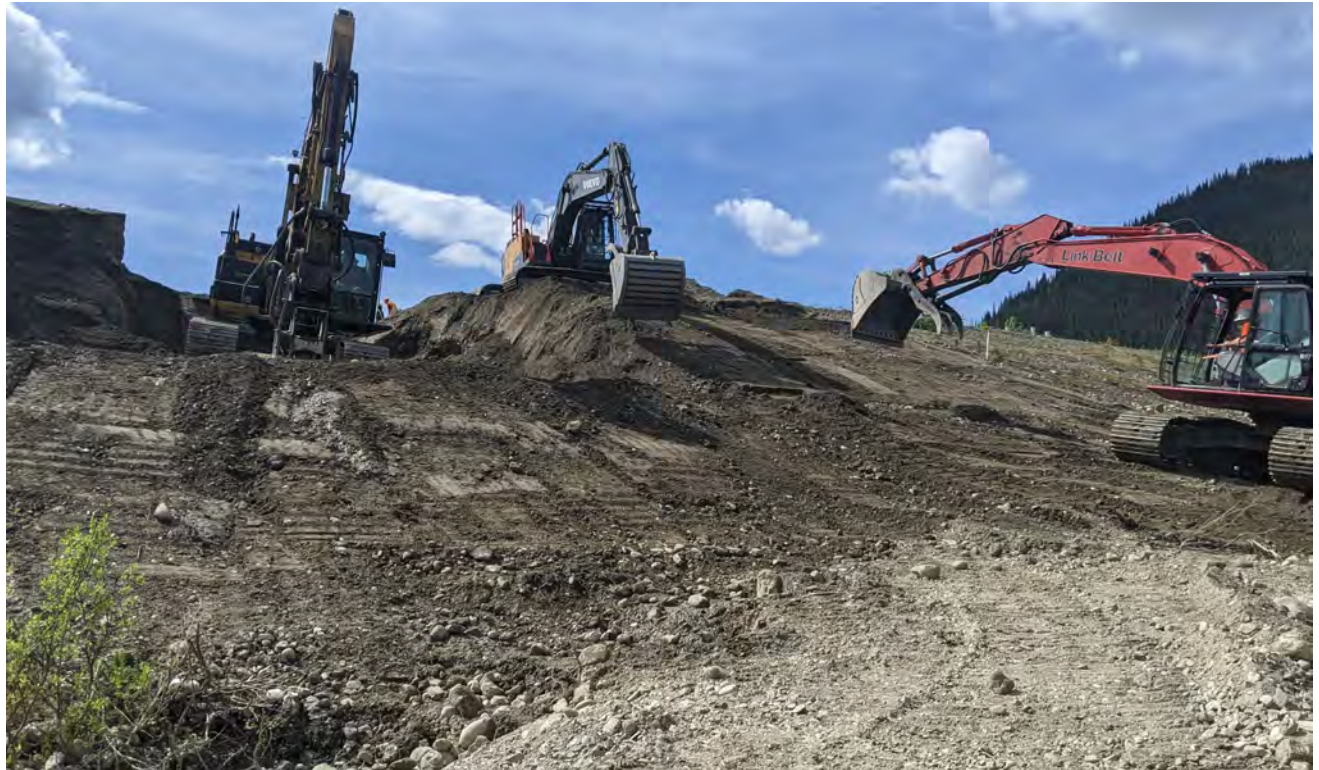
Photo 9: Placement of sand and gravel and trimming of the dam slope (June 25, 2022).
