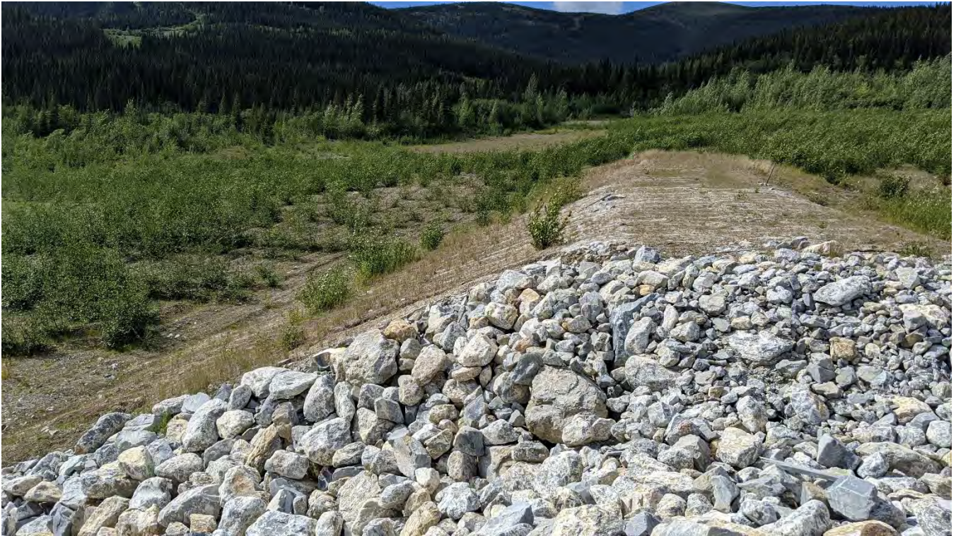
Photo SRS-03: Crest and downstream slope of the SRS looking west from the spillway.
