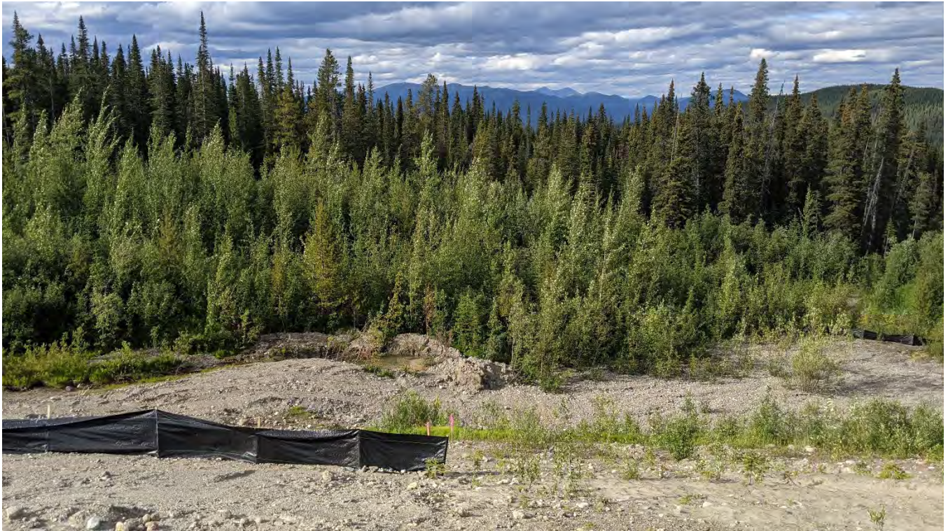
Photo ND-03: Erosion debris downstream of the dam. The silt fence is placed across the erosion gully repair area approximately midway down the slope. Historical wind-blown tailings visible to the right of the silt fence, further upslope.
