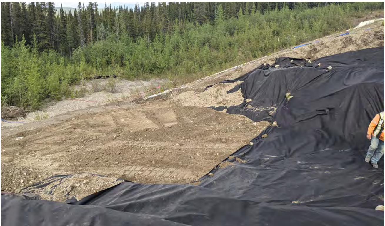
Photo 10: Geotextile installation to delineate between the Sand and Gravel and Repair Till embankment zones (June 25, 2022).
