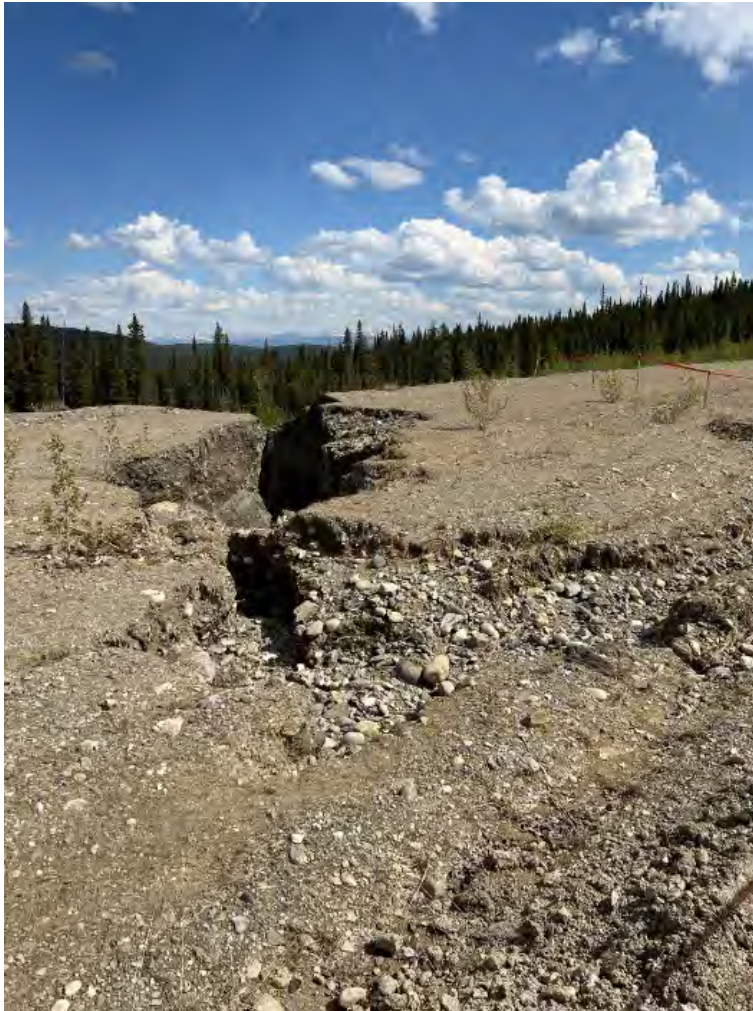
Photo 3: Erosion of the dam crest and tailings cover at the upstream end of the erosion gully (June 21, 2022).
