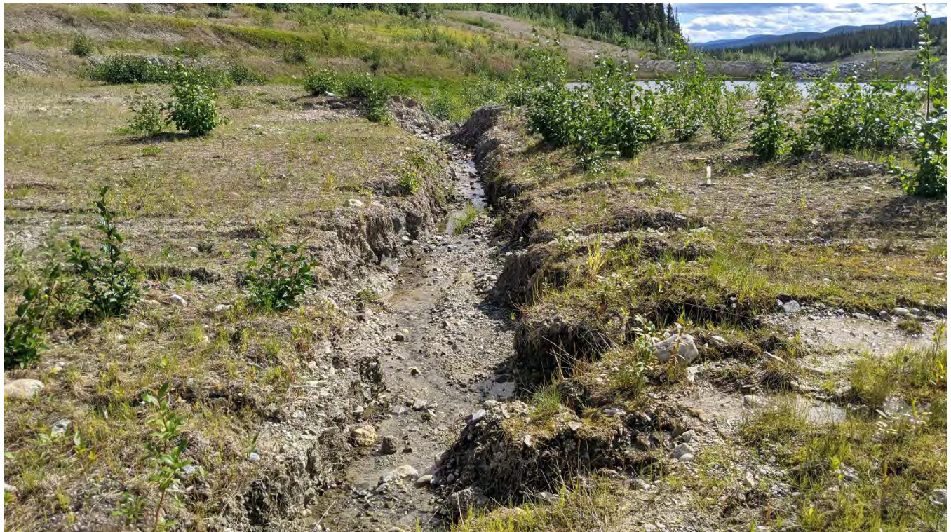
Photo TC-06: Erosion gully in tailings cover immediately to the south of the SRS Pond. Areas of exposed geotextile observed. No visible tailings observed.
