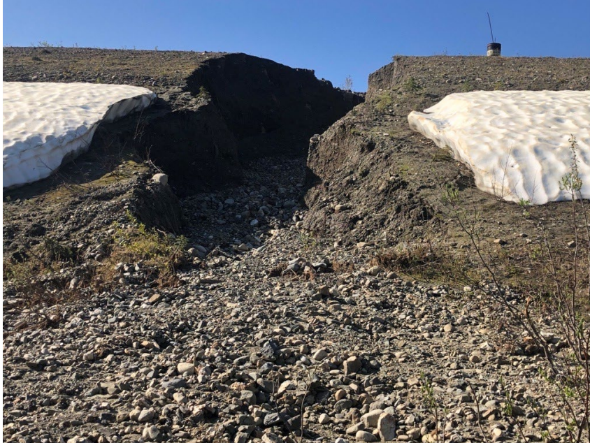
Photo 1. North Dam Erosion
