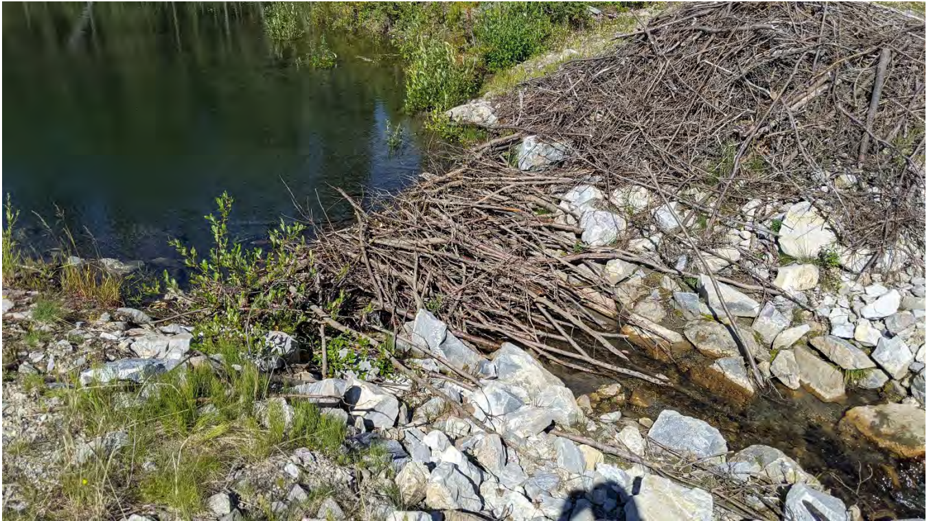
Photo NC-03: Beaver dam at the upstream end of the decommissioned North Creek Dike structure.
