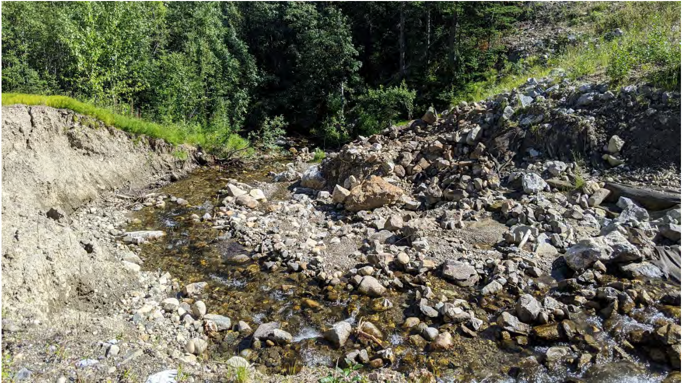
Photo NC-05: On-going channel and bank erosion at the downstream end of the lower decommissioned access road crossing of North Creek to the landfill area.
