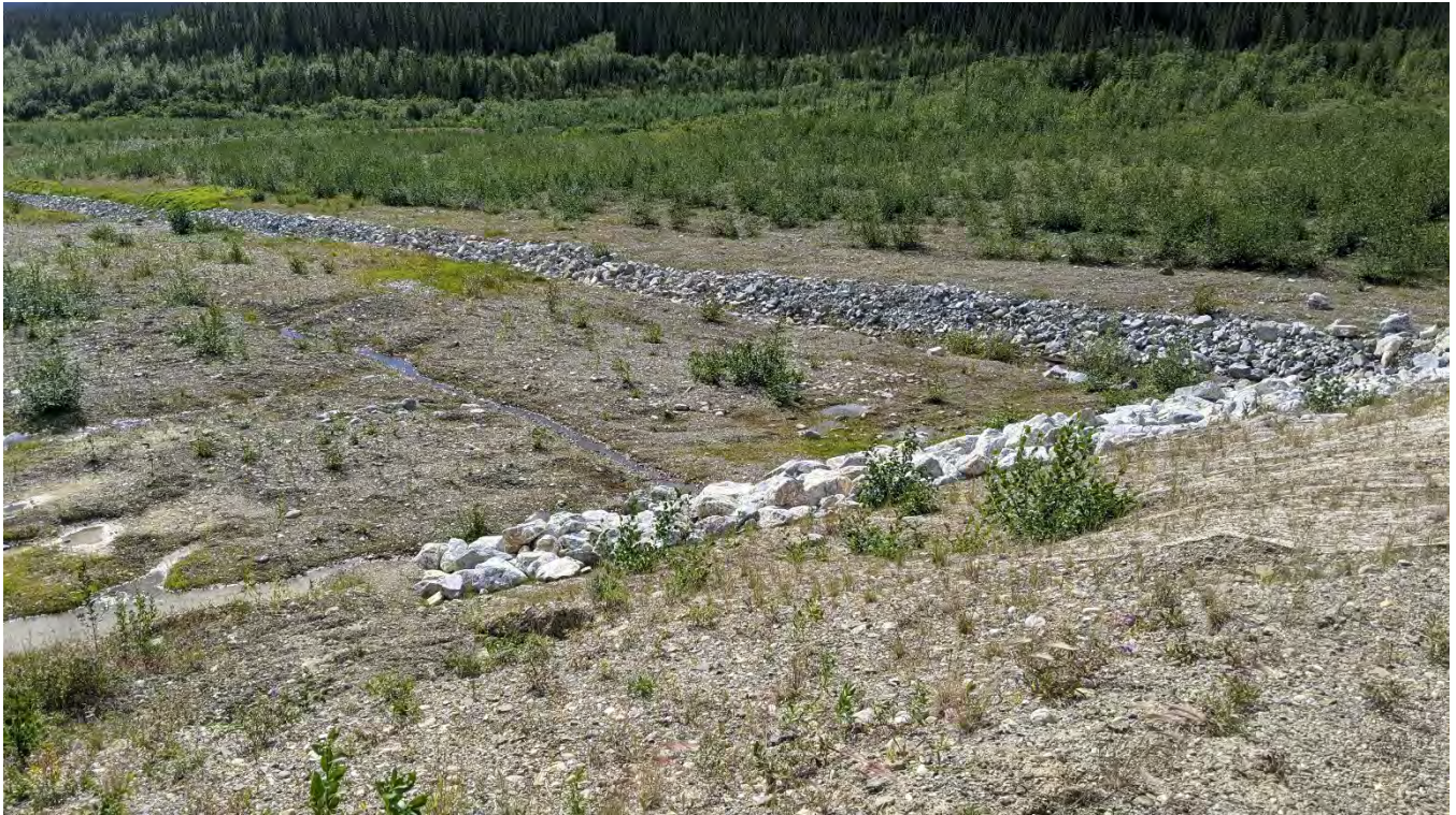
Photo SRS-05: Downstream face of the SRS on the east side of the spillway looking southwest.
