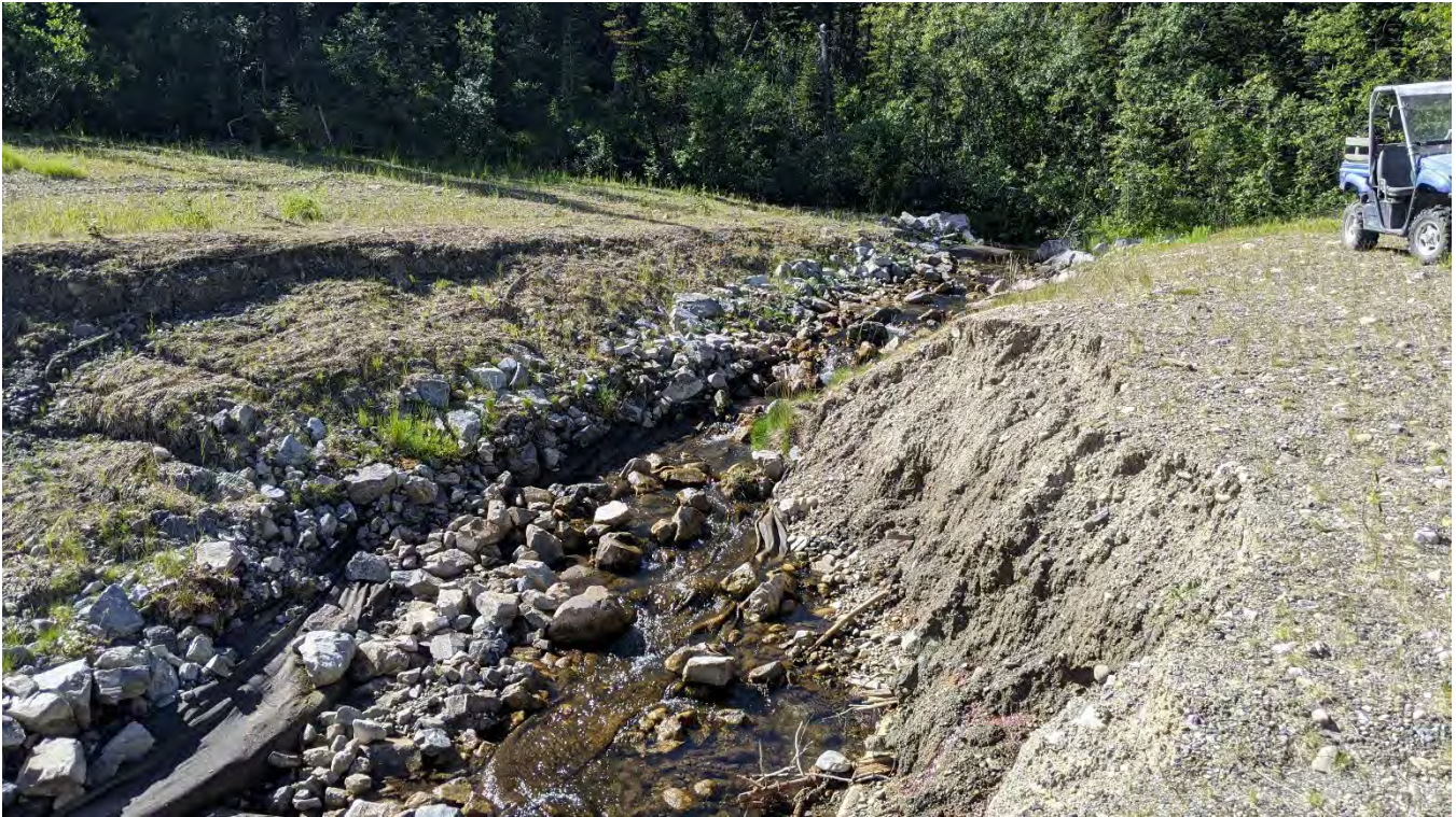
Photo NC-01: Channel Erosion at North Creek across the decommissioned access road to Burnick Zone.
