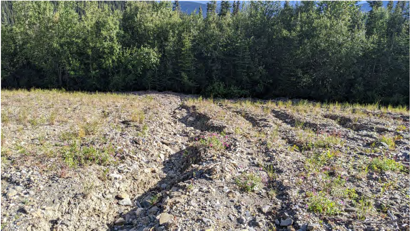
Photo WR-01: Rill and gully erosion across the decommissioned access road to the Jewelbox Waste Rock Dump.
