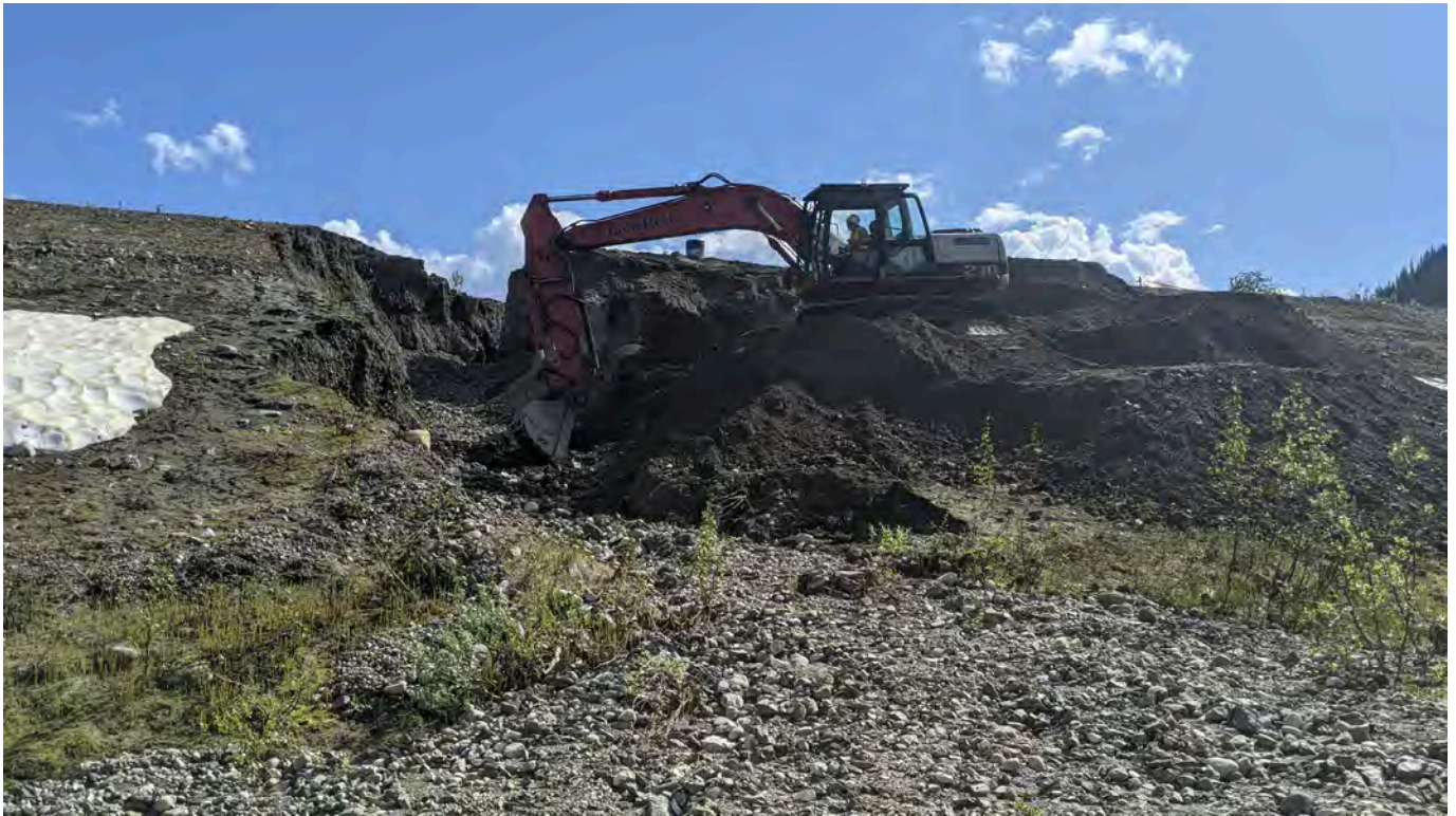
Photo 5: Excavator constructing working platforms down the west side of the gully (June 23, 2022).
