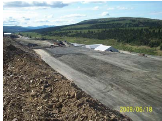
Photo 4: Looking down the cut slope at the Fuel Storage and Generator Pads.
