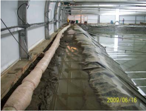
Photo 7: Looking at the liner key trench settlement along the perimeter of Sump 3.
