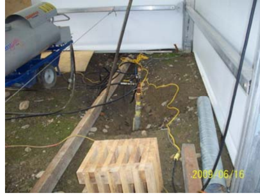
Photo 6: Looking at the NE corner of Sump 2 where there is noticeable settlement of the backfill over the buried propane line.
