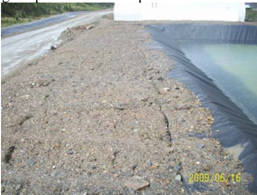
Photo 9: Notice the foot prints in the backfill material at Sump 4, which indicates that there was no compaction during placement.
