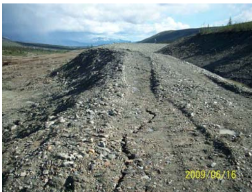
Photo 23: Looking south at the settlement cracks in the downslope fill portion of Ditch A.
