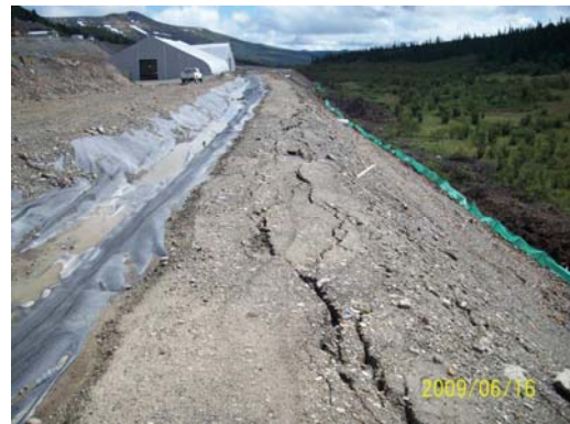
Photo 14: Looking SE at the tension crack along the downslope side of Collection Ditch 4.
