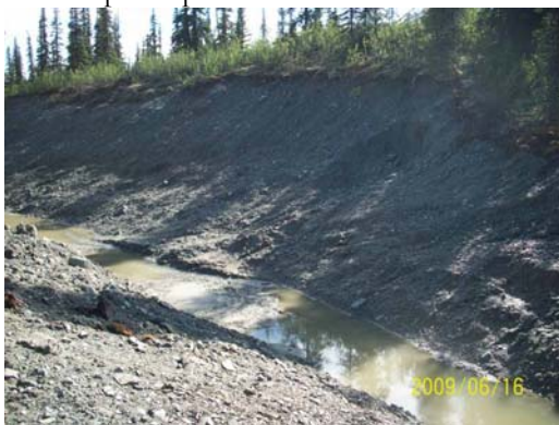
Photo 25: Looking SE at the cut slope of Ditch A. Notice the sloughing of the slope.
