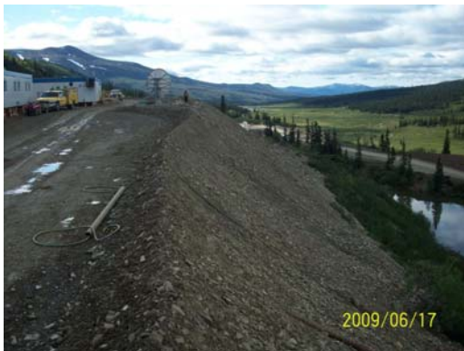
Photo 15: Looking SE from the NW corner of the Camp pad along the fill slope.
