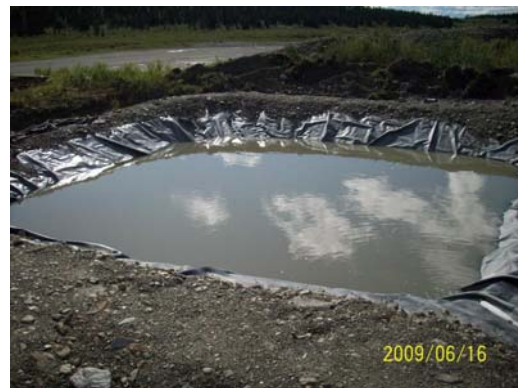
Photo 22: Looking west at the runoff collection sump that is located in the western corner of the LTF.
