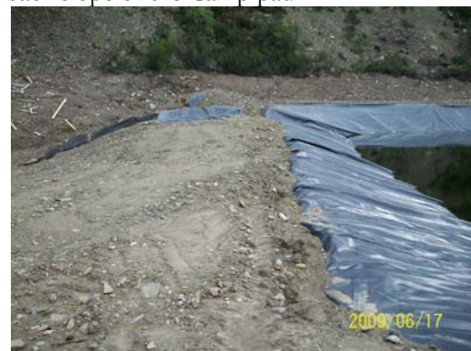
Photo 18: Looking at the settlement of the backfill material along the liner key trench of the treated effluent pond.
