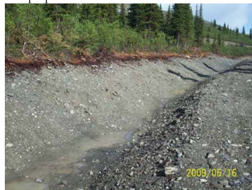
Photo 26: Looking SW at the cut slope of Ditch B at an area that is starting to slough.
