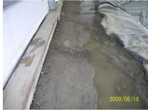
Photo 8: Looking at the seepage that is flowing in from beyond the perimeter of Sump 3's enclosure.
