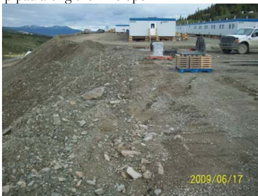
Photo 17: Looking NW along the south west portion of the Camp pad at the area where settlement cracks have formed after spring thaw.
