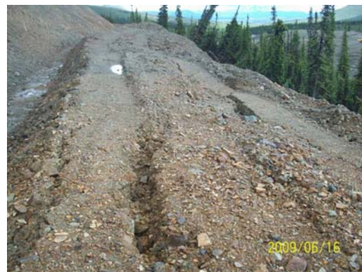
Photo 24: Looking SE at the settlement cracks in the downslope portion of the Ditch B.
