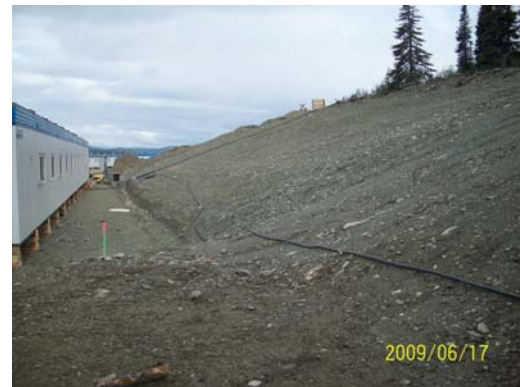
Photo 16: Looking NW from the SE corner along the back slope of the Camp pad.
