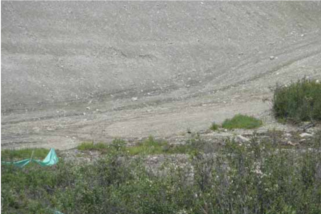
Photo 42 View of moist areas on downstream slope of dam – left abutment
