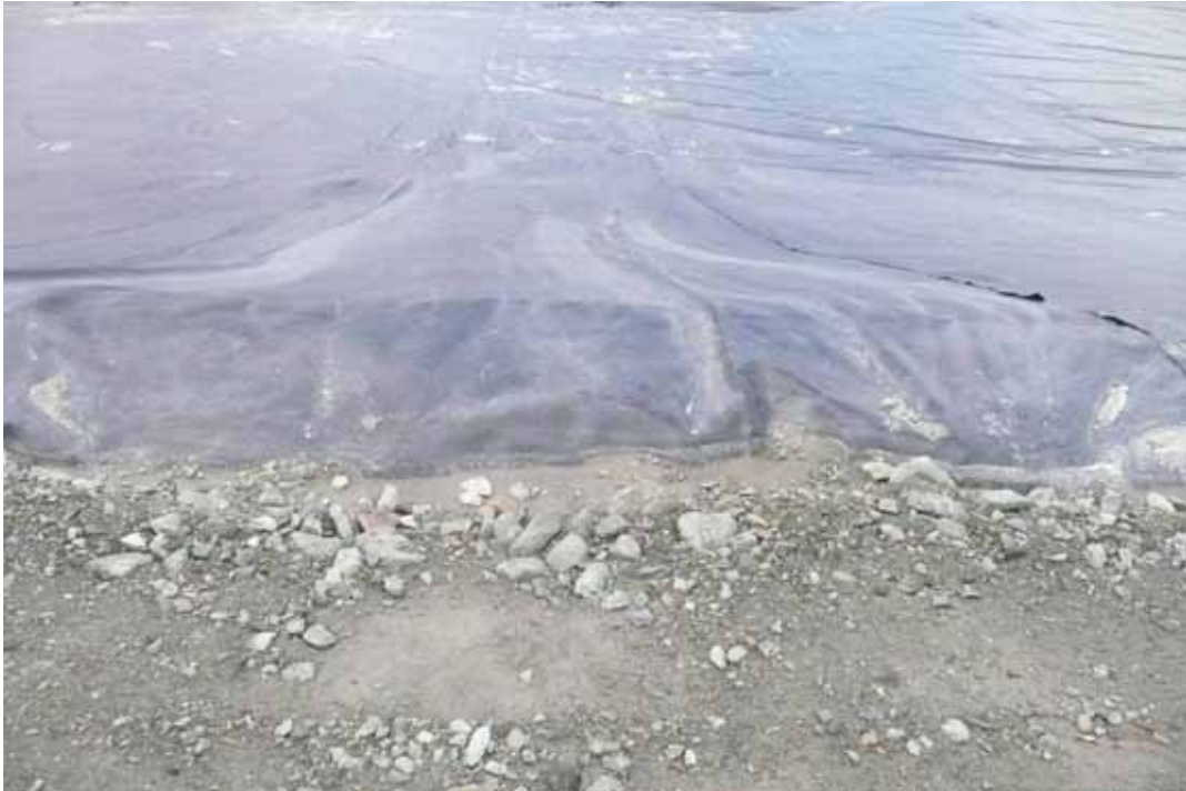
Photo 12 Minor slope slough under liner on the east side of the impoundment
