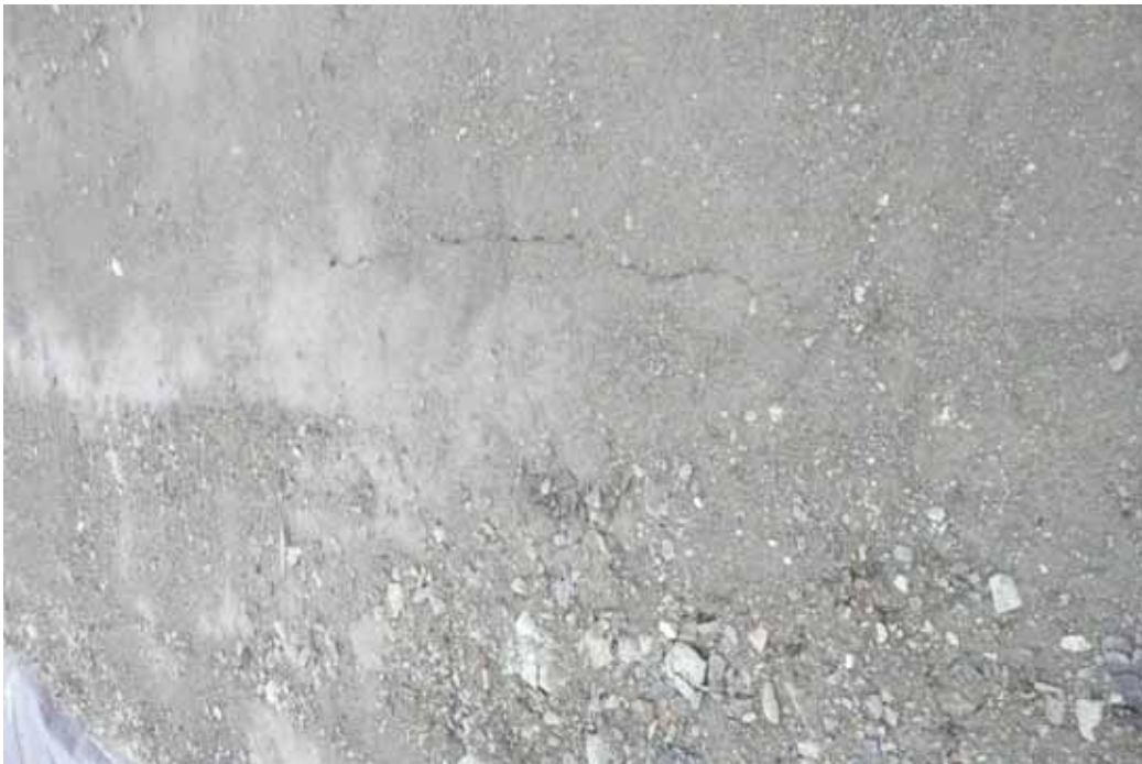
Photo 11 Minor settlement crack on perimeter road on the east side of the impoundment
