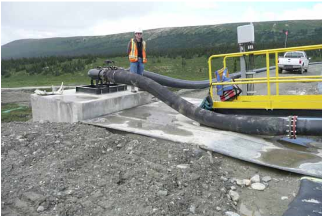
Photo 23 Anchor block for pump barge
