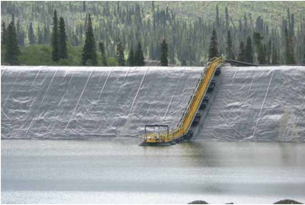
Photo 6 Reclaim pump barge
