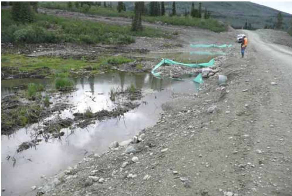
Photo 29 Seepage pond area – note culverts in road to be removed during construction of dam in August 2010
