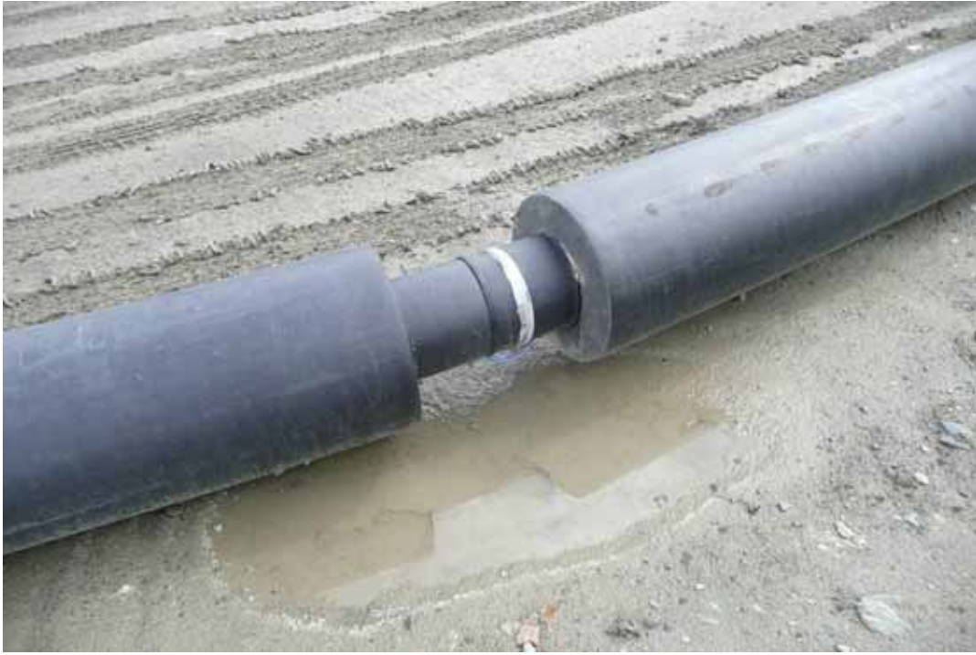
Photo 34 View of insulated tailings pipeline
