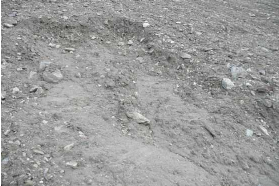
Photo 24 Moist area on left abutment of main dam
