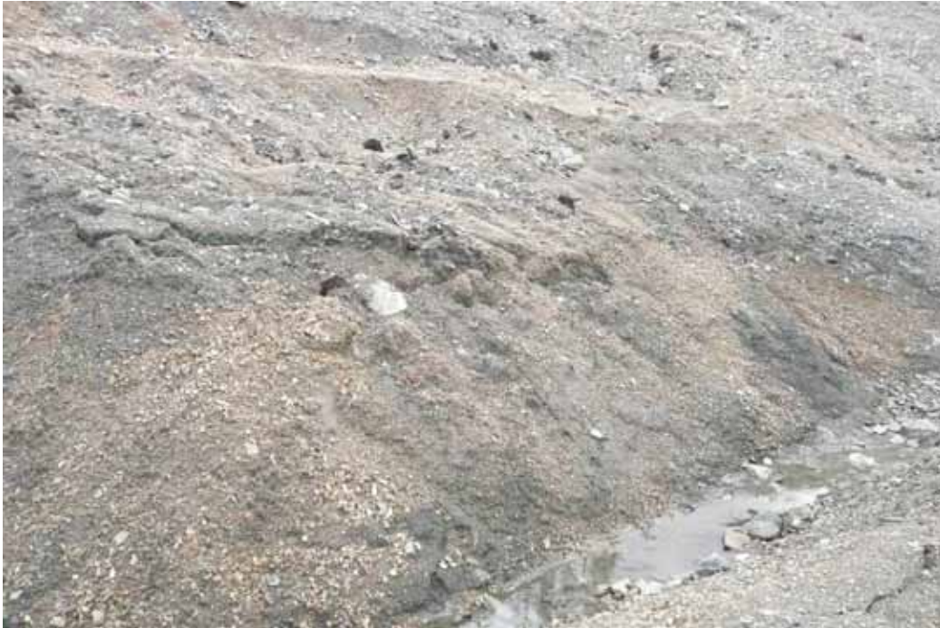
Photo 10 Inlet to the underdrain – flow from the upstream portion of Ditch B
