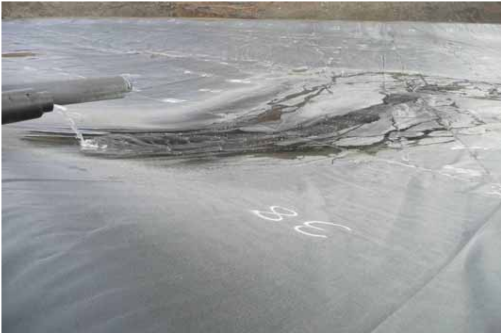
Photo 7 Tailings discharge pipeline (insulated pipes) (currently discharging mine water)
