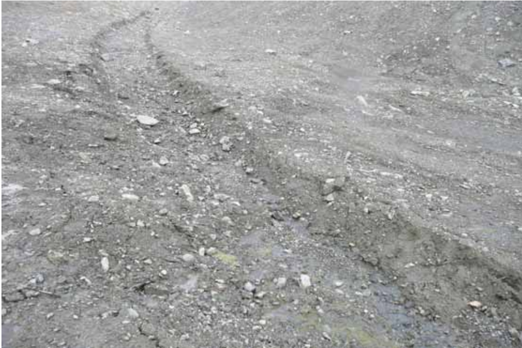
Photo 26 Seepage from low ridge near right abutment of dam - <1 L/s
