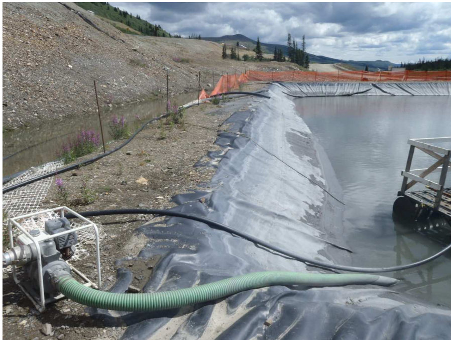
Photo 6 Sump 5 full of underground waste water. (July 9, 2013)
