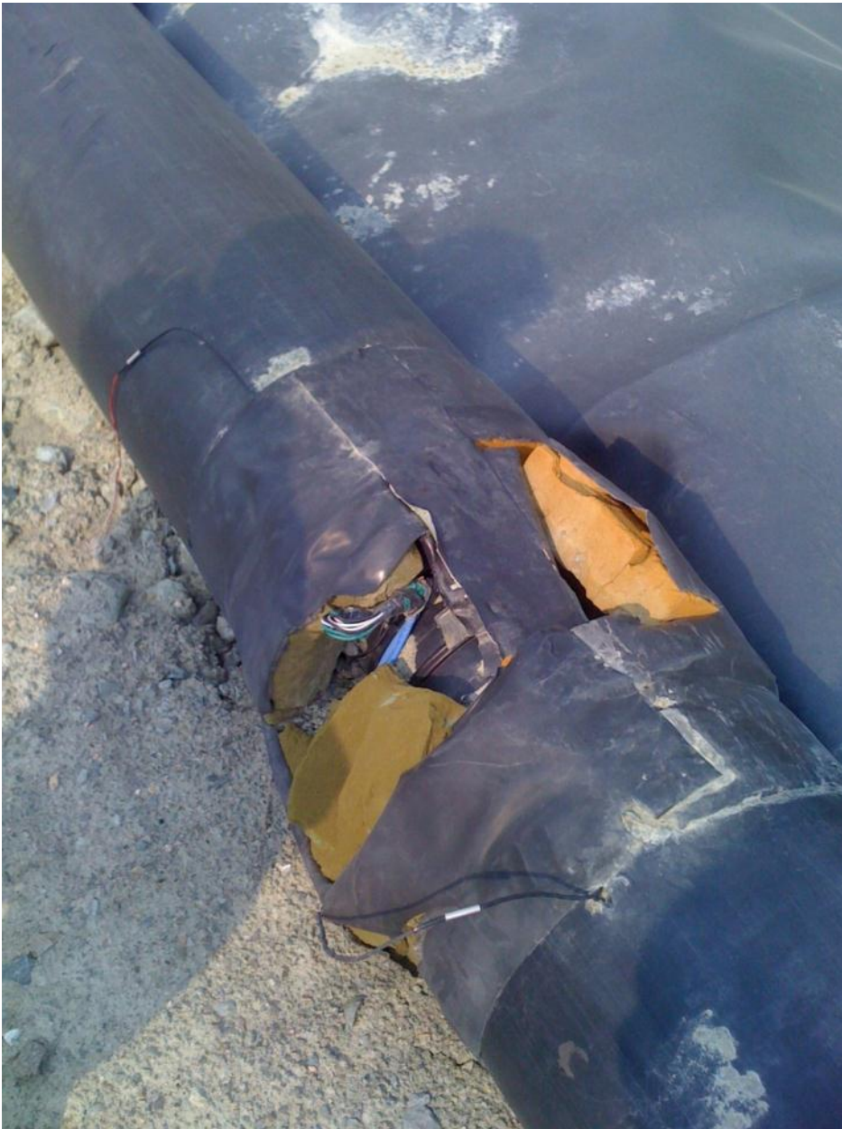
Photo 9 Reclaim line damage to outer insulating pipe wall following dam raise construction
