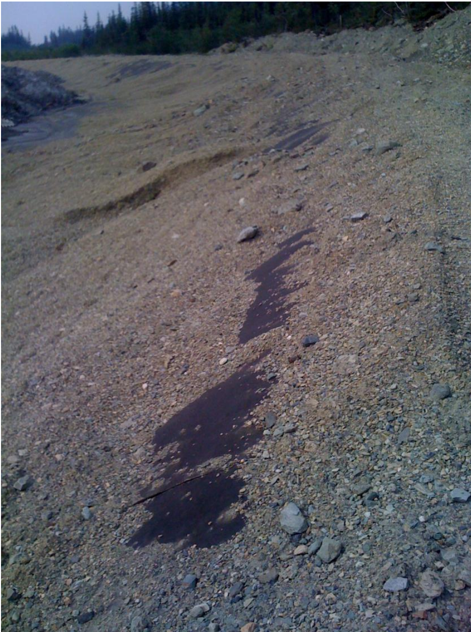
Photo 33 Waste Rock Stockpile – Service layer washed out
