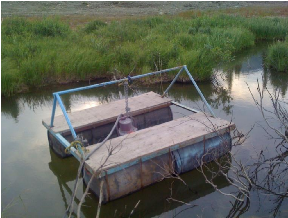
Photo 29 Seepage Return Pump
