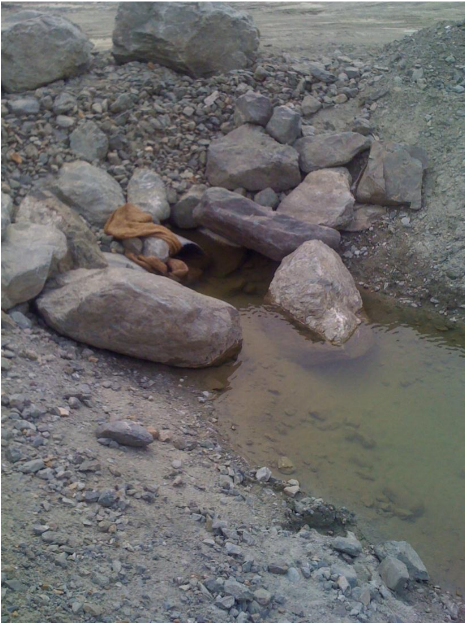
Photo 21 Ditch A culvert inlet partially blocked by coconut matting
