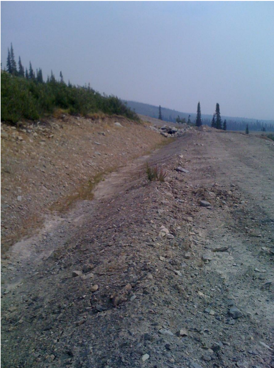
Photo 22 Ditch B –no flow
