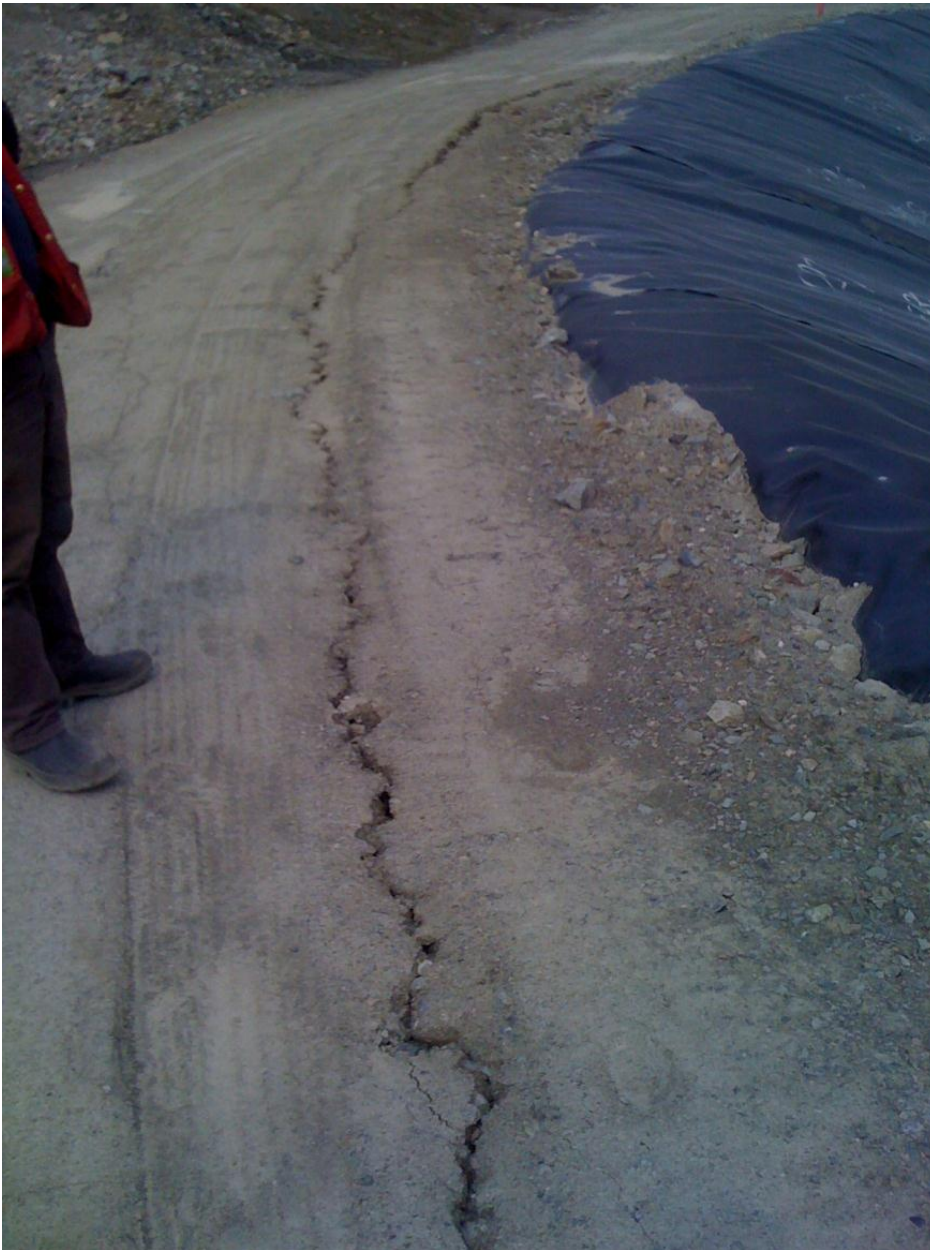
Photo 15 Cracks at north end of impoundment on crest
