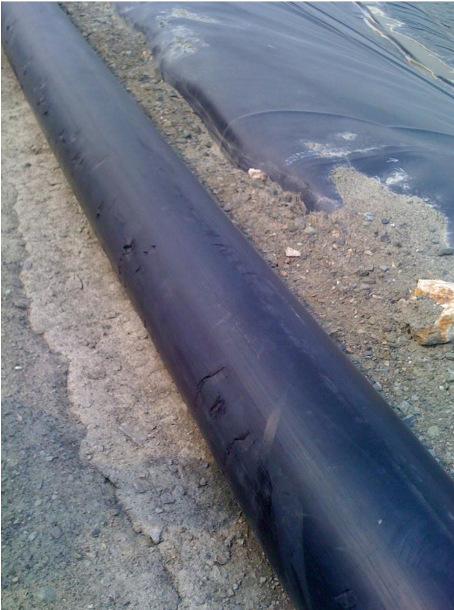
Photo 3 Minor cracking around reclaim line
