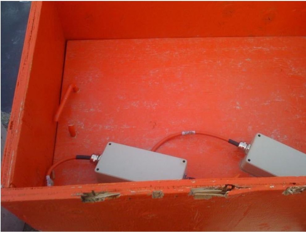
Photo 6 Piezometer data collection box
