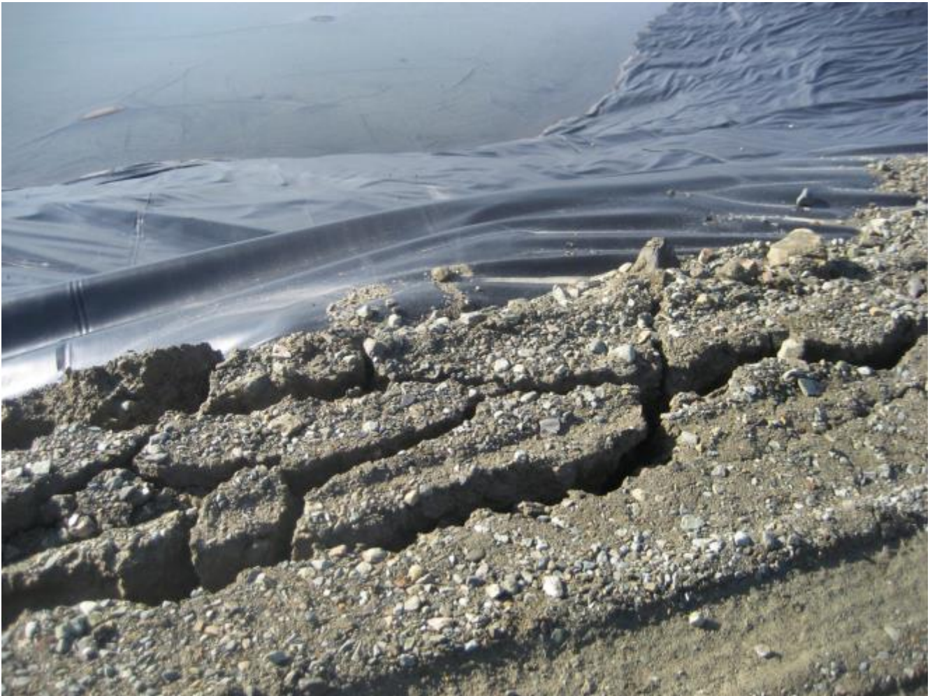
Photo 24 Cracks at north end of impoundment on crest
