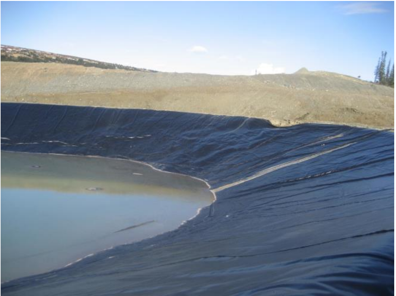
Photo 25 Slumping in north end of impoundment
