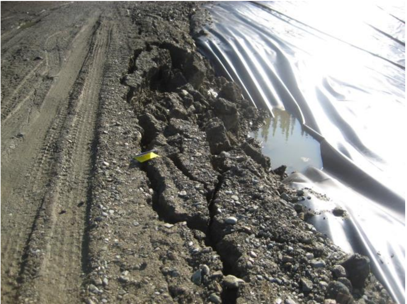
Photo 26 Cracks around slumping area
