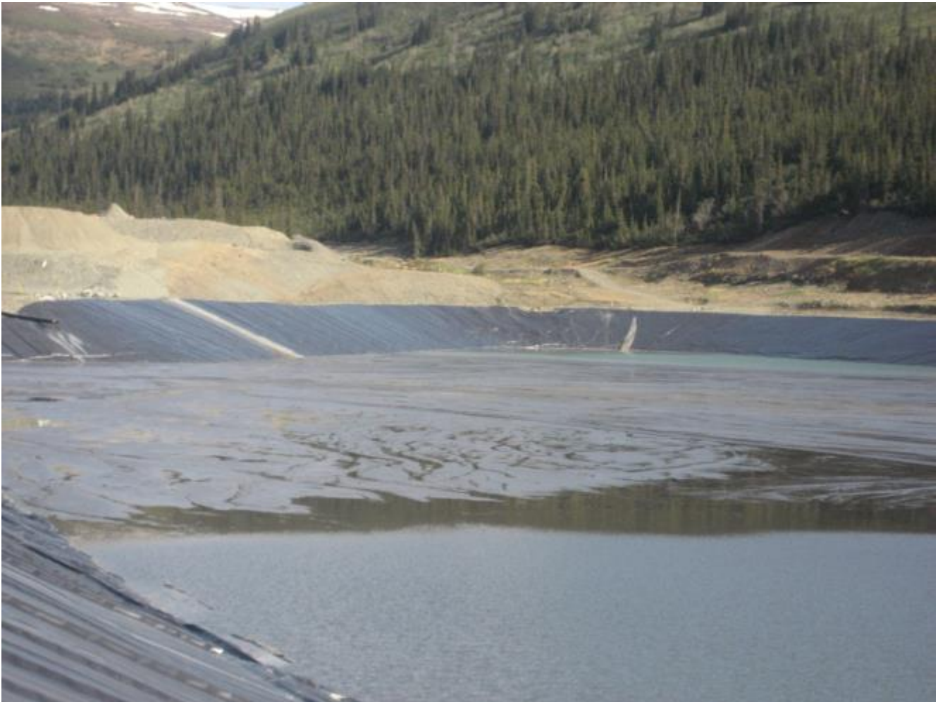
Photo 27 Slump at north end of impoundment from dam
