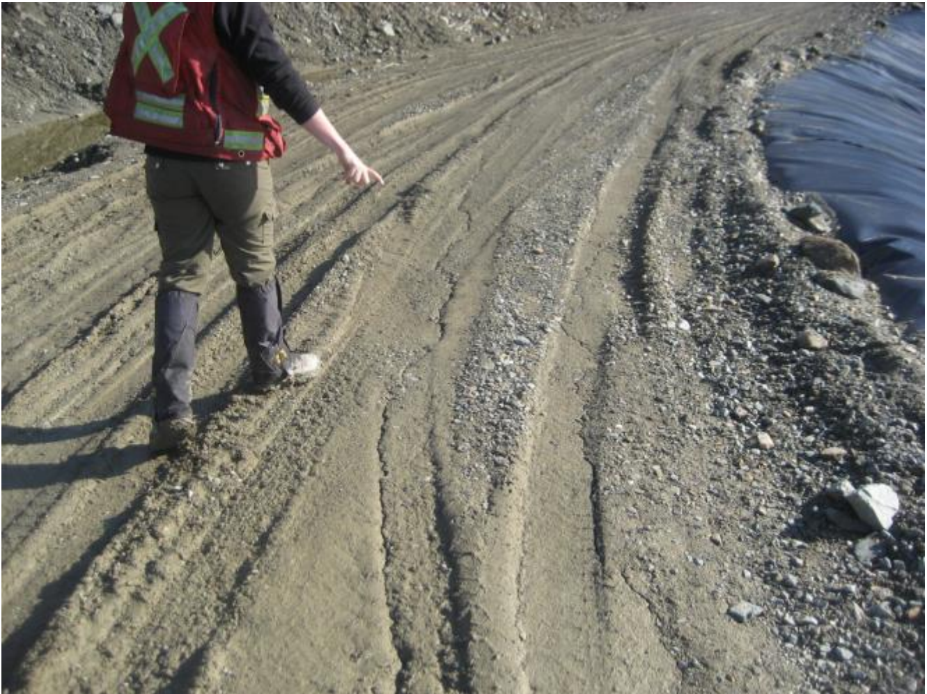
Photo 23 Cracks at North End of impoundment
