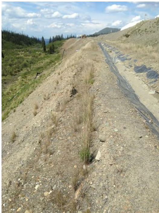
Photo 15 Vegetation growth throughout the tension cracks, areas of settlement and erosion channels. (June 24, 2014)
