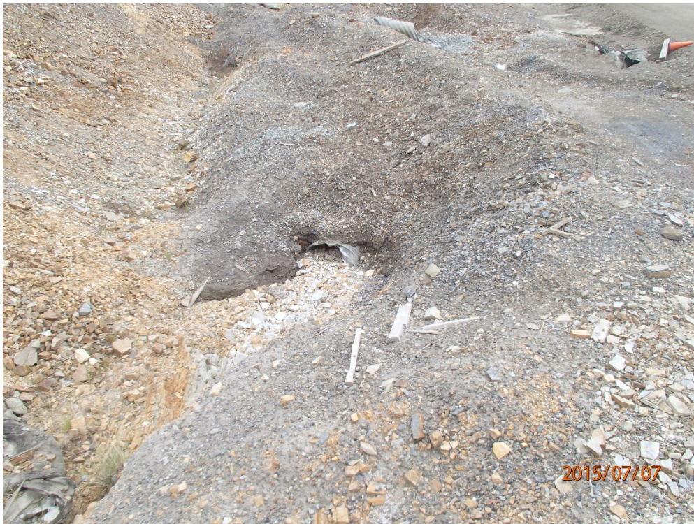
Photo 17 Ditch 1- culvert inlet completely blocked
