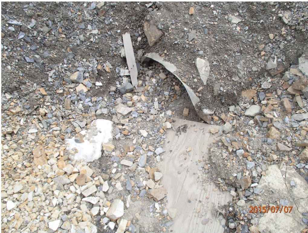
Photo 19 Ditch 2 – inlet for upper culvert, completely plugged, non-functional
