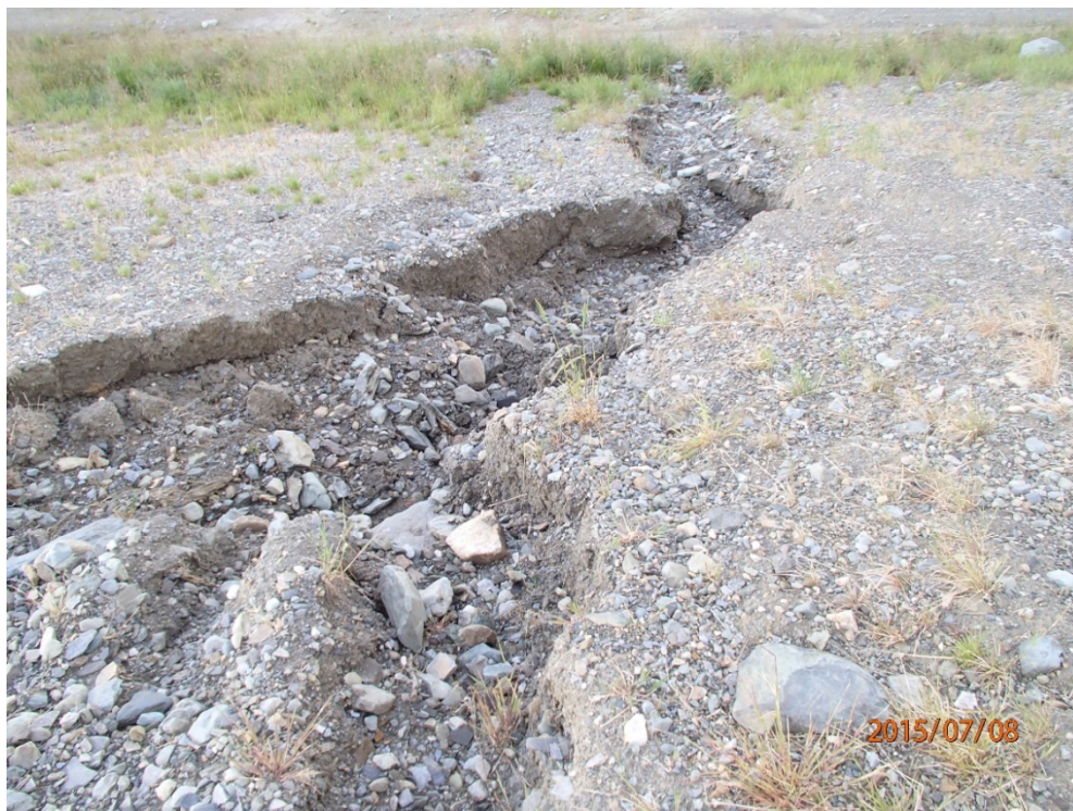
Photo 41 Northwest waste pile – erosion gully at the slope by the air strip
