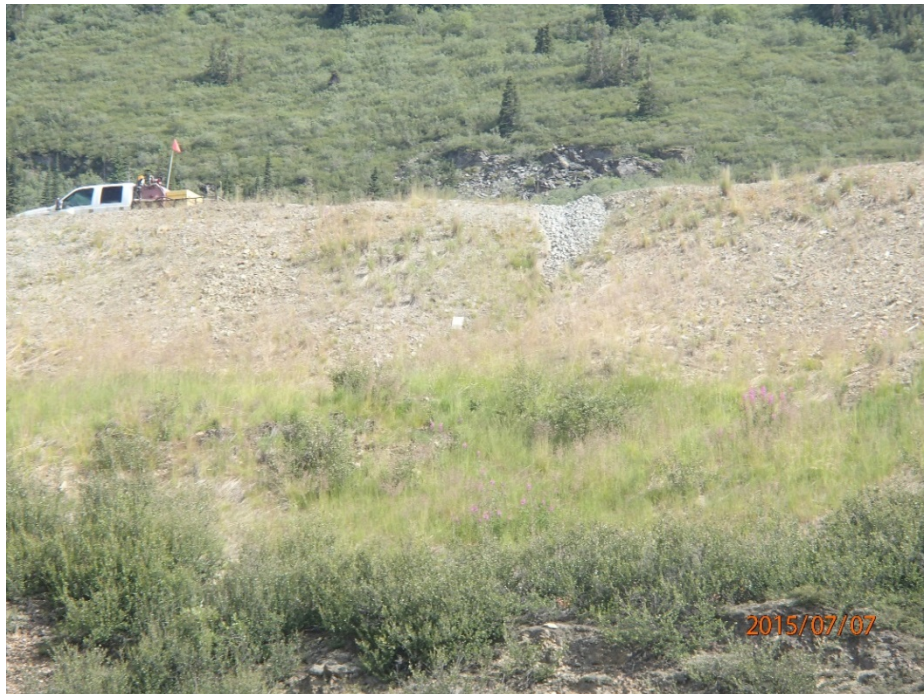
Photo 35 Camp pad – erosion channel in cut slope in south wall, partially backfilled with rock (centre part)
