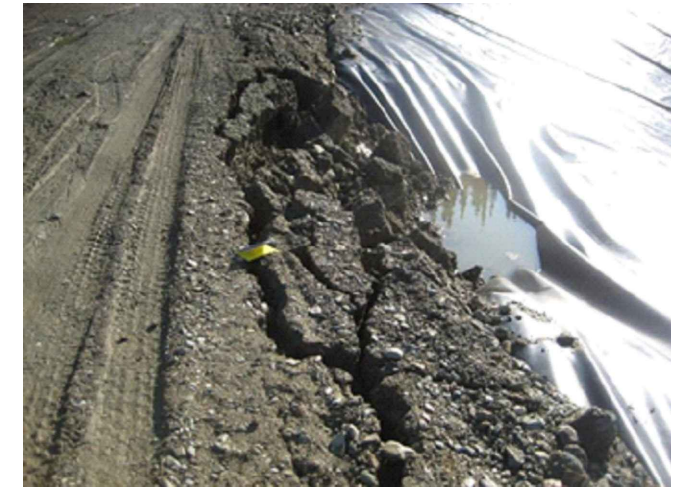
2014: CRACKS AROUND SLUMPING AREA
