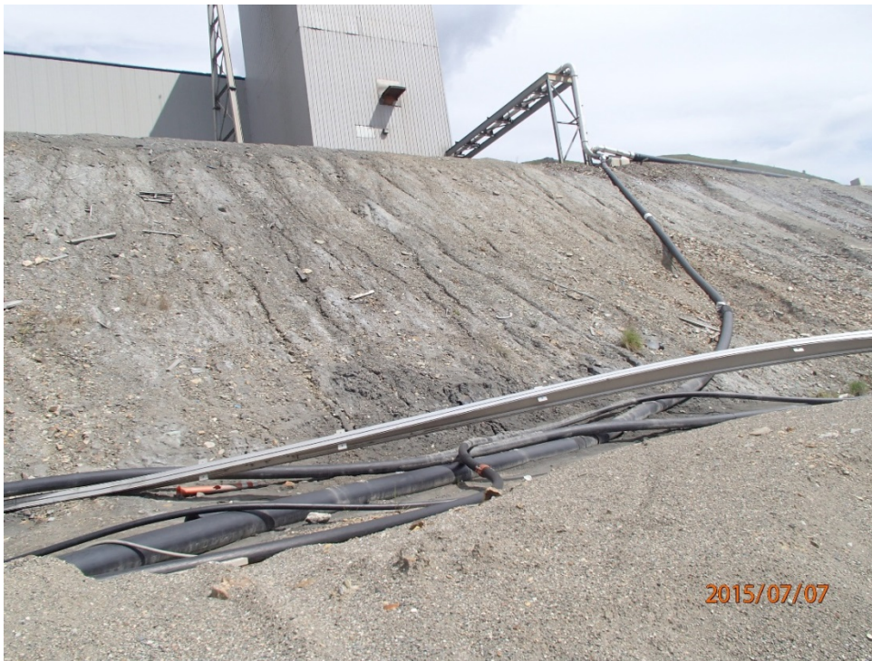
Photo 2 Mill building – downslope, minor erosion
