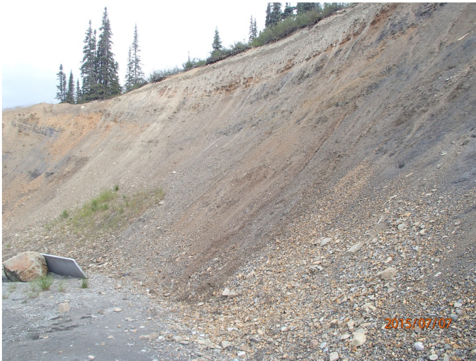
Photo 48 Vent Raise and Underground Mine Office – back slope, very steep cut slope, minor signs of erosion, crest of the slope not checked
