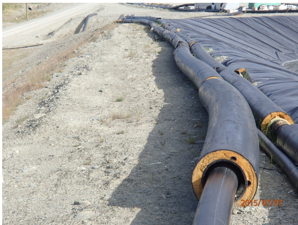
Photo 6 West dam crest - looking north between access ramp and spillway, tailings line and reclaim line
