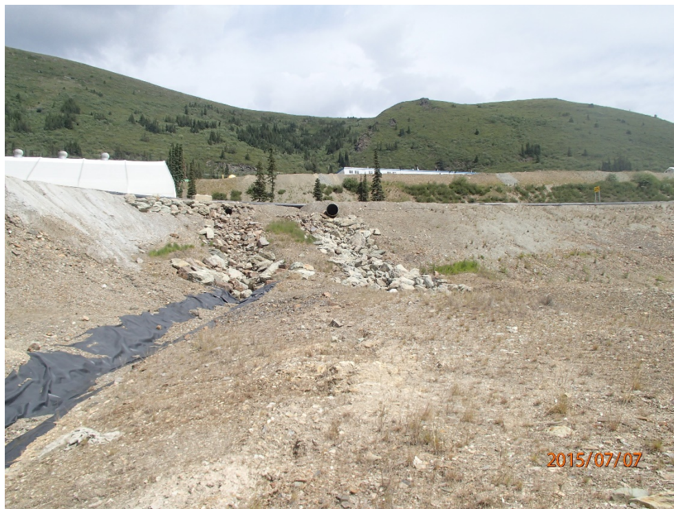
Photo 20 Ditch 2 – rip-rapped outlet for upper culvert on the left; gravel swale for groundwater culvert and Ditch 1 outlets on the right
