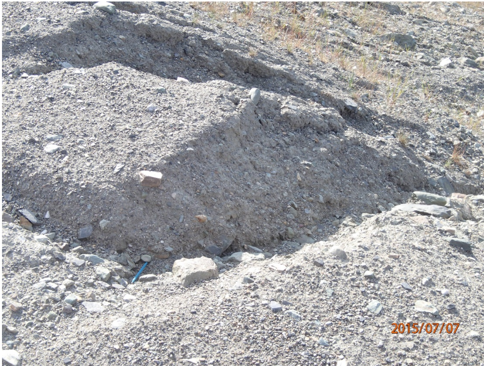
Photo 2 South dam –erosion gully on downstream edge
