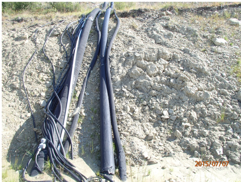
Photo 38 Upper generator and potable water treatment pad – cut slope, slumping along the water line corridor
