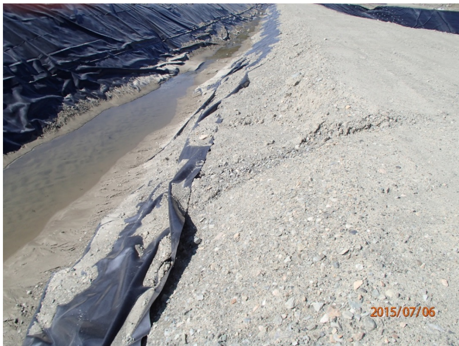
Photo 28 Ditch A – lined part – no anchoring of geotextile
