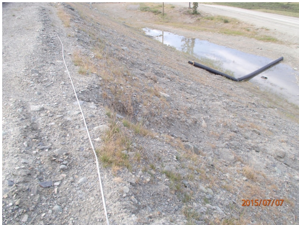
Photo 7 West dam – erosion on downstream slope north of the access ramp, 10 m wide area; crest width is approximately 4 m
