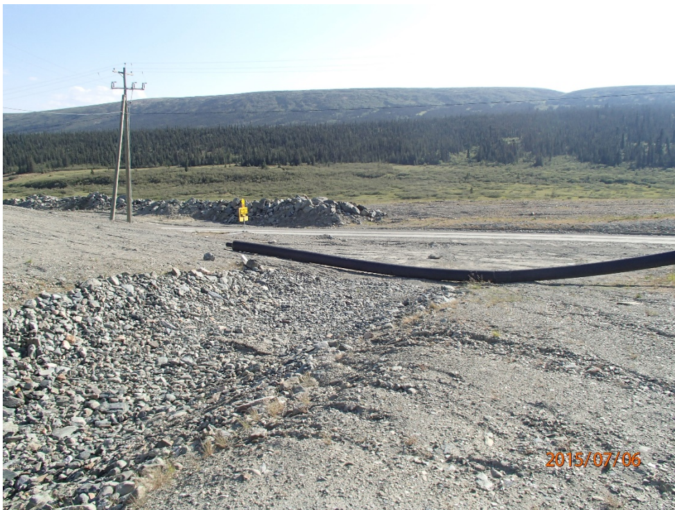
Photo 17 Spillway –looking downstream- rip rap ends upstream of the haul road and 12 inch redundant tailings line blocking the spillway
