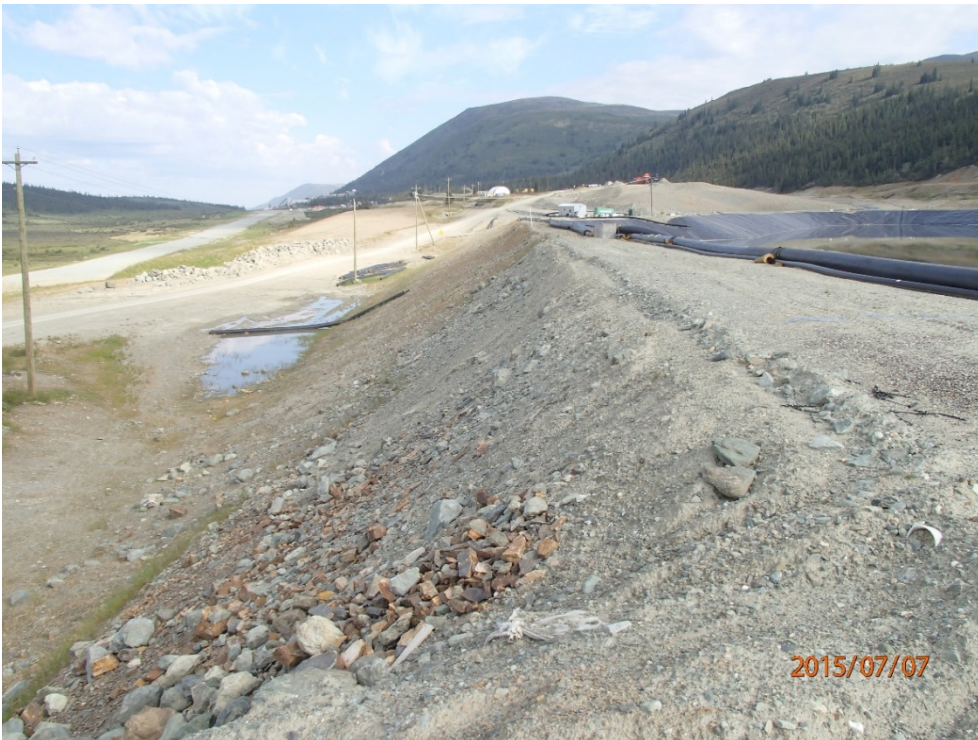
Photo 9 West dam – downstream slope, looking north, north of access ramp, ponded rain water at the toe
