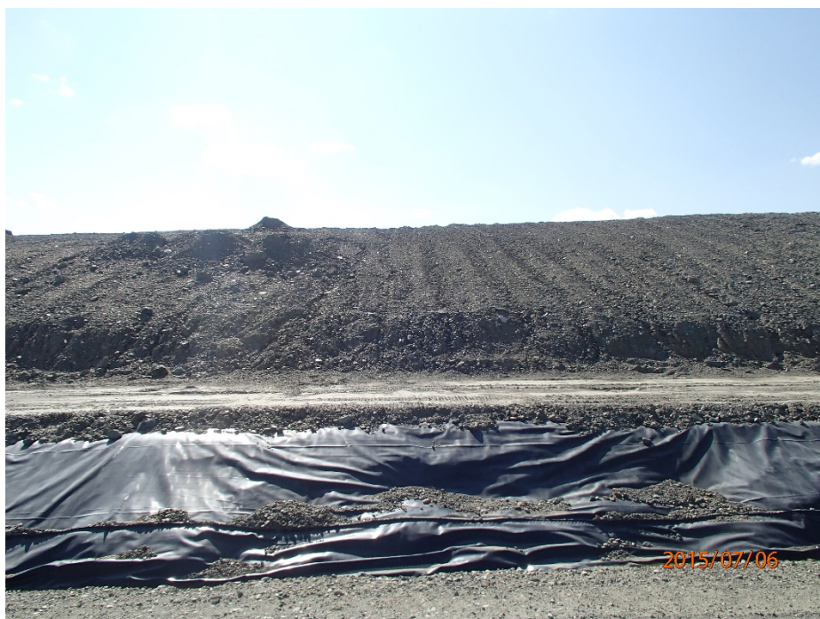
Photo 29 Fill slope upstream of Ditch A – graded in 2014, signs of erosion
