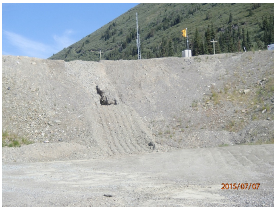
Photo 32 Camp Pad – large erosion channel in cut slope east wall, partially filled with rock, surface runoff from camp pad area accumulates at low point and drain through this area
