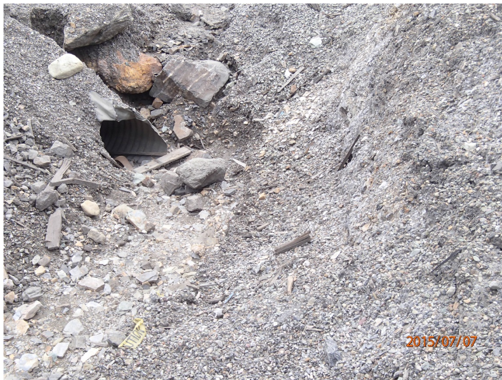
Photo 31 Ditch 5 – culvert inlet, channel bottom filled in and partially blocked with litter
