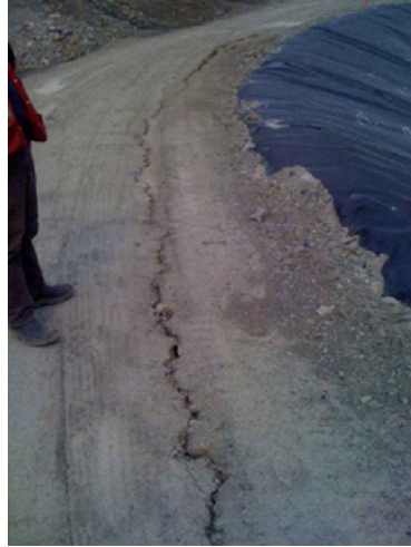
2013: CRACKS AT NORTH END OF IMPOUNDMENT ON CREST
