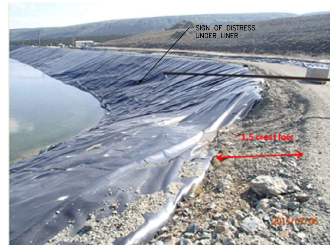
2015: CREST LOSS ALONG THE 2014 SLUMP AREA
