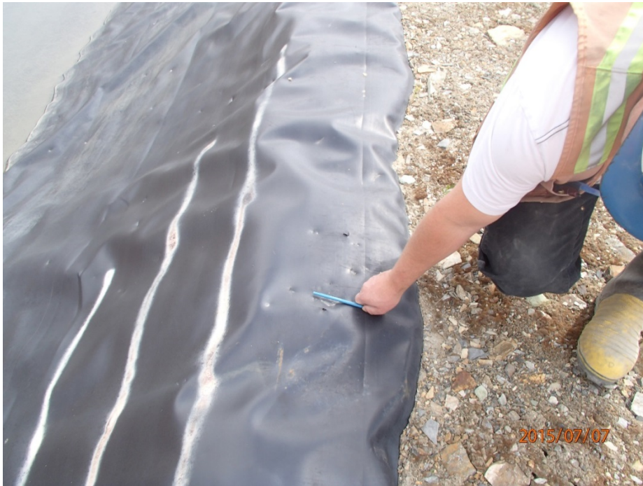
Photo 14 Sump 5 – puncture in the liner
