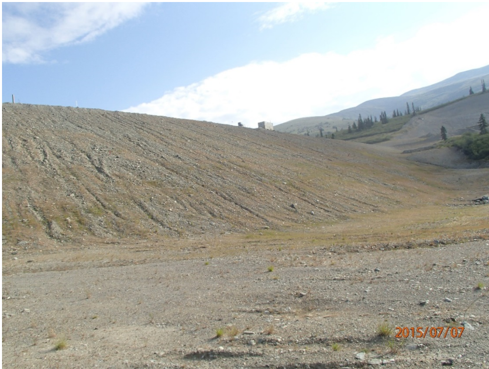
Photo 3 South dam –downstream slope looking east, erosion gully, minor grass grown naturally
