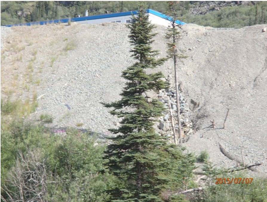
Photo 36 Camp pad – erosion channel in cut slope in south wall, partially backfilled with rock (east end), this channel was backfilled with rock to work as a French drain for surface runoff after large storm event
