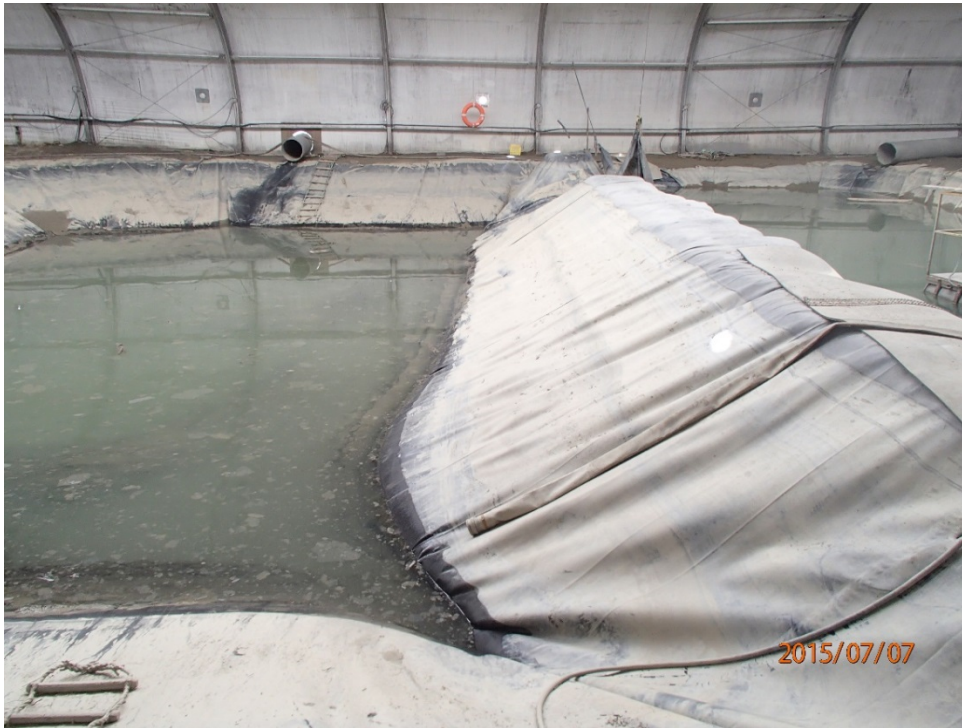
Photo 12 Sump 2 – bulge in the liner in the cross dyke, caused by groundwater
