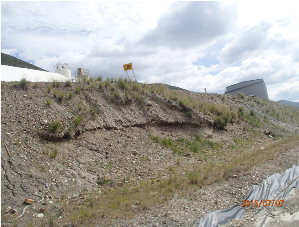
Photo 28 Ditch 4 – area of undercutting in the upslope noted in 2014 report was repaired (downslope of shotcrete and cement plant)
