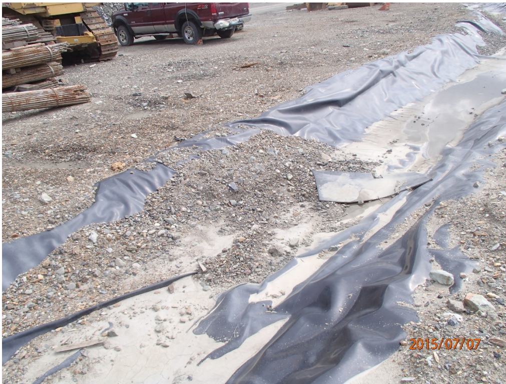
Photo 26 Ditch 4 – ditch bottom silted and filled with washed rock, reduced flow capacity
