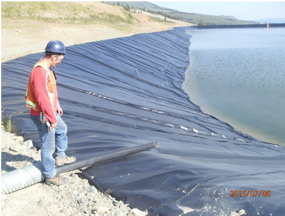
Photo 34 4 inch line discharging underdrain flow from waste rock storage area
