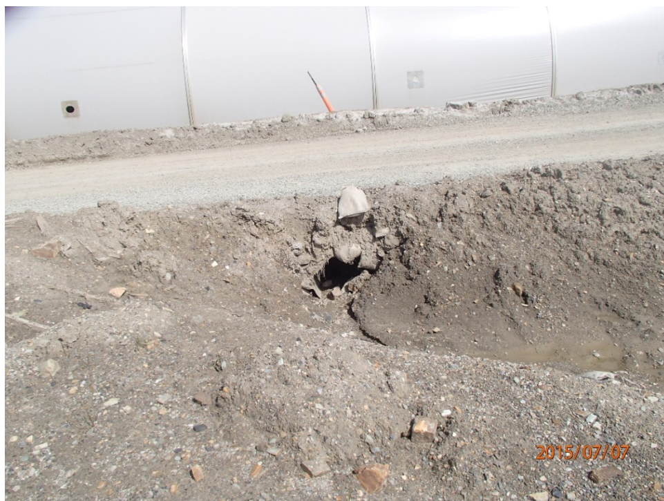
Photo 24 Culvert inlet to Sump 2- damaged and blocked
