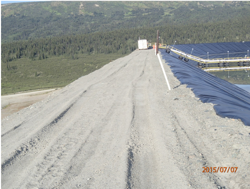
Photo 1 South dam crest - looking west; ruts on the crest surface
