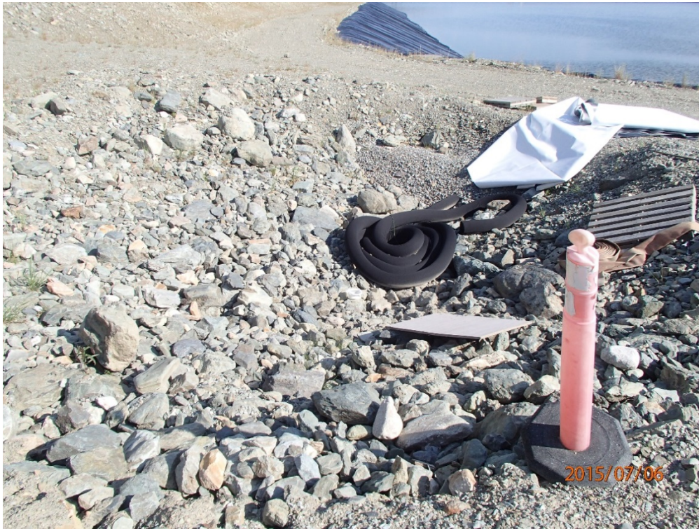
Photo 18 Underdrain intake basin – north end of the TSF
