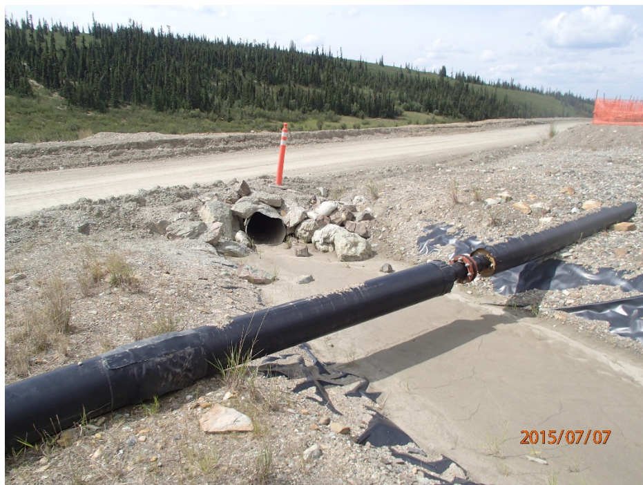
Photo 21 Ditch 3 – culvert inlet at the end of Ditch 2, channel bottom of Ditch 2 filled with silt, reduced flow capacity
