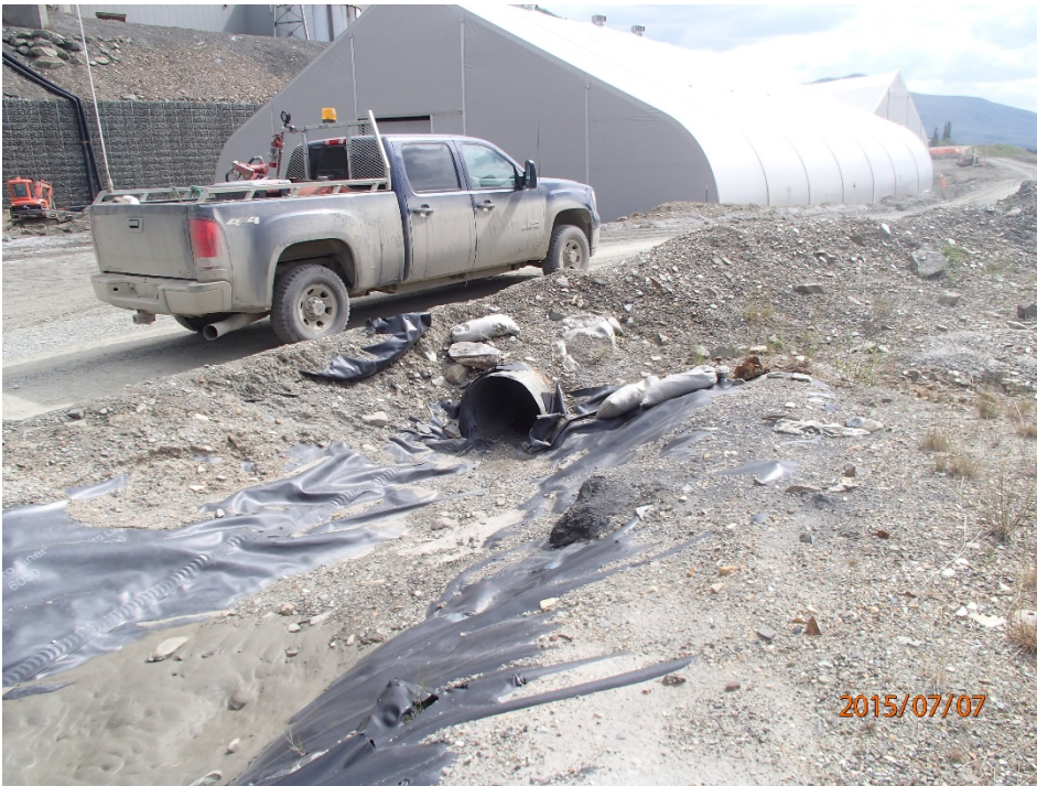
Photo 29 Ditch 4 – inlet for culvert, channel bottom and culver invert filled with sand, silt and gravel
