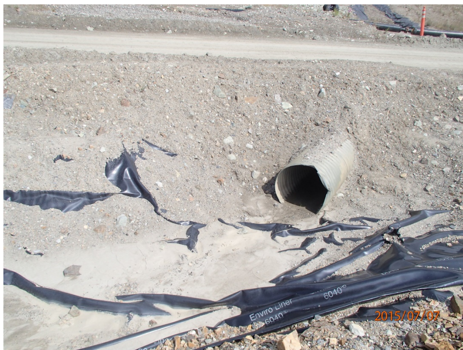
Photo 22 Ditch 3 – culvert outlet; channel bottom filled in and liner loose
