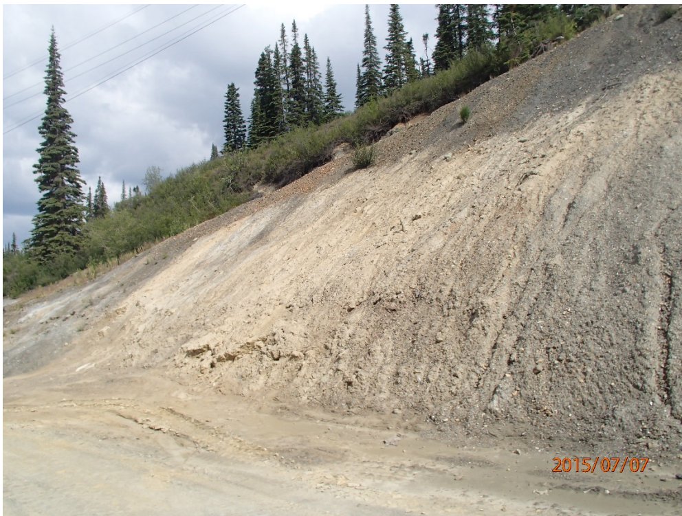
Photo 49 Truck shop pad – back slope, signs of sloughing
