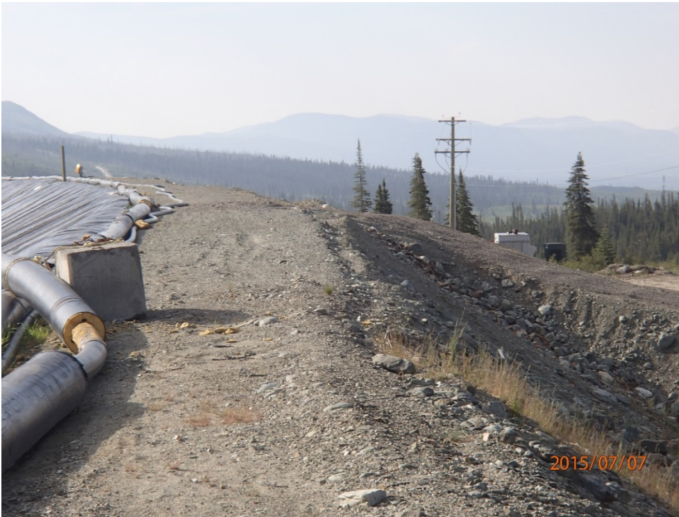
Photo 8 West dam crest - looking south, south of access ramp, less erosion and no crest loss
