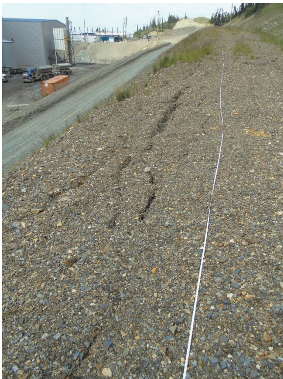
Photo 15 Ditch 1 – 26 m long crack in the Ditch 1 embankment, looking north from corner of Mill building
