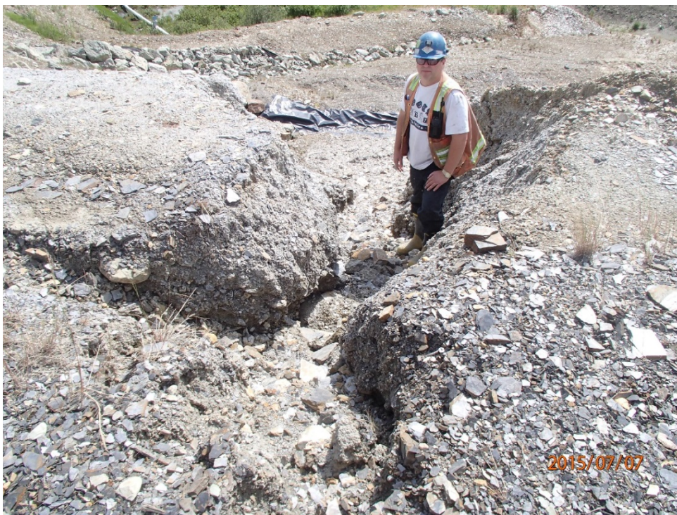
Photo 3 Mill building pad – downslope at southeast corner, large erosion gully from previous year, not repaired
