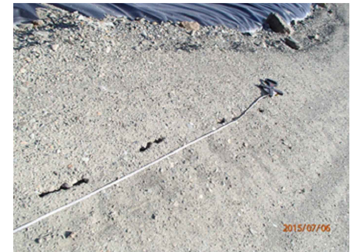
2015: TENSION CRACK UPSTREAM OF SLUMP APPEARED TO BE FILLED IN
