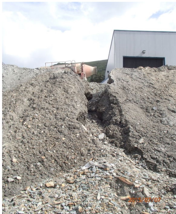
Photo 51 Truck shop pad – downslope, erosion channel near the west corner of truck shop building
