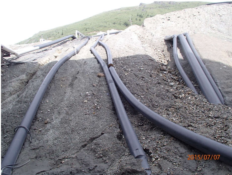
Photo 52: Crusher Building - sloughing and erosion around the pipe line corridor in the back slope
