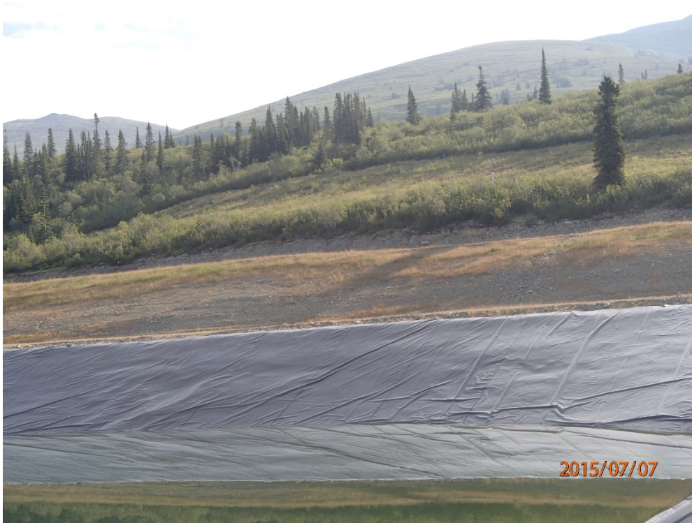
Photo 14 TSF east side liner– from west berm, minor bulging
