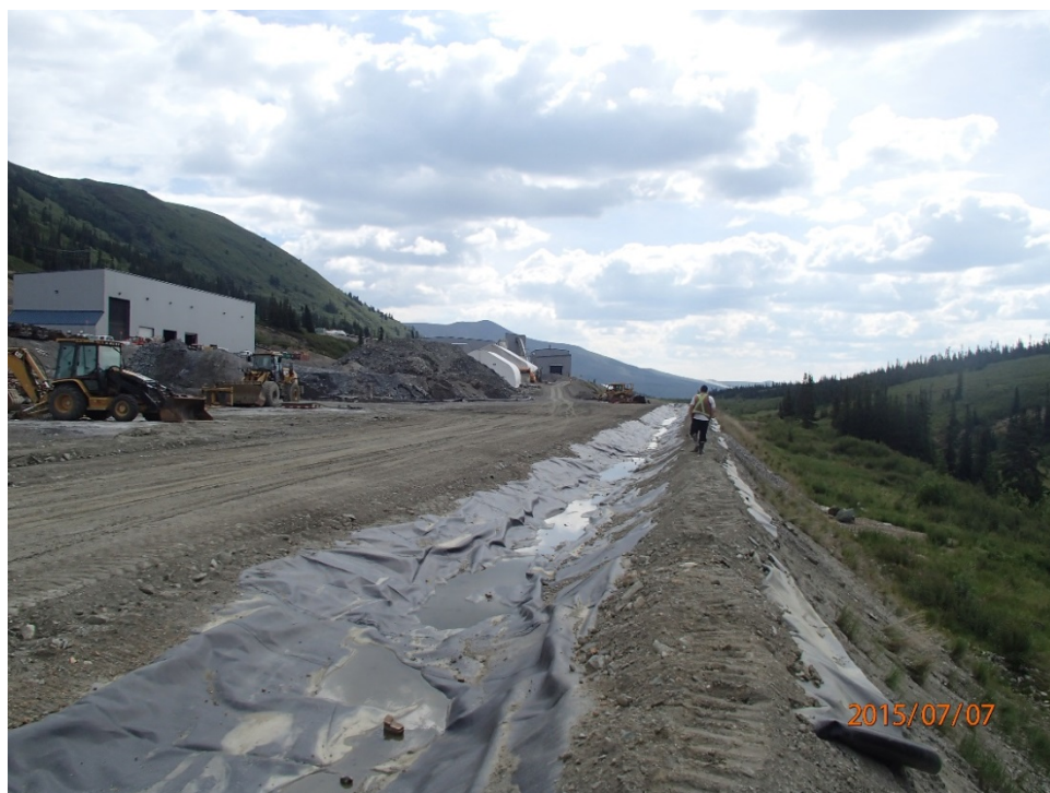
Photo 25 Ditch 4 – lined channel looking east, liner along the downstream side loosely anchored by uncompacted fill, may wash away after large rainfall event (2015 construction)
