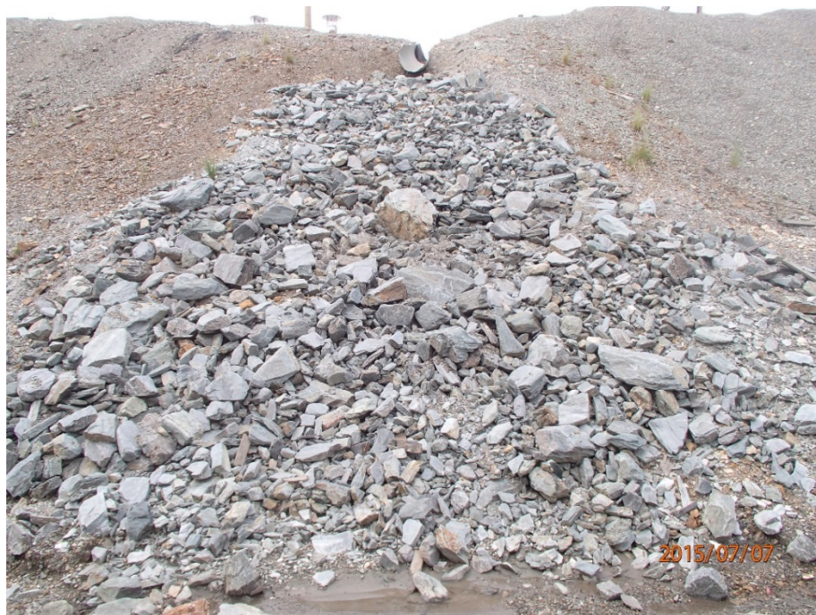
Photo 8 Fuel Tank Farm and Genset Pad –downslope at east side, half culvert with rockfill slope, good condition
