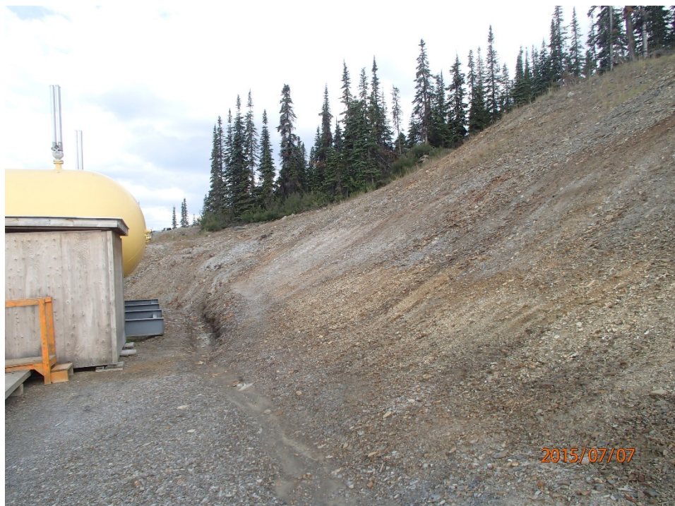
Photo 47 Propane Tank Pad – back slope, surface water cutting a small channel at the toe
