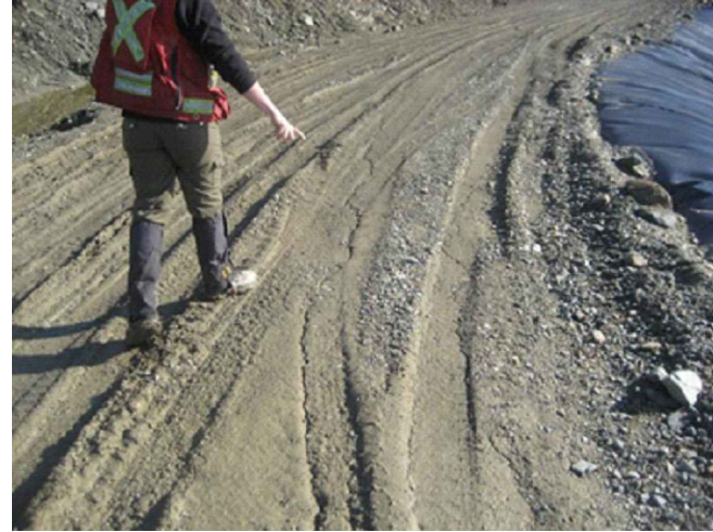
2014: CRACKS AT NORTH END OF IMPOUNDMENT
