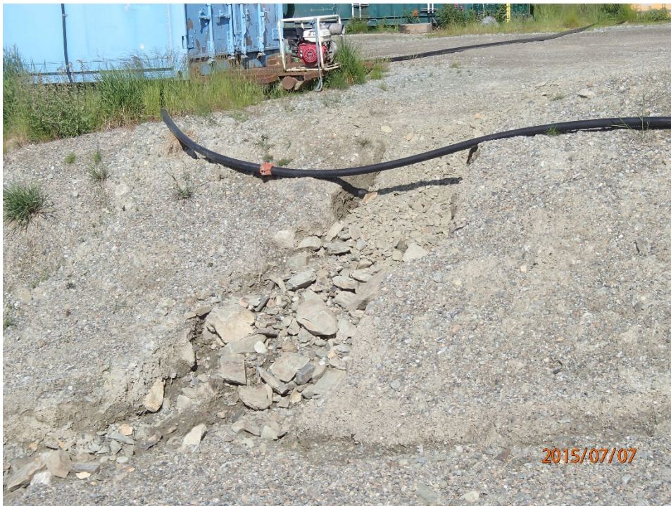
Photo 40 Sewage Treatment Plant Pad – erosion channel in the down slope south east corner
