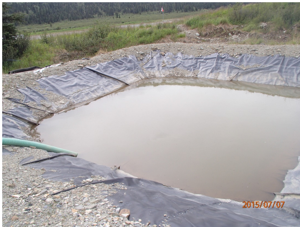
Photo 46 Land Treatment Facility – sump
