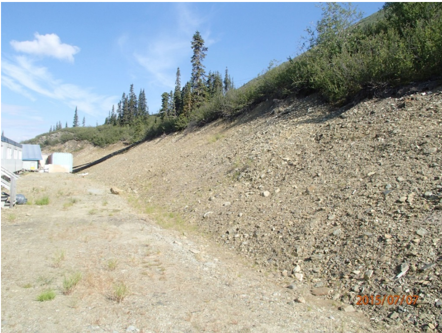
Photo 37 Upper generator and potable water treatment pad – cut slope looking west, minor erosion gullies
