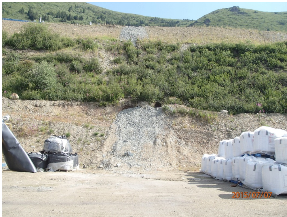
Photo 34 Camp pad – erosion channel in cut slope in south wall, partially backfilled with rock (centre part)
