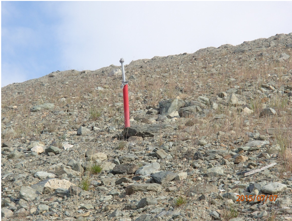
Photo 42 Non-functional Inclinometer on the downstream slope
