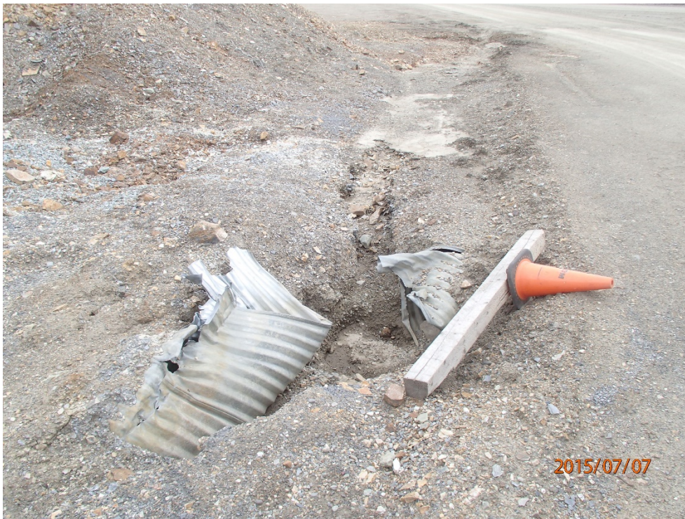
Photo 18 Ditch 1 – culvert damaged
