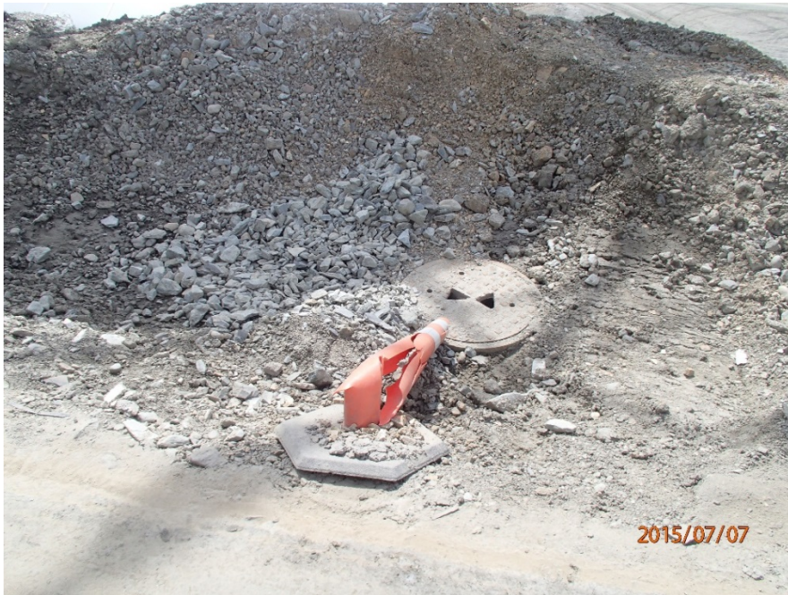
Photo 6 Manhole upslope of MSE wall corner of Mill building and Concentrate building, this manhole is outlet for culvert from Ditch 5, a large sinkhole developed around this manhole after a recent rain storm, backfilled with rock fill
