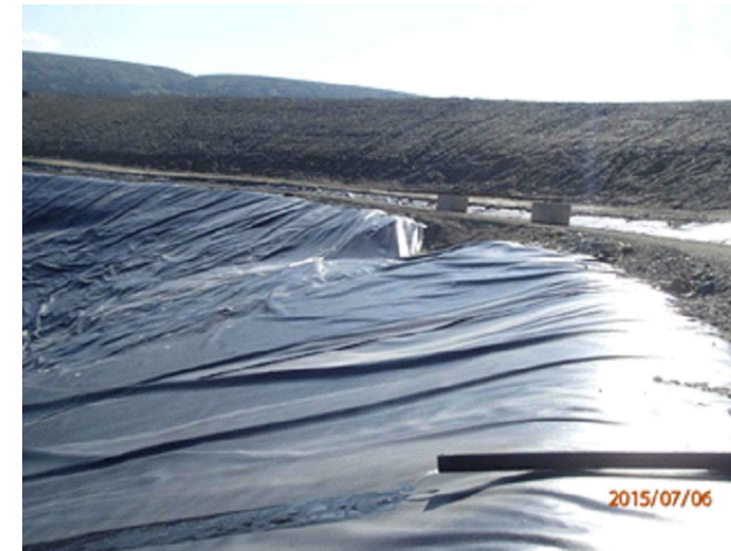
2015: ANCHOR FAILED IN 2014 CRACK AND SLUMP AREA
