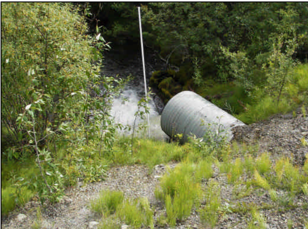
Photo 4: Perched culvert at the Robert Campbell Highway on Light Creek 1, August 6, 2005.
