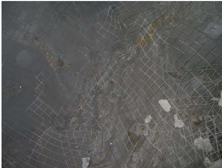
Photograph 32 View of the back at the intersection of herringbone panels and decline - Note ground support consisting of split sets, screen, and shotcrete
