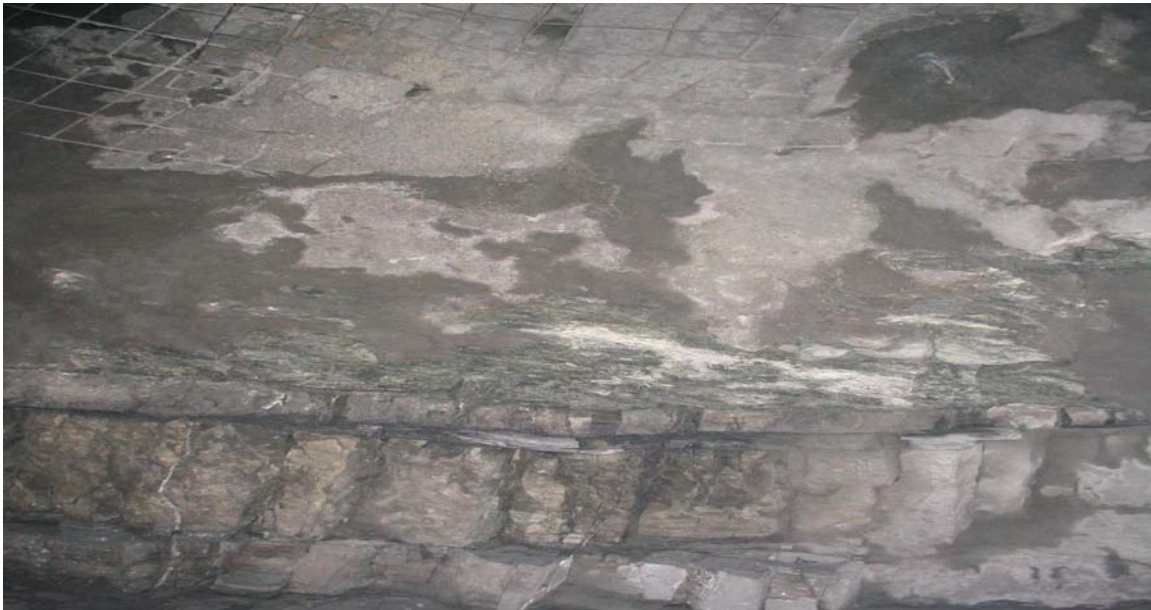
Photograph 18: Location 6 View of the upper part of wall in massive sulphide and argillite contact and argillite in the back
