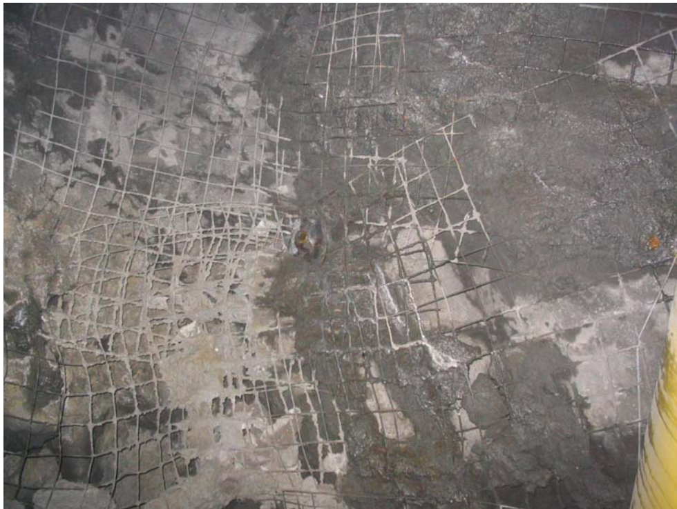
Photograph 20: Location 6 View of the Shotcreted back with screen and split set ground support
