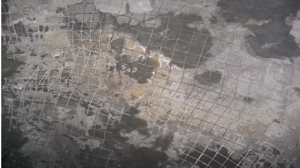
Photograph 19: Location 6 View of the Shotcreted back with split set and screen ground support
