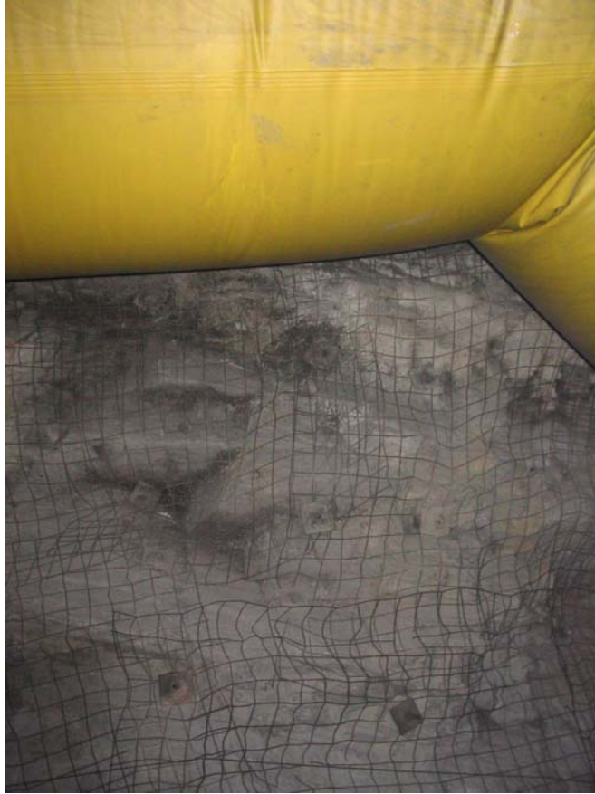
Photograph 7: Location 2 View of the back in EXCP. Note screen, split sets and a resin rebar
