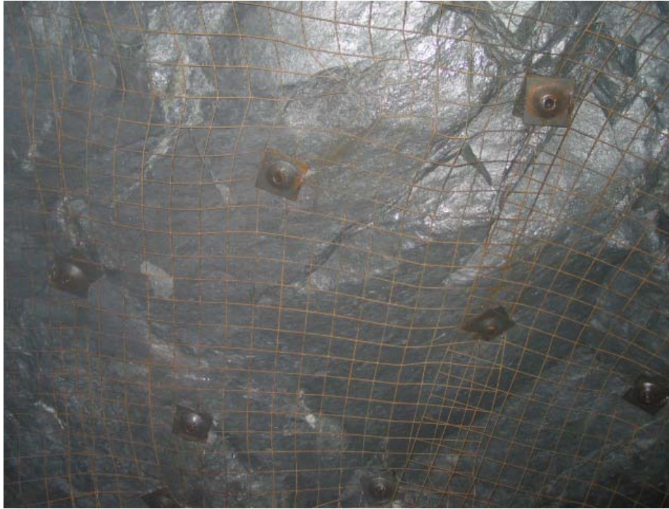
Photograph 29: Location 8 View of the back in the ore zone – Note the split sets and screen ground support
