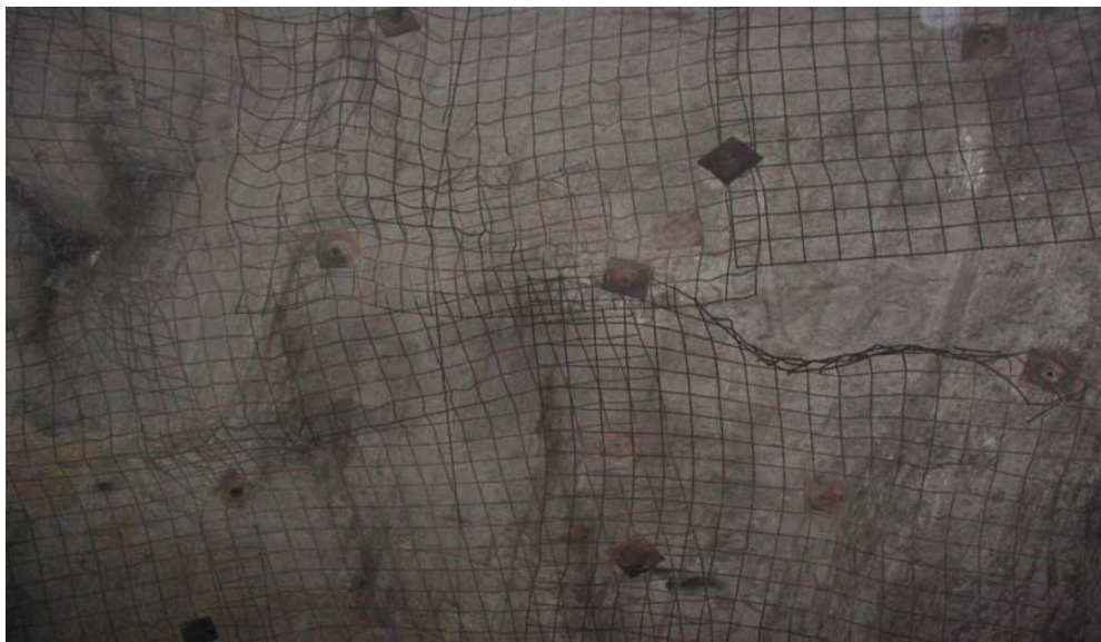
Photograph 6: Location 2 View of the back in EXCP. Note screen and split sets ground support
