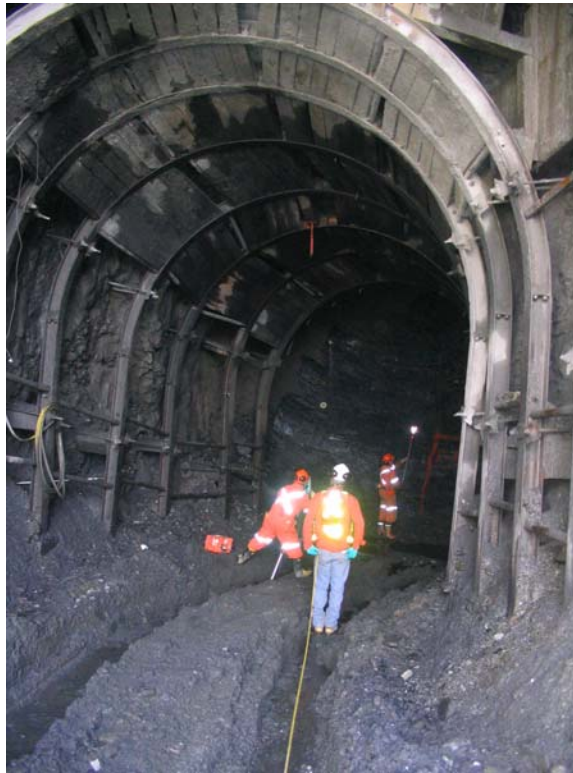
Photograph 4: Location 1 View of Arch steel set support at the portal - Note very poor rock quality of the FW
