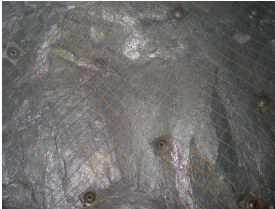
Photograph 28: Location 8 View of the back in the ore zone – Note the split sets and screen ground support
