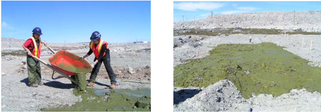
Figure 2.5. a) Sludge from the North Inlet Water Treatment Facility being applied to the 25/75 substrate, b) Sludge after being applied to the substrate at the reclamation site at Diavik Diamond Mine, NWT.
