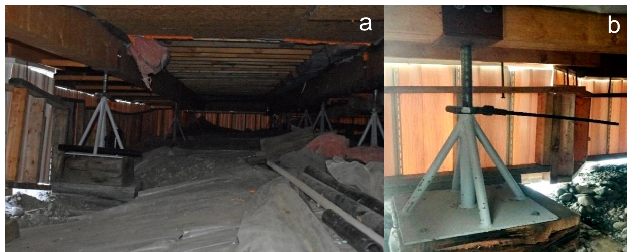
Figure 5.5 (a) Foundation jack located under the house, where (b) a wrench is used to raise or lower the support beams.
