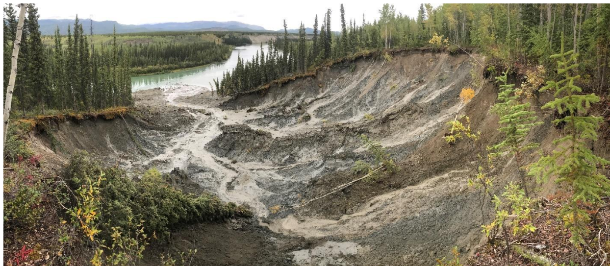
Figure 7.2 Panoramic view of thaw slump bowl on 24 August 2020, looking northeast. The headscarp retreats as mudflows transport thawed material into Takhini River.
