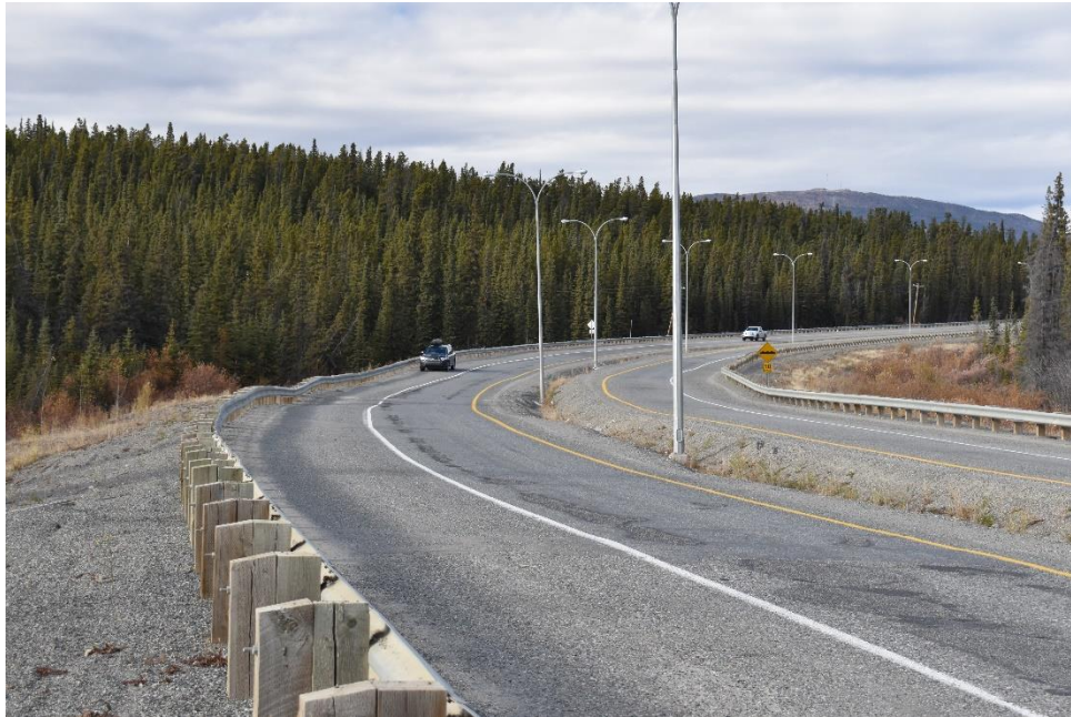
Figure 4.5 Example of differential road settlement (4 October 2018).
