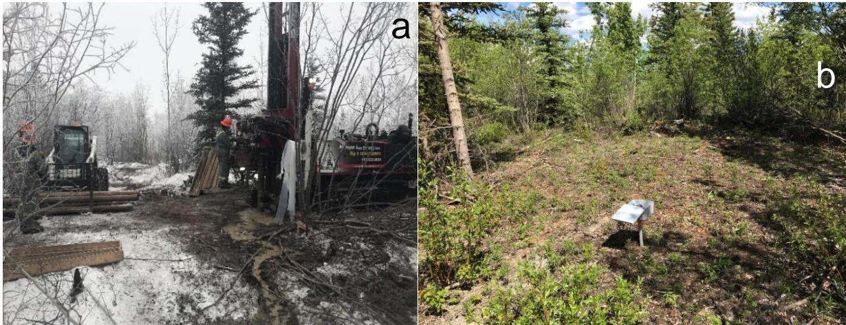
Figure 6.4 Midnight Sun Drilling Sonic drill rig (a) and instrumented borehole (b) at IV_BH1.
