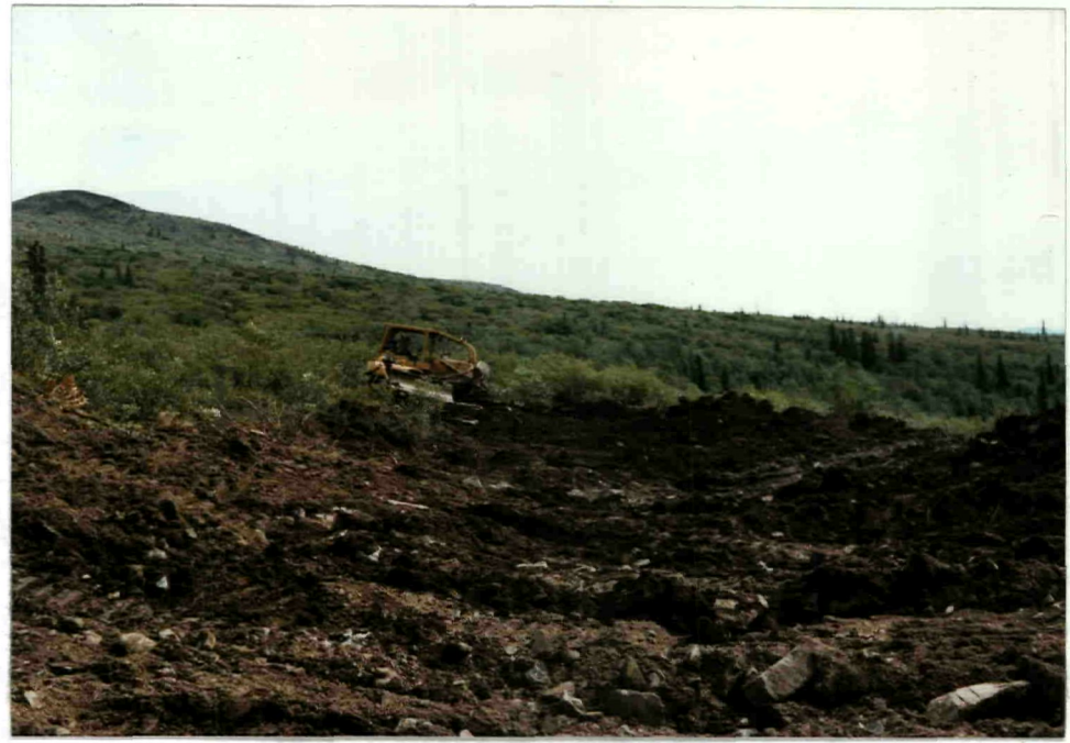
Bulldozers stripping prior to backhoe trenching (removal of vegetation facilitates thawing of permafrost).
