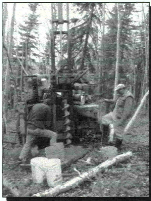
Drilling along a line on the rim of the high bench at the 1650 ft. contour.
