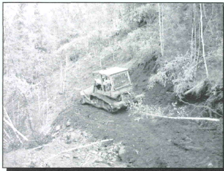
Photo 5 - Building road along the south facing slope of the Marten Creek valley.
