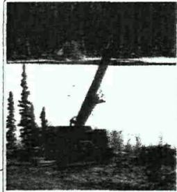
Drilling on the Can Alaska property near the White River by Anchor, Cathro and Assoc ('81) Ltd during their 1995 exploration program. A 1973 drill hole intersected 3m of 1.8 gpt Pt+Pd, 0.94% Ni and 0.33% Cu.
