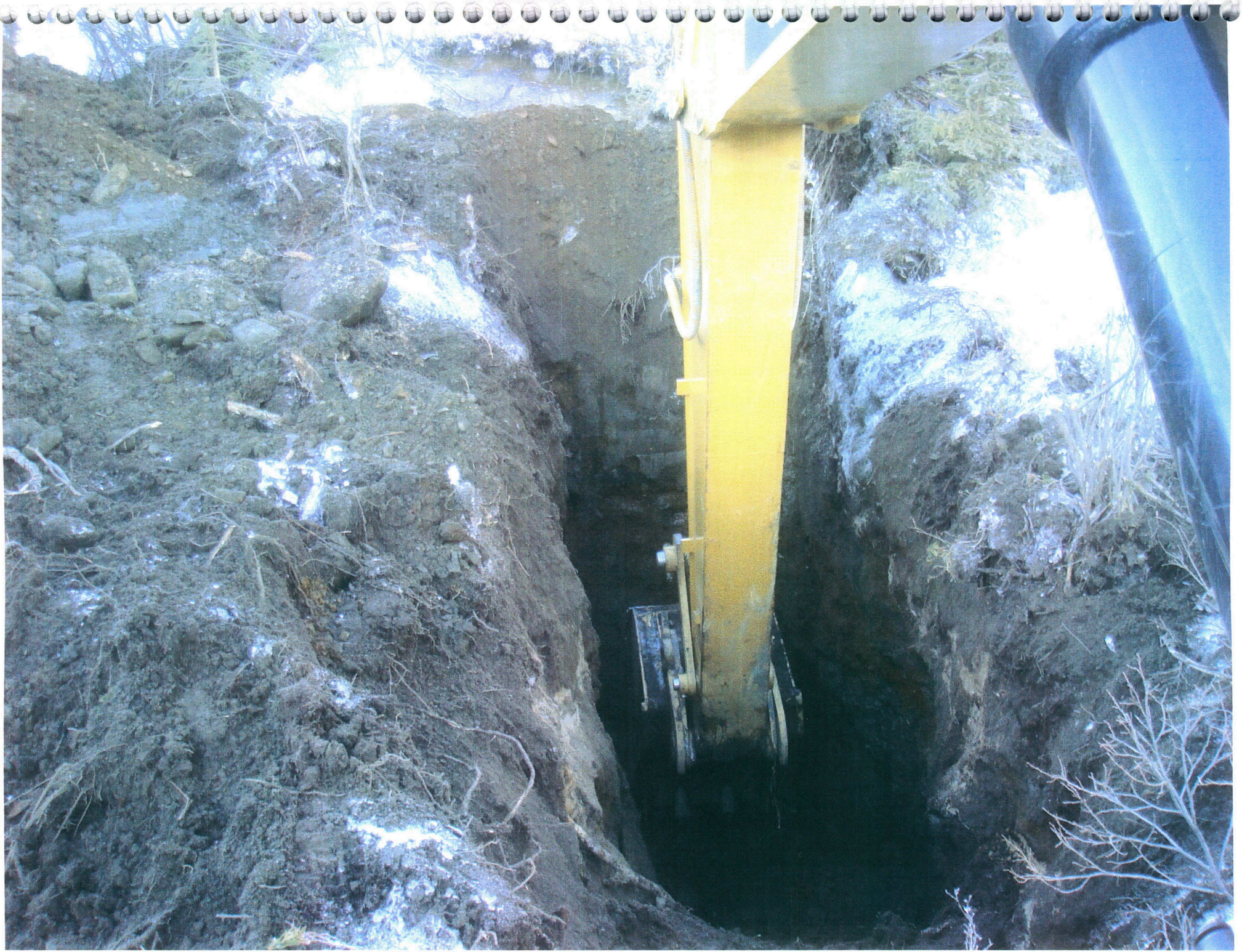
Test Pit to check for accuracy of the layer depths that the resistivity lines indicated.
