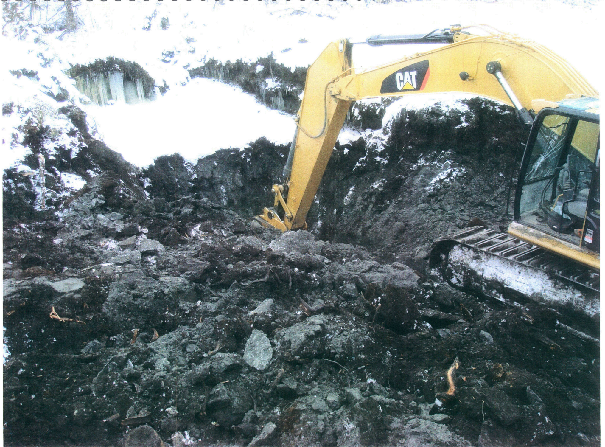
Test Pit to check for accuracy of the laser depths that the resistivity lines indicated.
