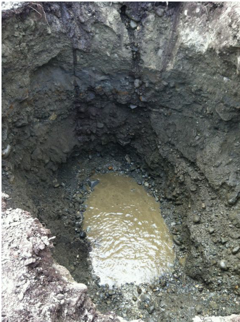
Groundwater entering pit 2
