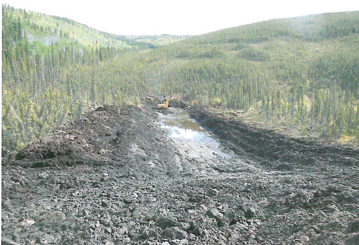
Plate 6 - A view looking south along the bulldozer trench excavated by the D10N. The Caterpillar 225 excavator can be seen at the south end of the trench.
