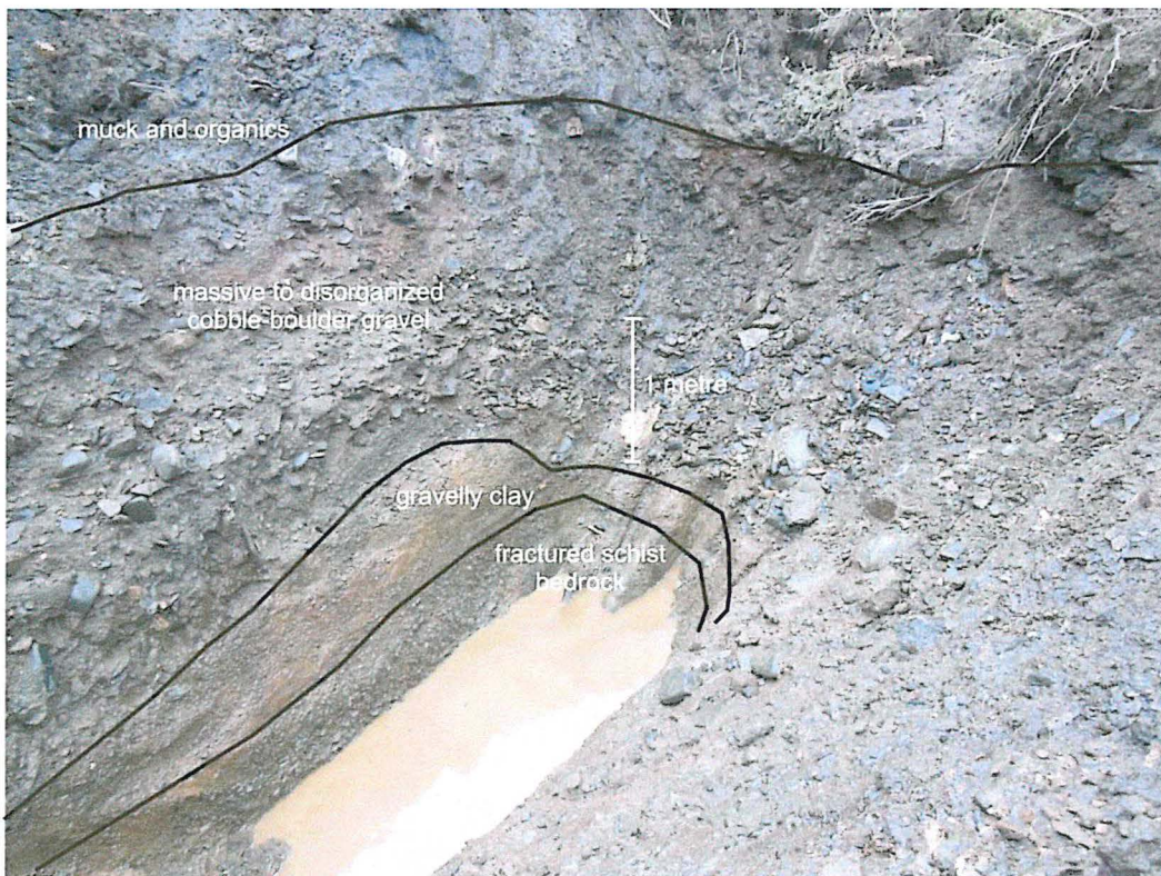
Plate 7 - Excavator test-pit CAN14-01, showing the stratigraphy down to bedrock. View looking south-southwest.
