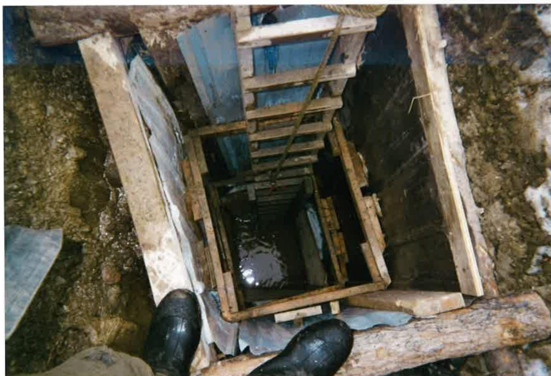
THAWED WET AT BOTTOM CC-4 MARCH 27, 2015
