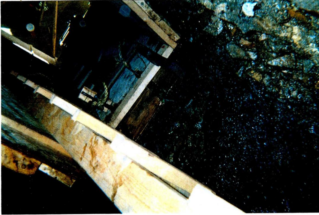
SHAFT CC-3 LOOKING UP TO TIMBER ON JULY 7, 2014 TIMBERED TO 14 FT. 9 in.
