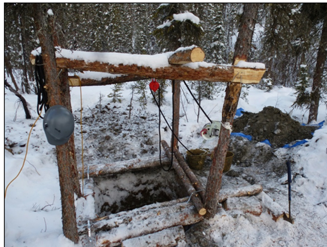
Figure 16. The shaft setup manual windlass (pulley bucket system) with the first gravel stockpiled to right
