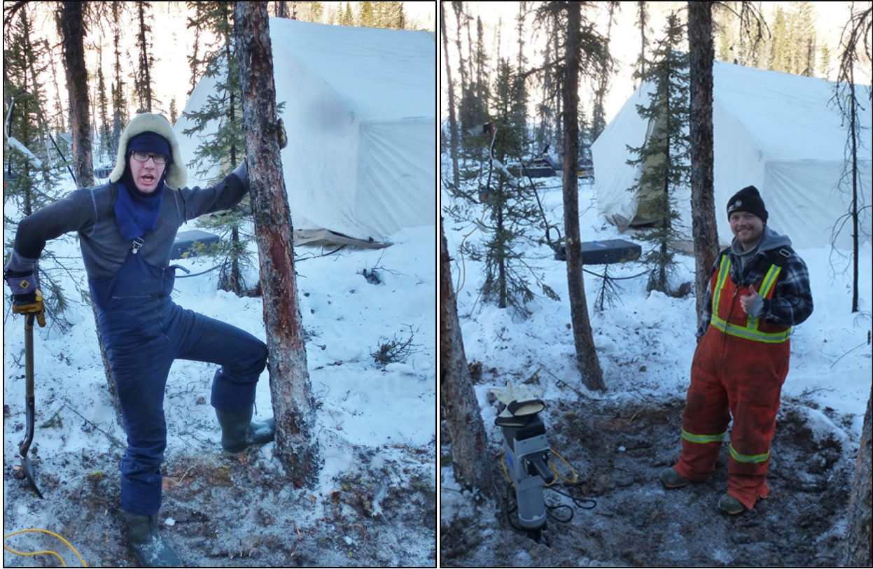
Figure 15 Clayton Jones (left) and Milo Mielniczuk (right) breaking ground for the shaft
