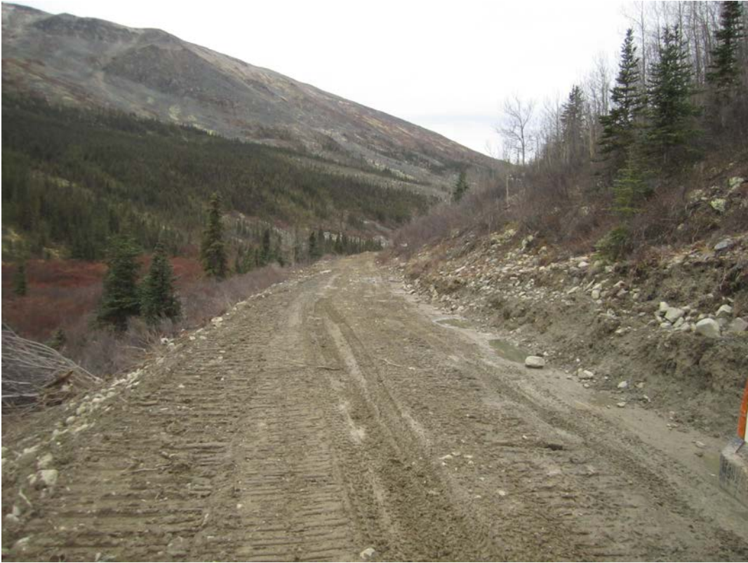
Figure 25: Upper Lightning Road upgrading on claims. Derocking, brushing and grading to accommodate trucks. img 8069
