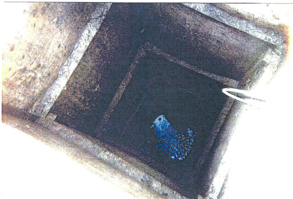
SHAFT CC-3 PUMPED OUT ON SEPT 23, 2014 NOTE: FOAM-WATER HAS INCREASED FROM DRIPPING TO FLOWING (RATE 4 FT. DEPTH/DAY) PUMPED OUT 22 FOOT LEVEL
