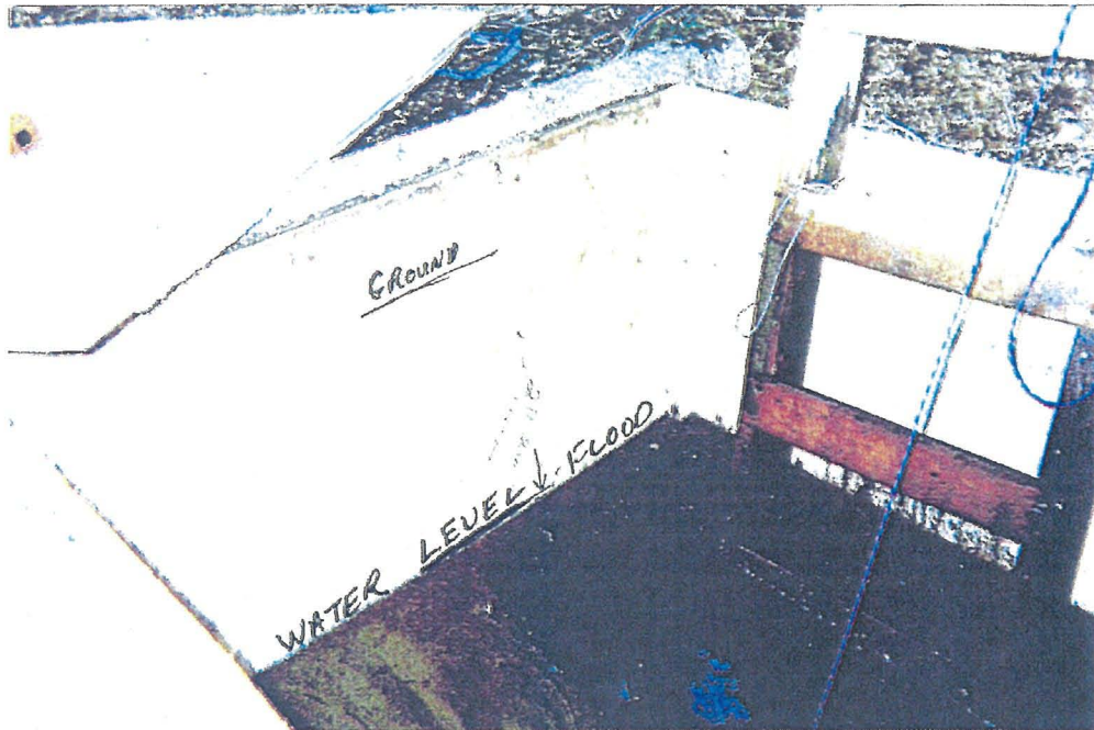
SHAFT CC-3 FLOODED
