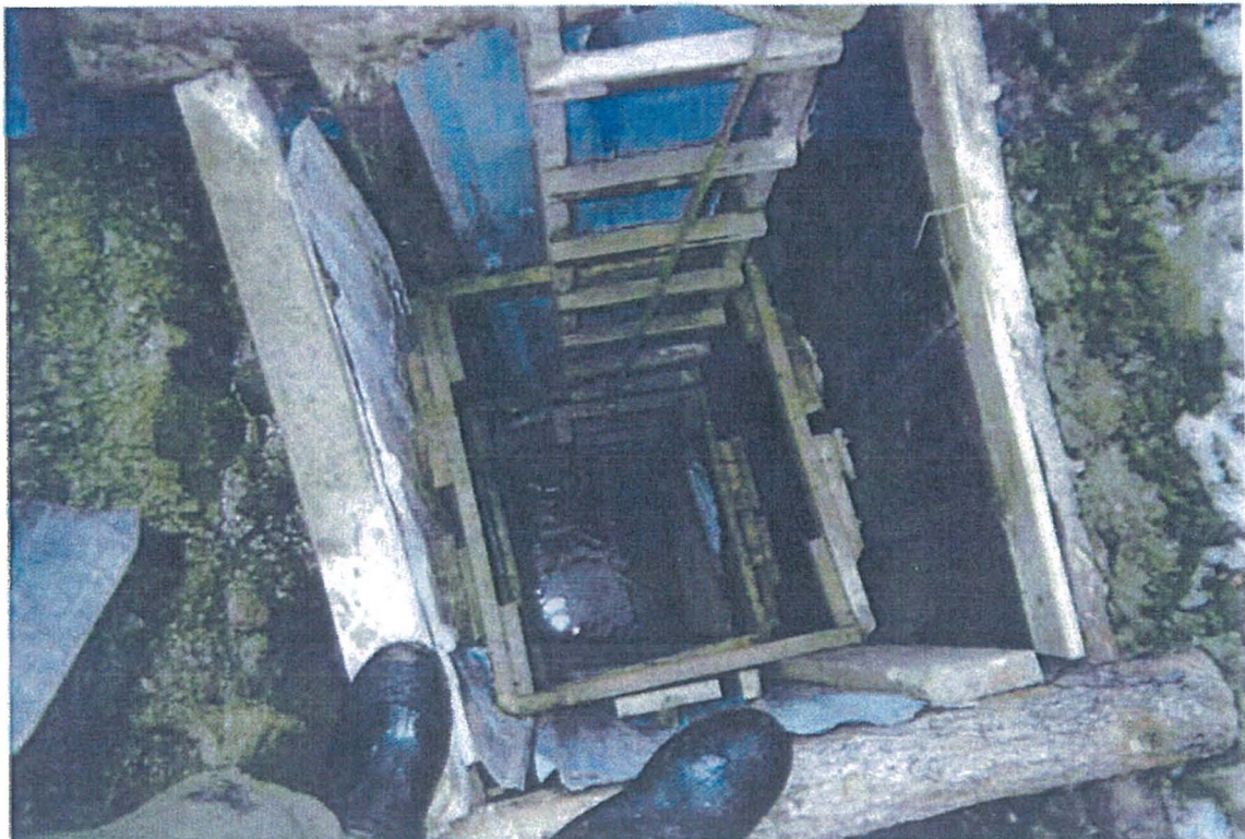
THAWED WET AT BOTTOM CC-4 (FLOODING) MARCH 27, 2015
