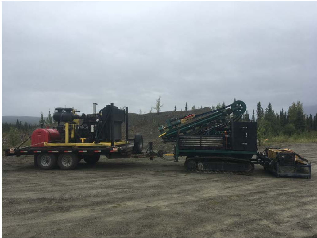
Figure 10: RC Drill with compressor in tow. Casing and other drilling equipment is carried in the steel basket chained to the blade.
